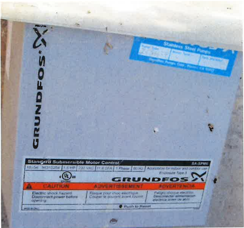
Figure 11 Pump & Motor Controller for Well Behind Barn
