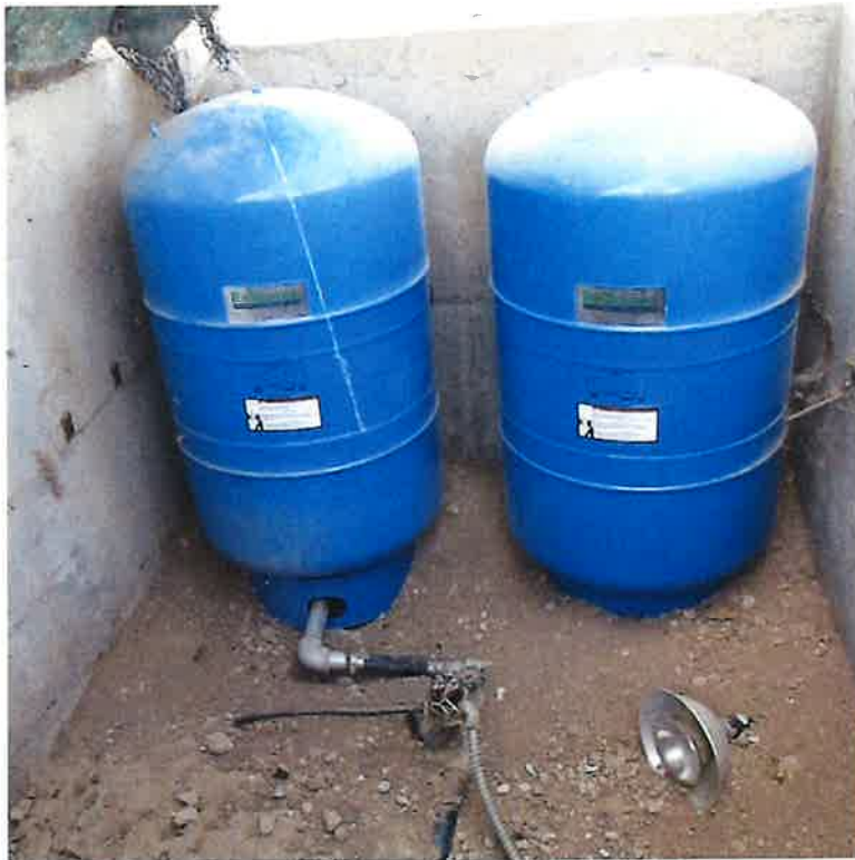
Figure 10 Pressure Tanks for Well Behind Barn
