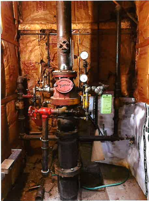
Controller inside main warehouse.
