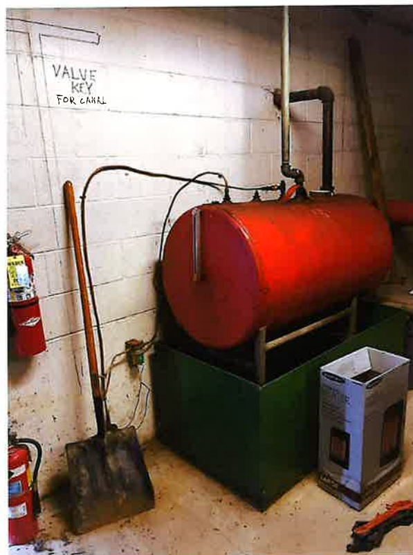
Diesel fuel tank.
