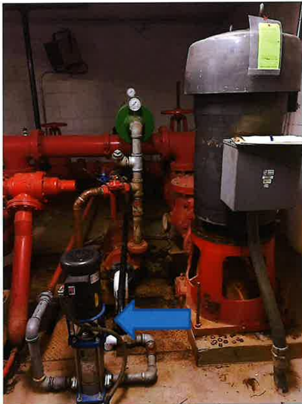
Jockey pump for primary pump on the right.
