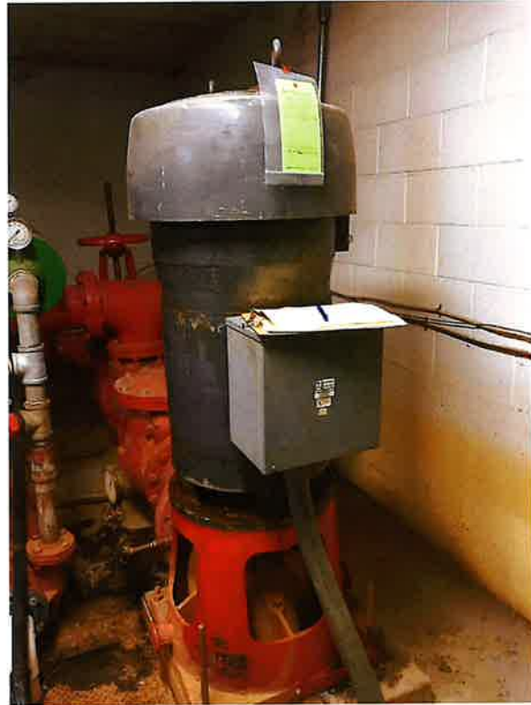
Primary fire protection pump in pump house.
