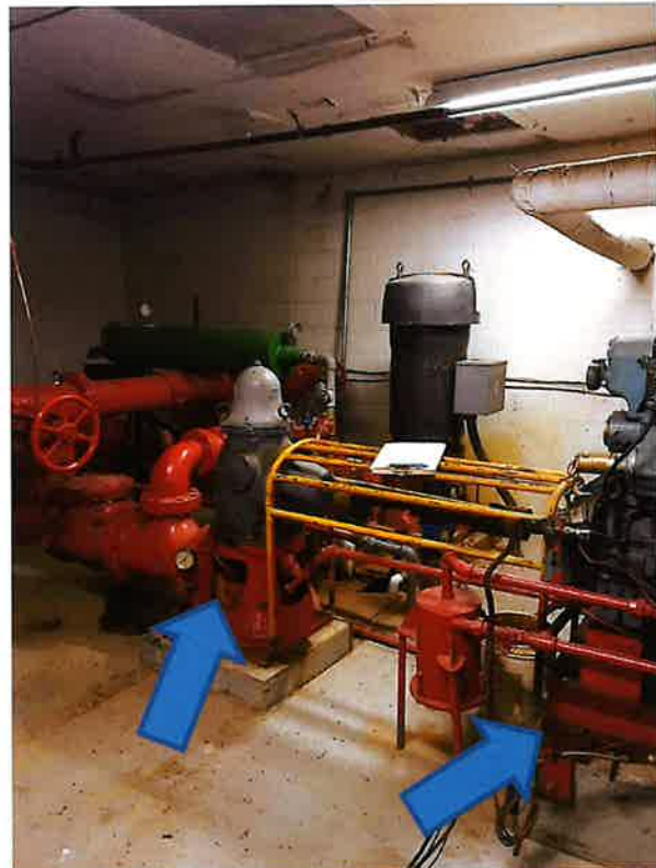
Diesel motor and pump for fire protection system.
