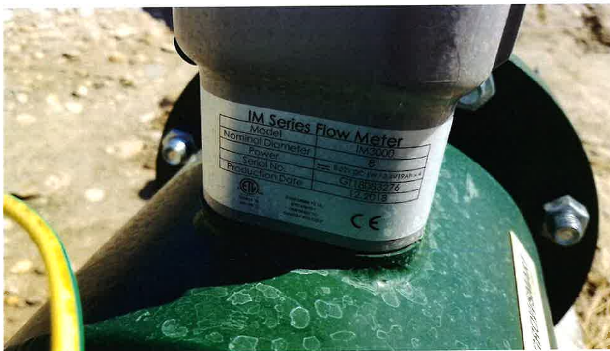
Figure 23: Flowmeter information for flowmeter in easterly flowing discharge piping from Well 2
