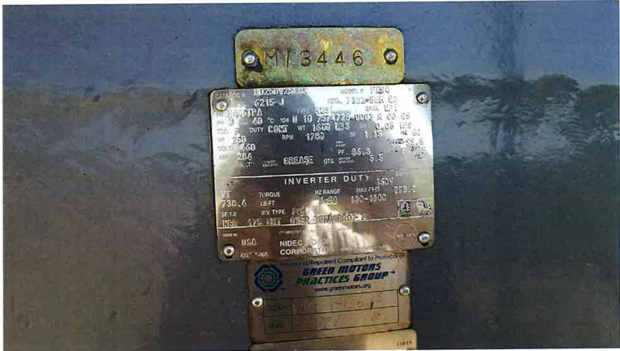
Figure 1: Well 1 (Hansen Well) - pump motor (40hp) information
