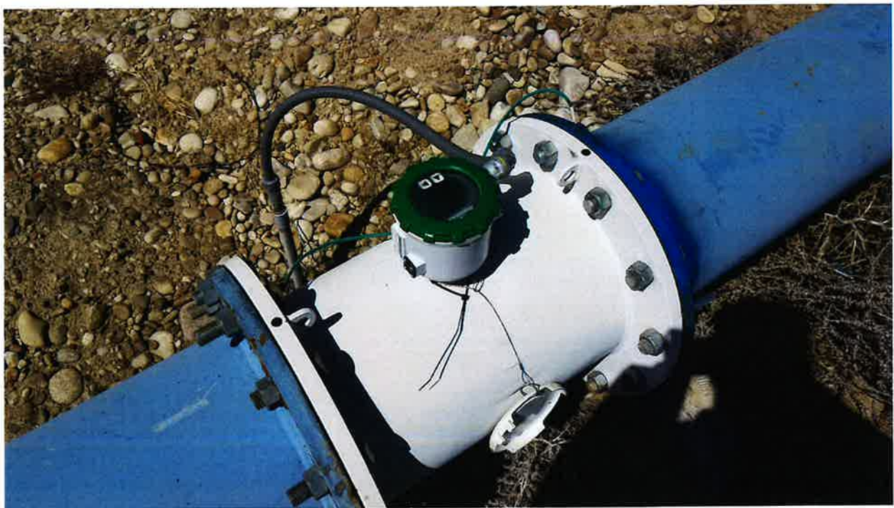
Figure 18: Well 2 primary flow meter
