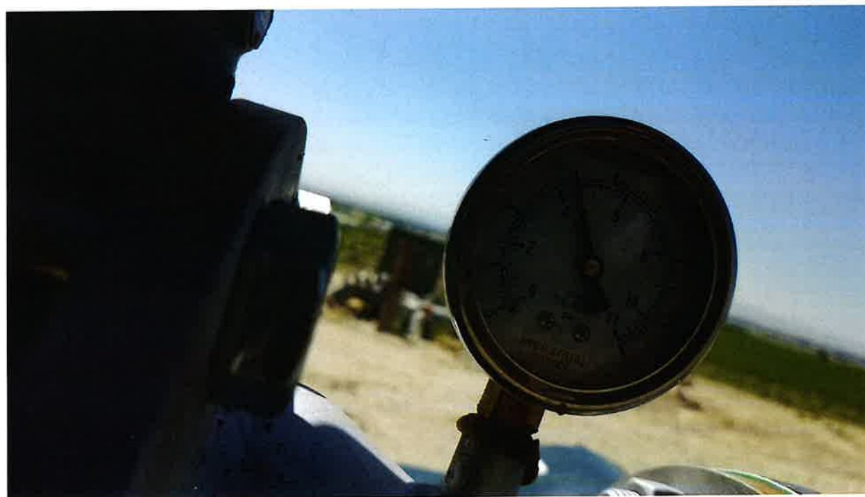
Figure 20: Well 2 pressure gage reading
