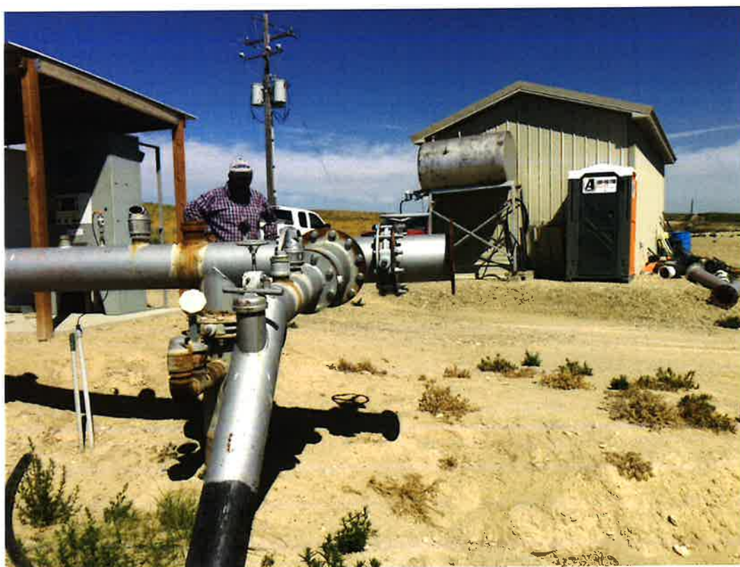
Figure 6: Well 1 discharge piping and flush (looking N)
