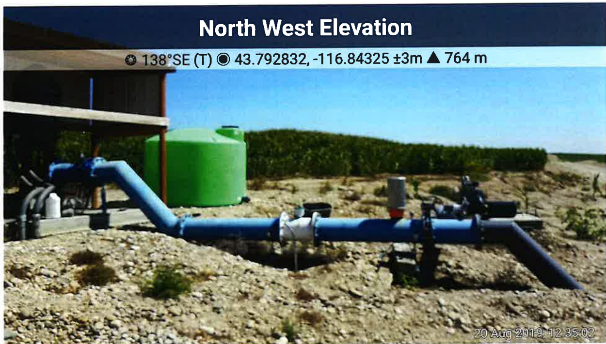
Figure 15: Well 2, pump, and discharge piping (looking E)
