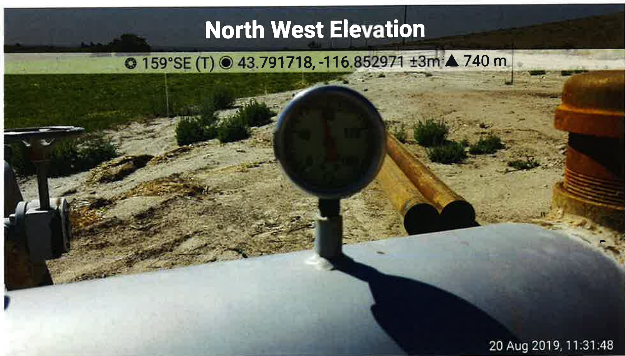
Figure 9: Well 1 pressure gage reading
