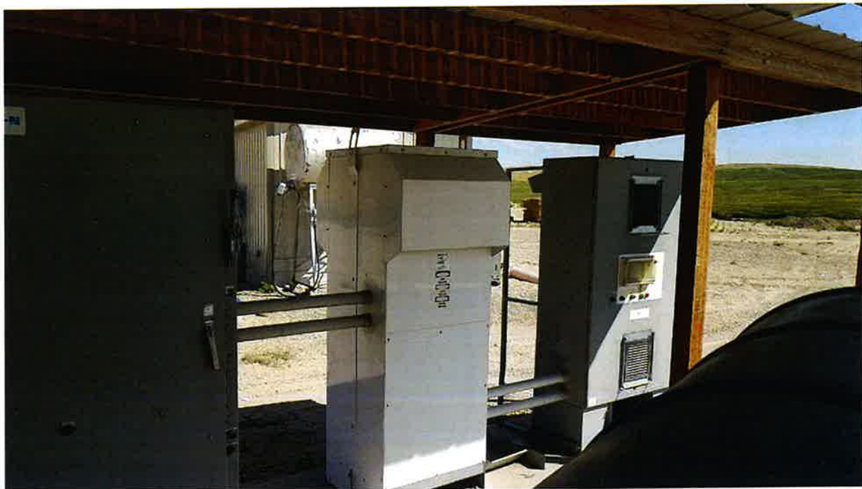
Figure 2: System control panels located next to Well 1 (vfd panel is on furthest right of photo)
