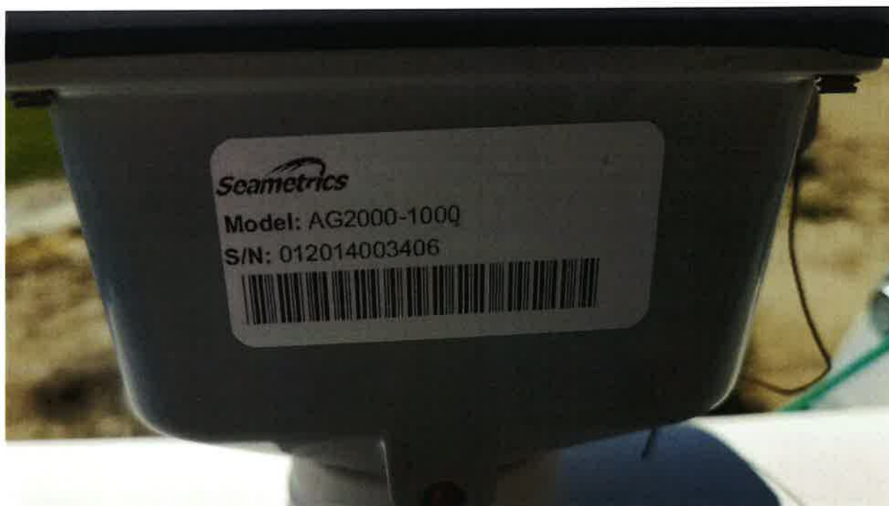
Figure 7: Well 1 flow meter information
