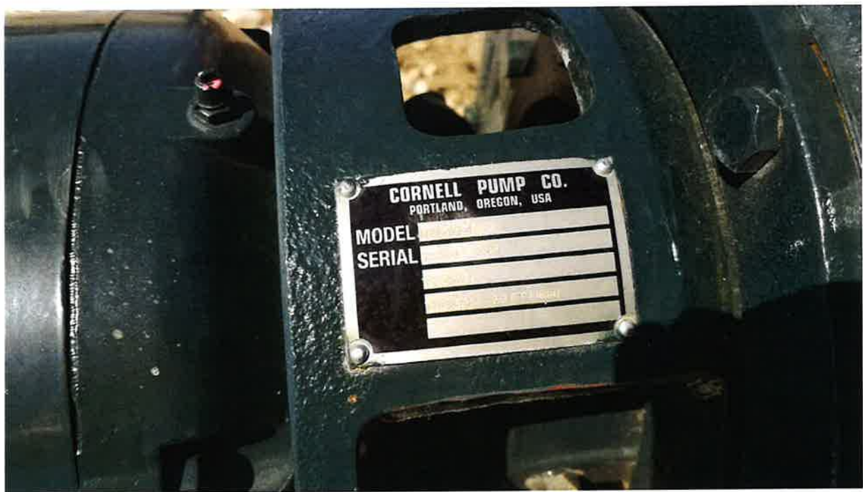
Figure 25: Booster pump information (from Well 2 easterly flowing discharge)
