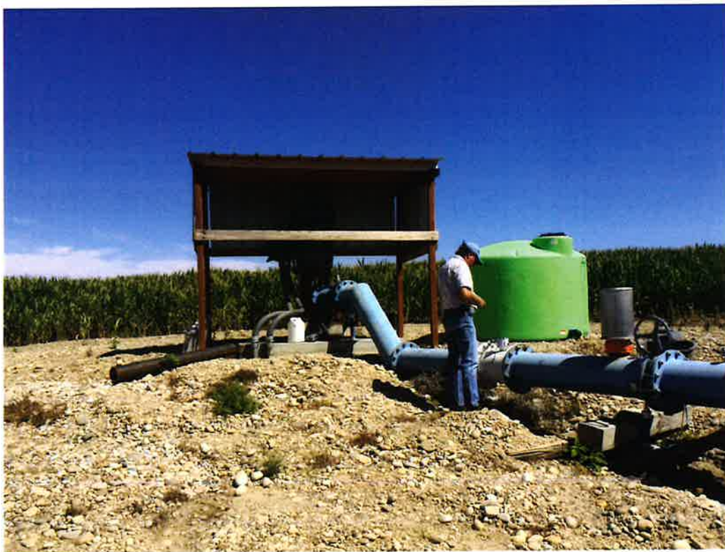
Figure 16: Well 2, pump, and discharge piping (looking N)
