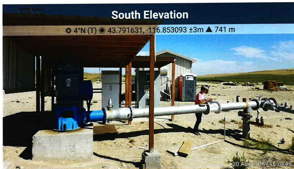
Figure 4: Well 1, pump, and discharge piping (looking N)
