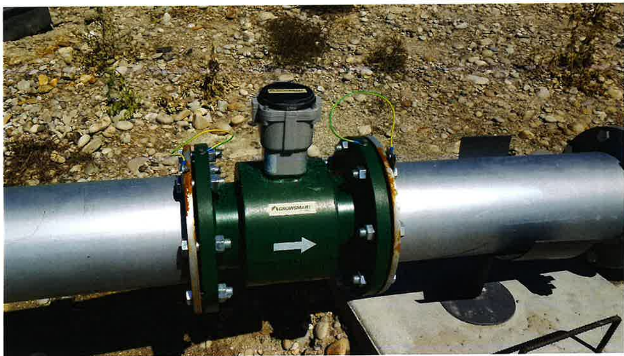
Figure 22: Flowmeter in easterly flowing discharge piping from Well 2
