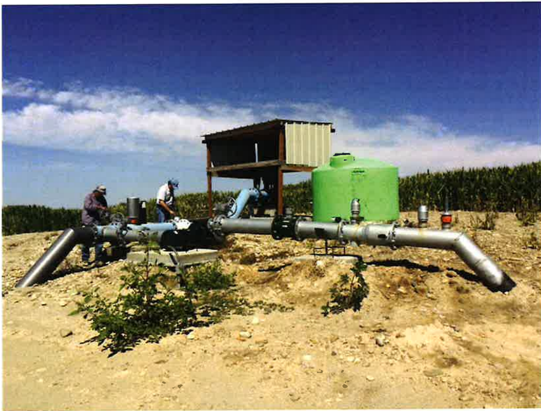
Figure 17: Well 2, pump, and discharge piping (looking NW)
