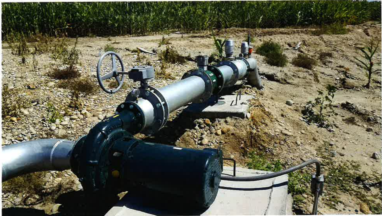
Figure 21: Discharge piping and booster pump (looking ENE)
