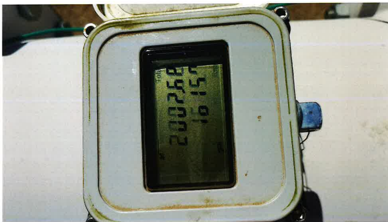
Figure 8: Well 1 flow meter reading near end of measurement period
