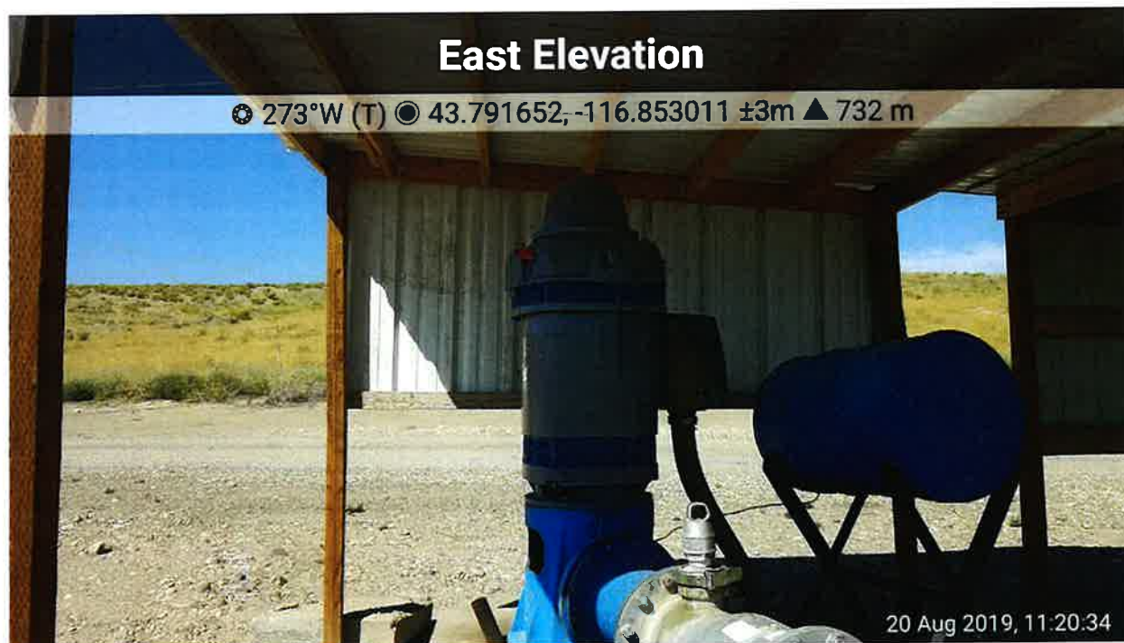
Figure 3: Well 1 & well pump (looking W)
