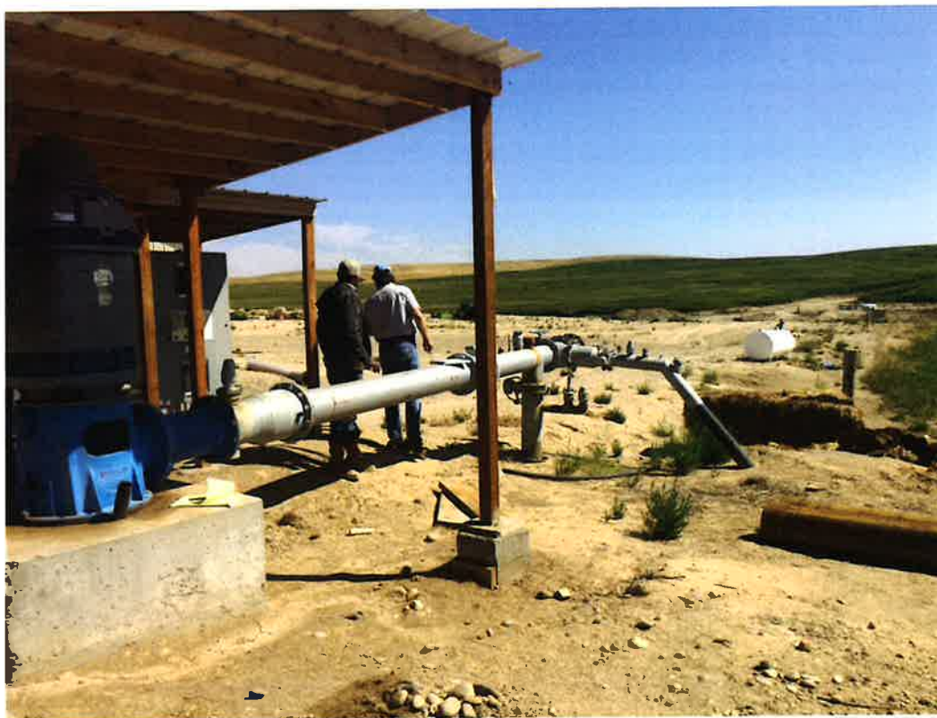
Figure 5: Well 1, pump, and discharge (looking NE)
