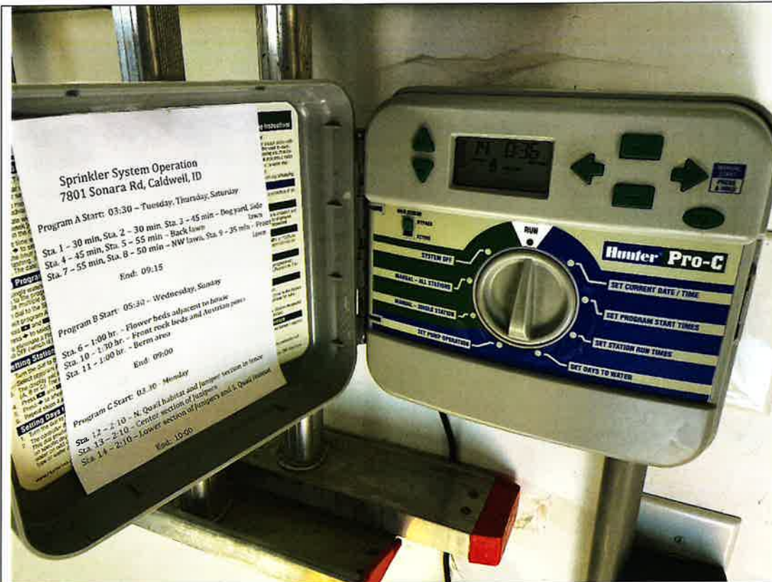
Sprinkler Control Box
