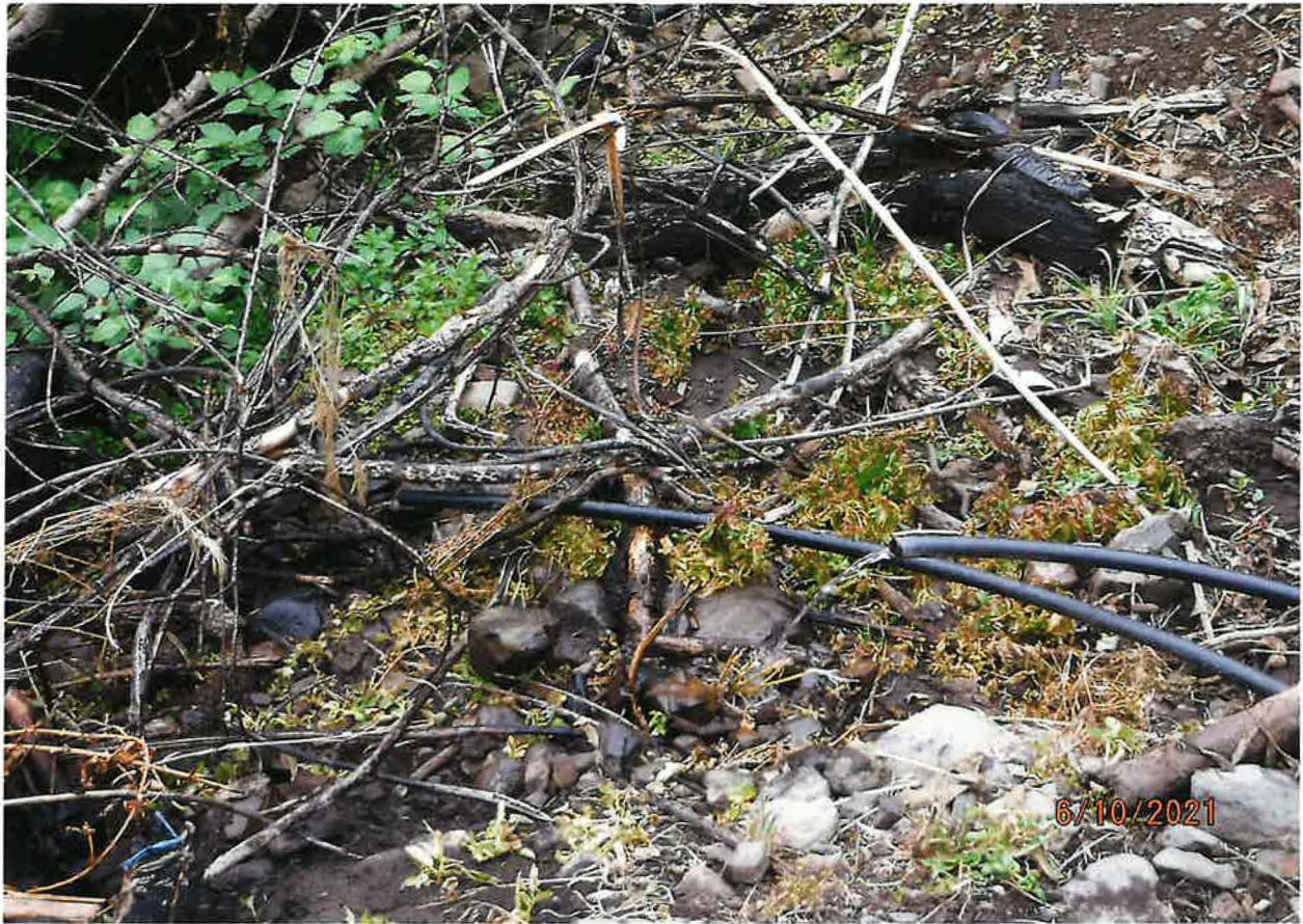
2EA OVERFLOW PIPES FROM 2EA SETTLING TANKS RETURN FLOW TO STREAM CHANNEL
