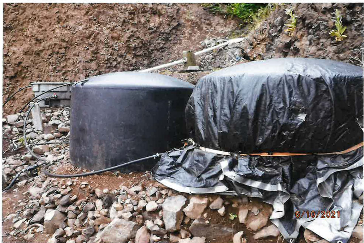
1EA 500 GAL & 1EA 450 GAL 24HR IMPOUNDMENT TANKS
