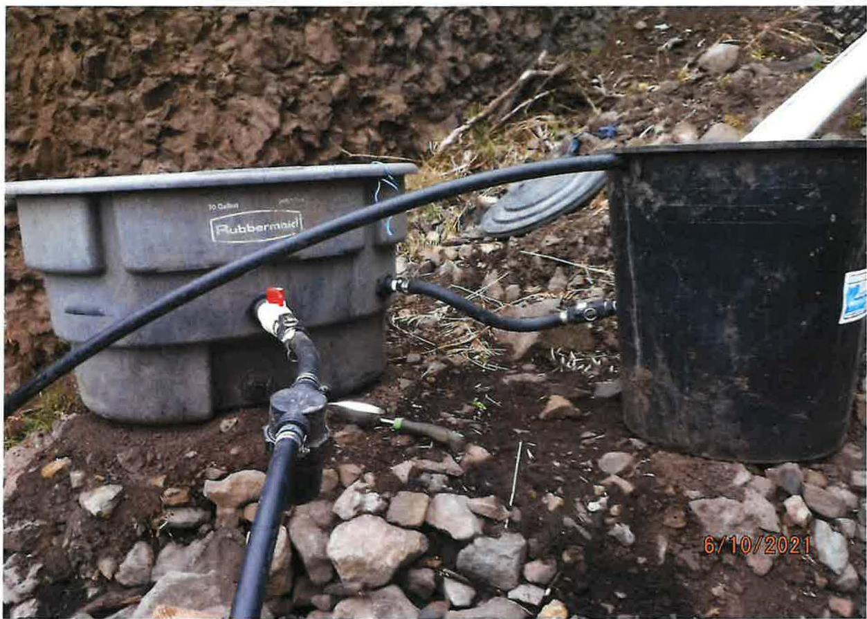
AT POD – 2 OPEN AIR SETTLING TANKS THAT ROUTE TO 2 CLOSED TANK 24HR IMPOUNDMENT TANKS
