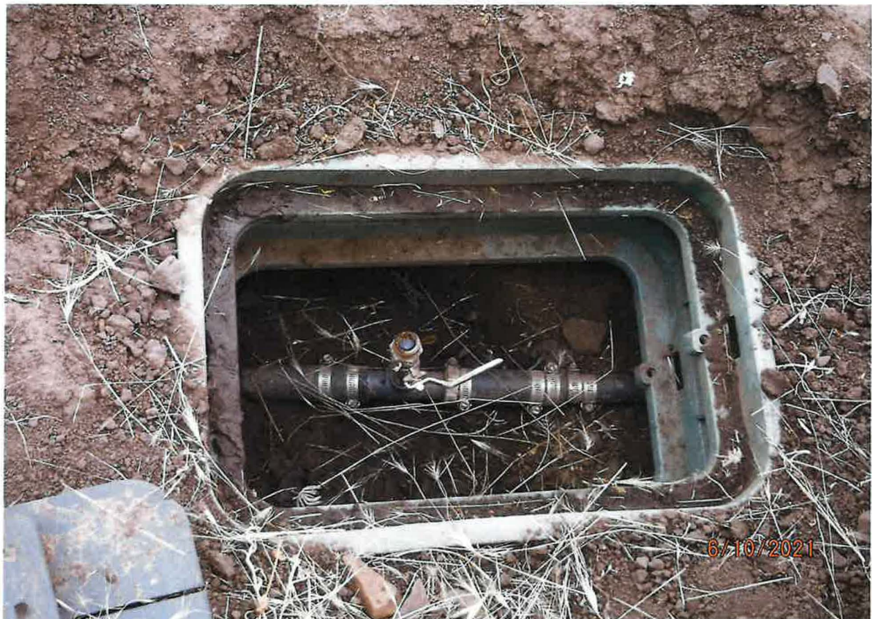
BLEED VALVE INSTALLED \frac{1}{2} WAY FROM POD-TO-POU
