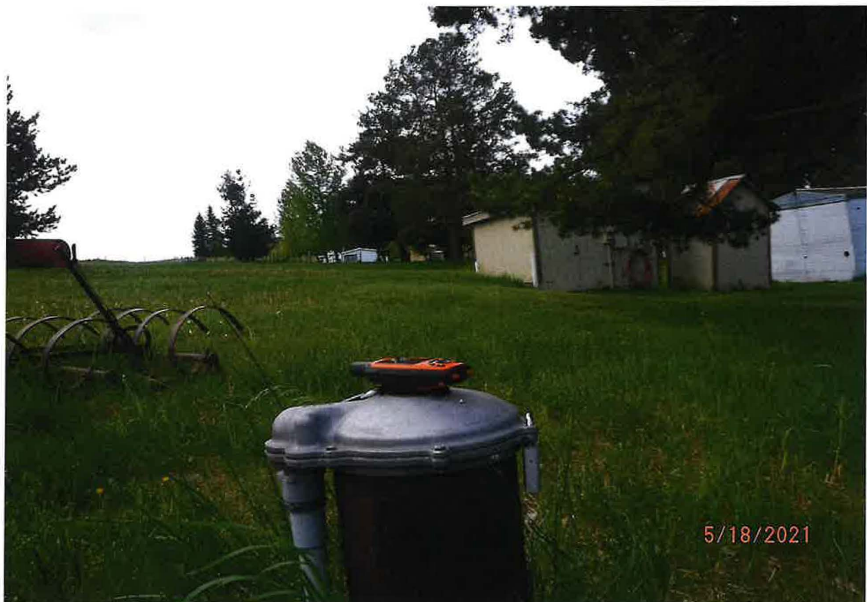
POD – GROUNDWATER WELL (NO WELL DOCUMENTS ON FILE)
