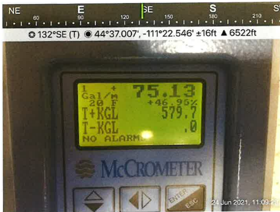
Flow rate for Well No. 1.
