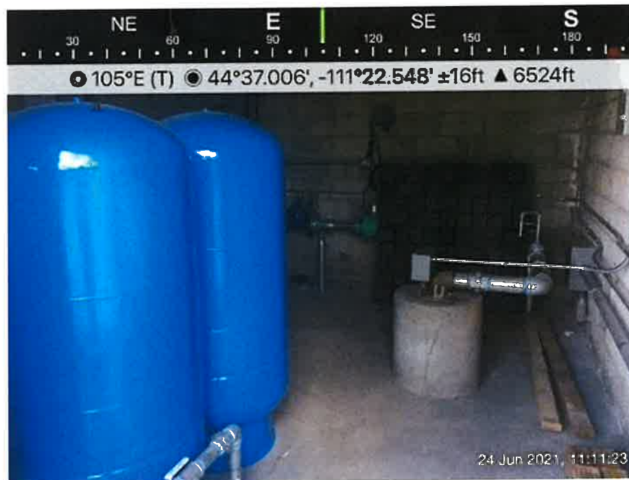
Inside well house for Well No. 1.
