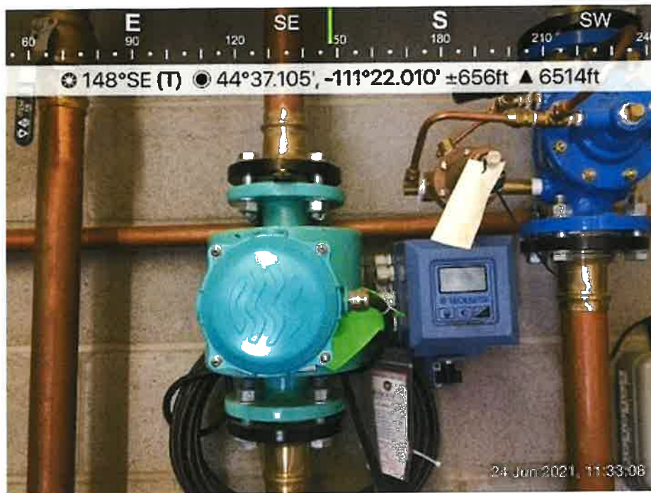
Flow meter for Well No. 2.
