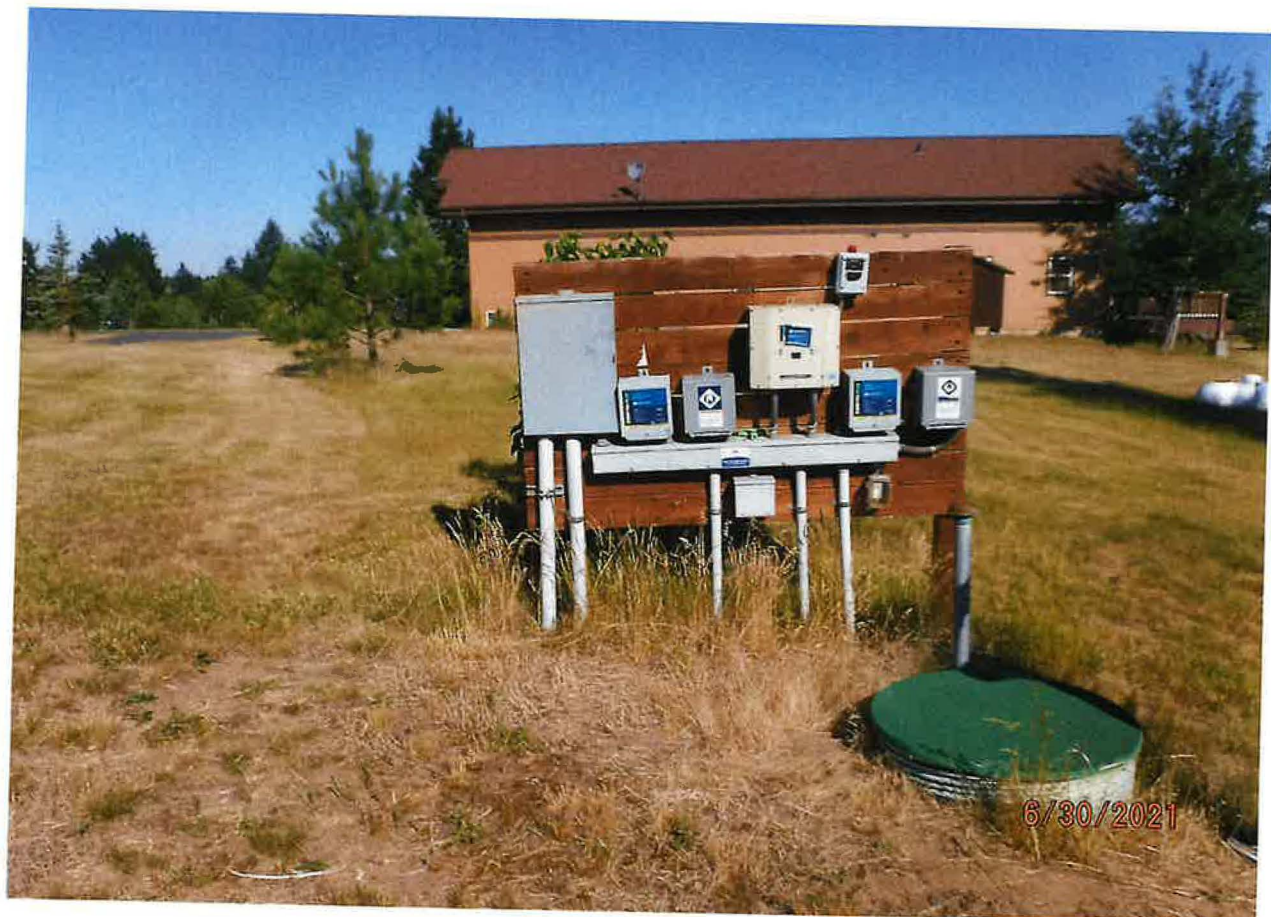
WATER SYSTEM PUMP CONTROL PANEL
