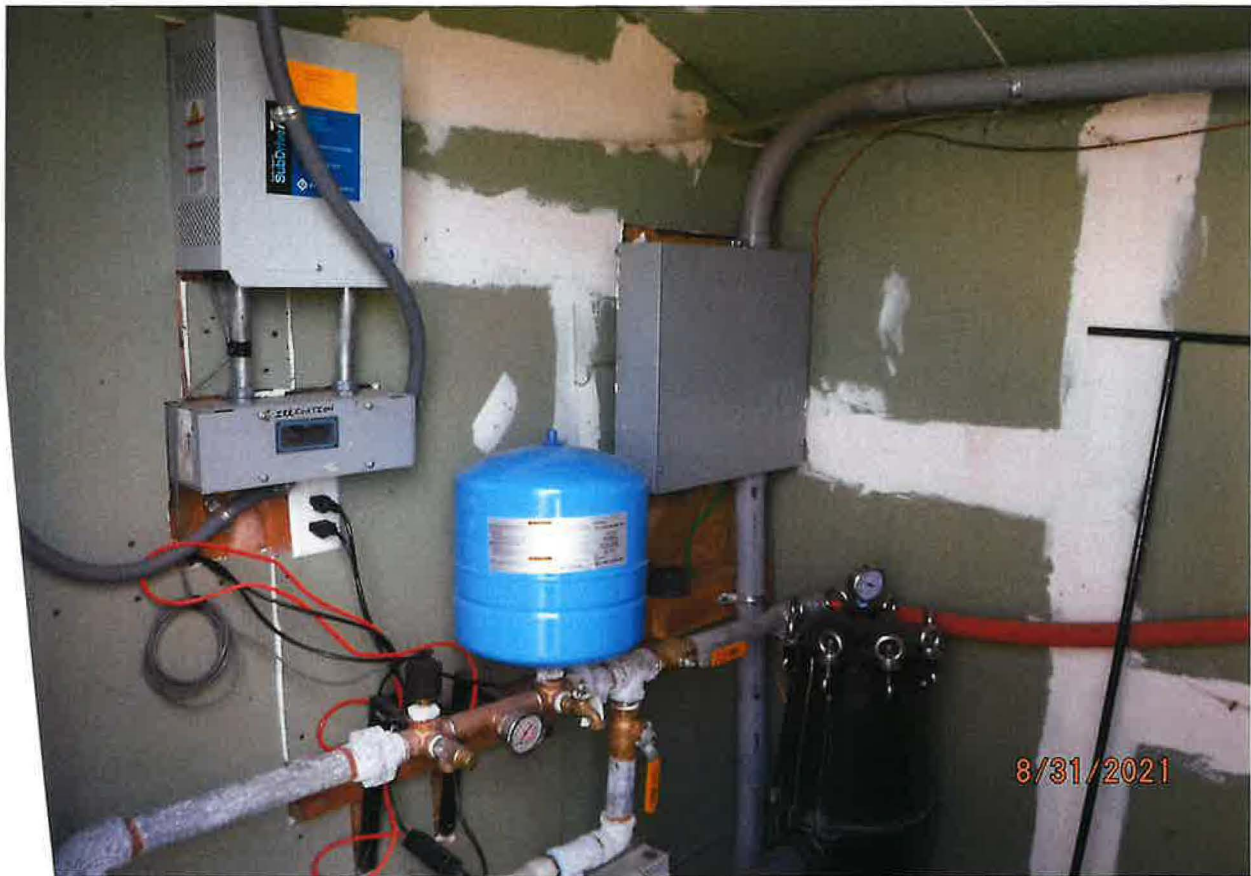
INTERIOR PUMP STATION – SMALL PRESSURE POT
