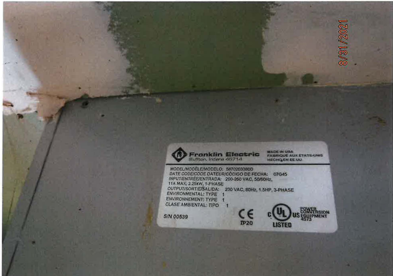
1.5 HP, 3-PHASE PUMP MOTOR INSTALLED IN SYSTEM
