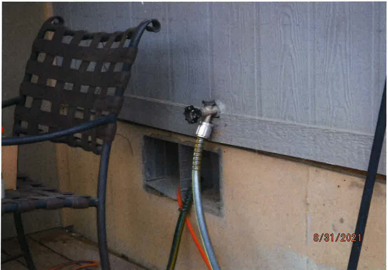
IRRIGATION FROM HOSE BIB(S) ON HOME
