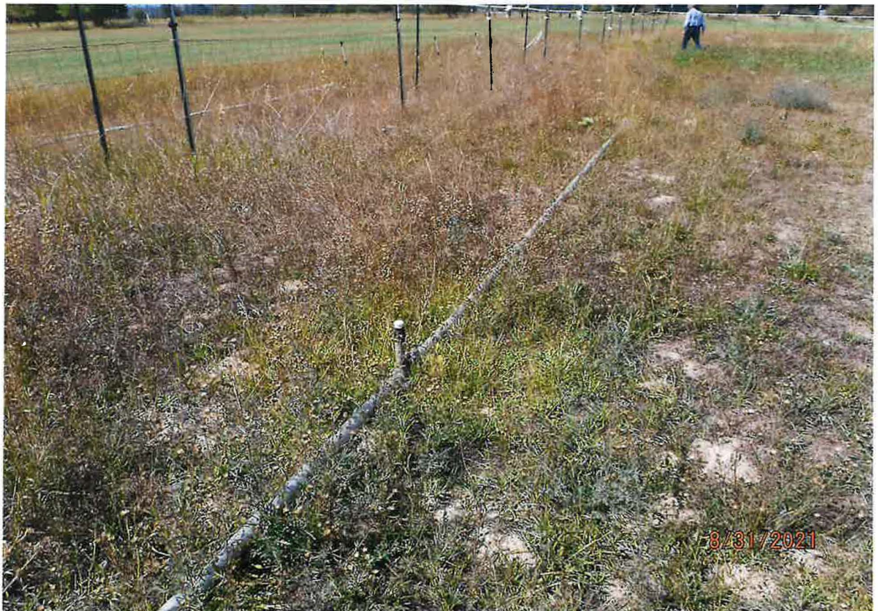
SPRINKLER SYSTEM MAIN LINE
