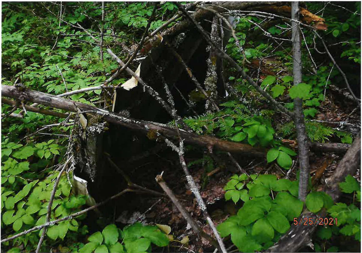
RUN-DOWN STRUCTURE AT POD FOR 1 ST SPRING SOURCE IN NESESW
