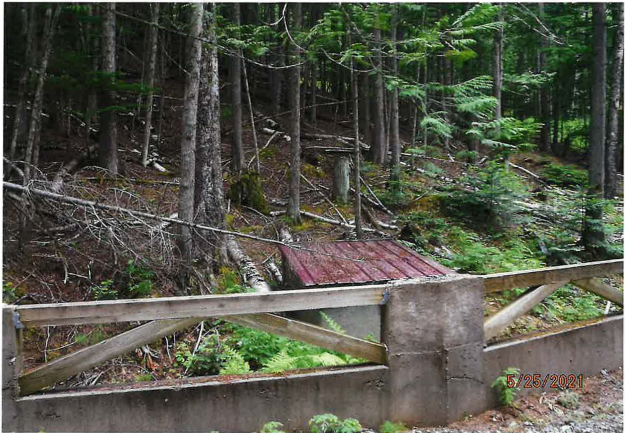
2 ND SPRING SOURCE WITH OVERFLOW PIPER ROUTING BENEATH ROAD
