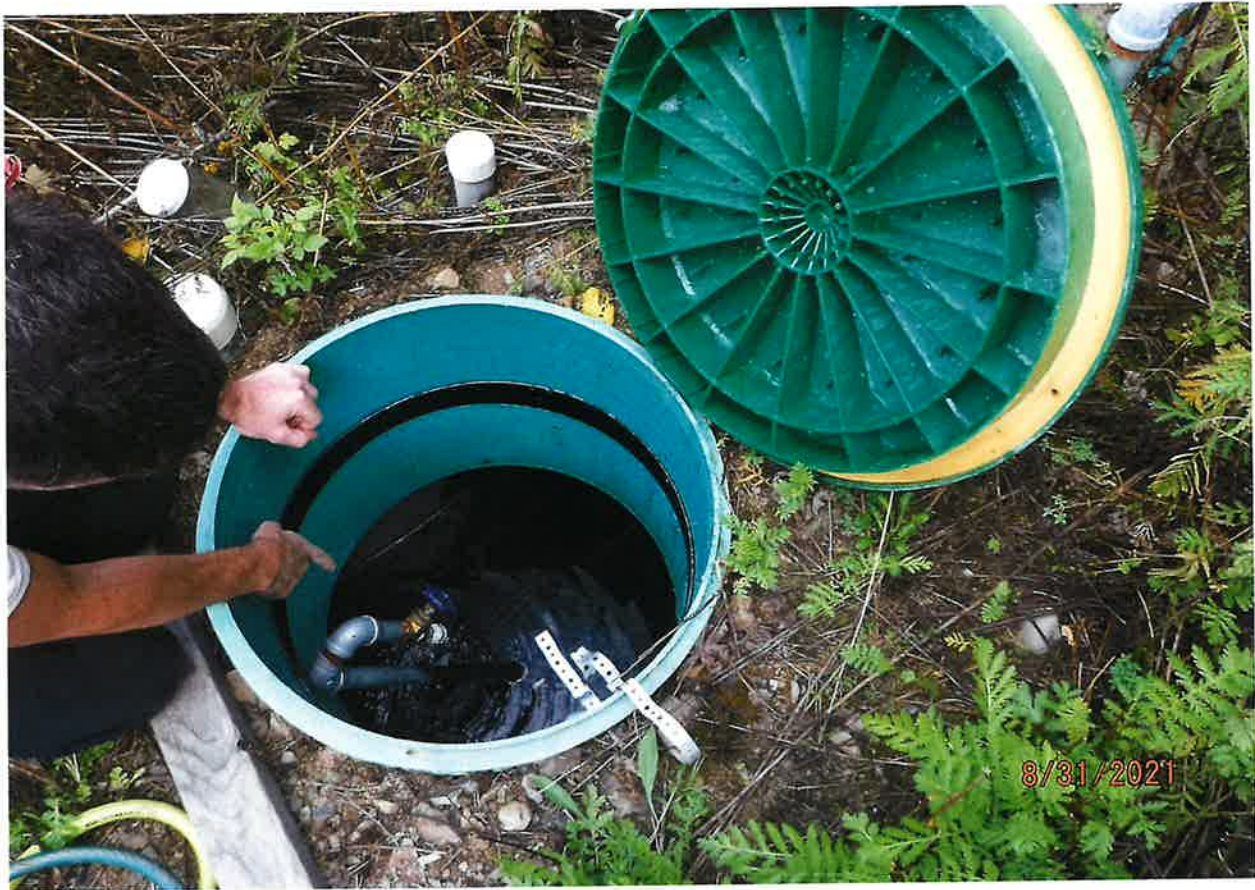
SPRING WATER ROUTED FROM POD TO 1 ST 2500 GAL STORAGE TANK
