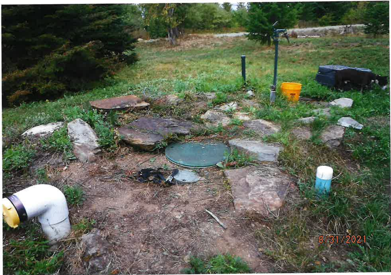
2 ND (LOWER ELEVATION) 2,500 GAL STORAGE TANK LOCATED IN LOT 2, EUEREKA HEIGHTS SUBDIVISION
