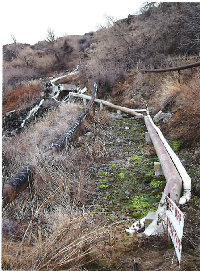
Figure 2: Pipelines from collection box that divert into hatch house.
