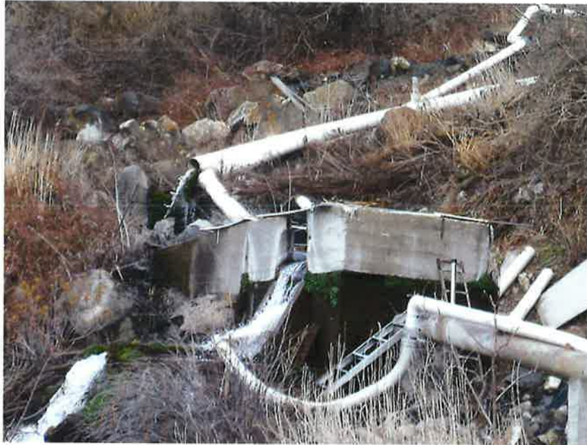
Figure 1: Lower Collection Box (notice the 2 pipes diverting water into box and the two diverting water out)
