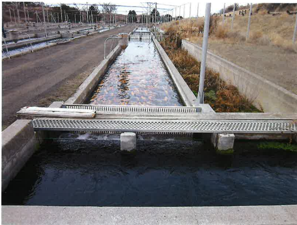
Figure 4: Middle raceway on north end where water diverted from Billingsley Creek enters system
