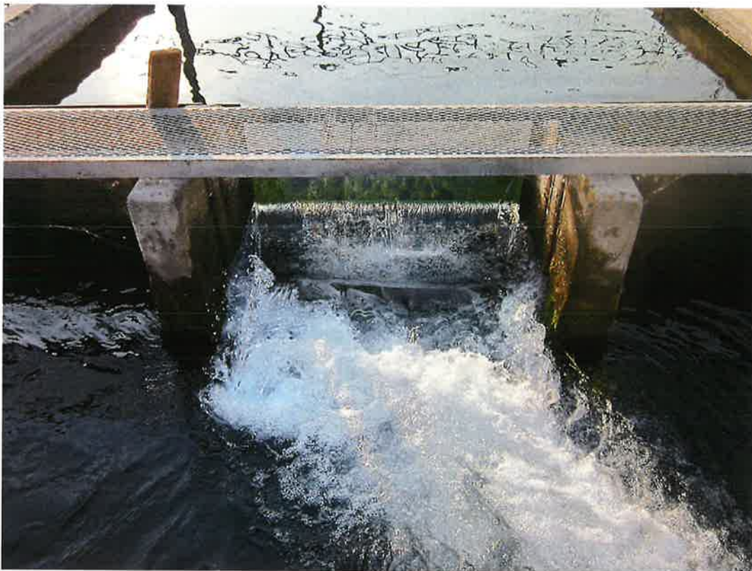
Figure 8: water flowing over south weir out to Billingsley Creek
