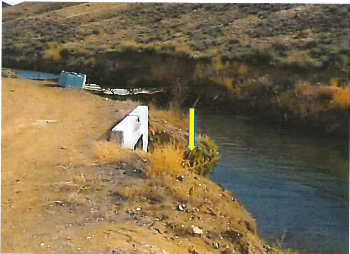
Discharge flow (at arrow) from re-lift pump to canal (Photo from 5/9/2000 Tim Luke memo)
