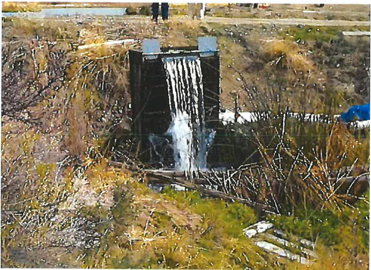
Spillway from settling pond back to Warm Spring Creek (Photo from 5/9/2000 Tim Luke memo)
