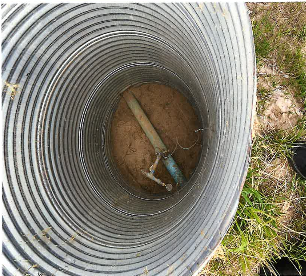
Fig. 12 – Access point for 4" PVC line coming from "Well 1" going to the pump house.
