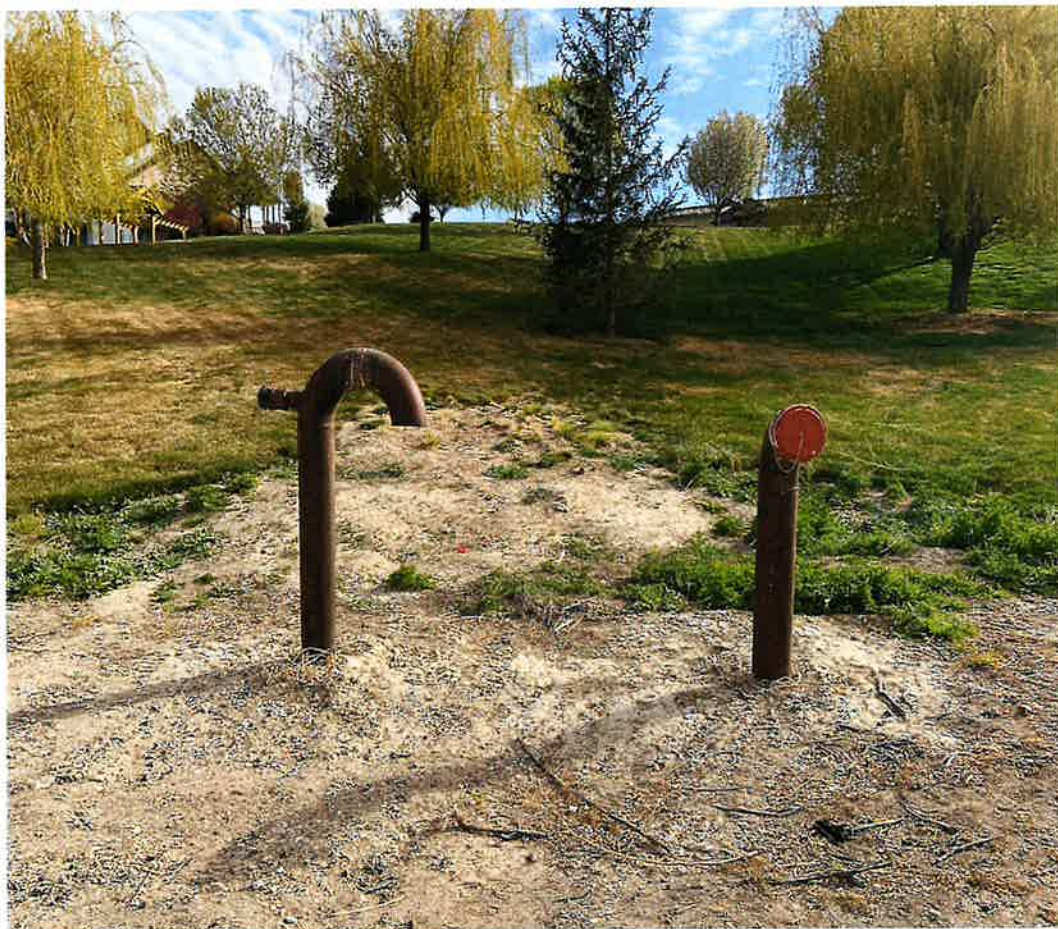
Fig. 15 – Access pipe for the fire protection tank buried on Lot 1, Block 2. Permit holder stated that tanks are between 3 to 6 thousand gallons.
