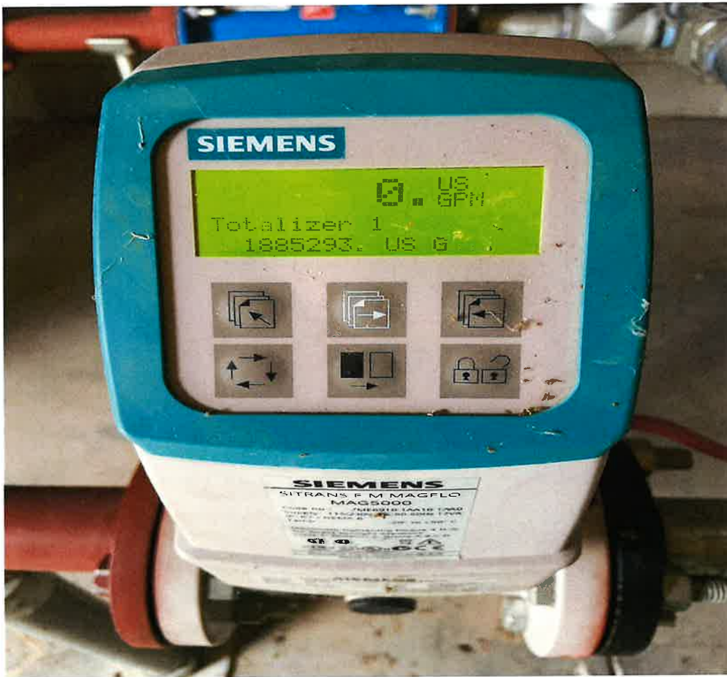
Fig. 5 – Siemens Sitrans F M Magflo MAG5000 installed inline from “Well 1”.
