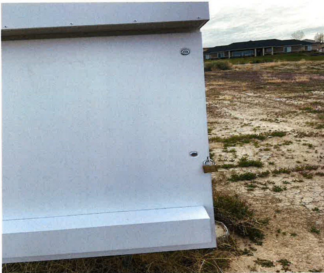
Fig. 14 – The control panel for “Well 1” is lockable and is typically stored locked.
