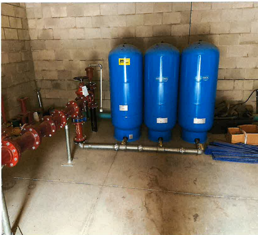
Fig. 10 – Well lines feed into three Amtrol Well-X-Trol WX-350, 119 gallon water pressure tanks. Water is held in the tanks to take pressure off of well pumps during peak demand.
