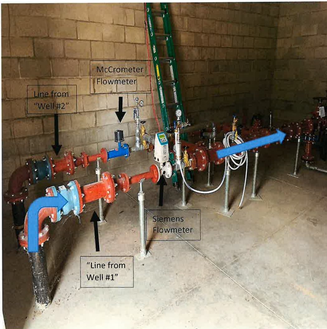
Fig. 4 – View inside of pump house. Line in foreground is from “well 1” and line in background is from “well 2”. Both lines pass through inline measuring devices before heading to the storage tanks.
