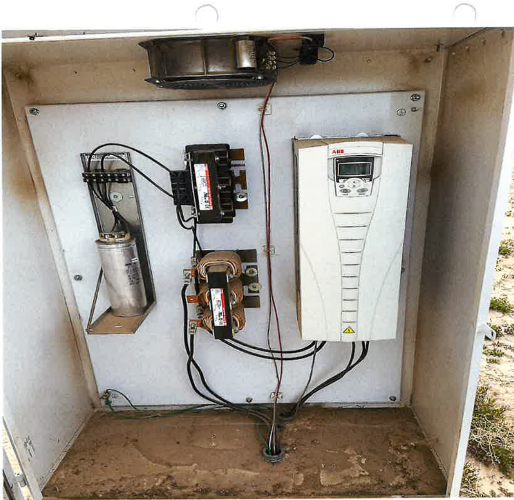
Fig. 13 – Control panel for “Well 1”.
