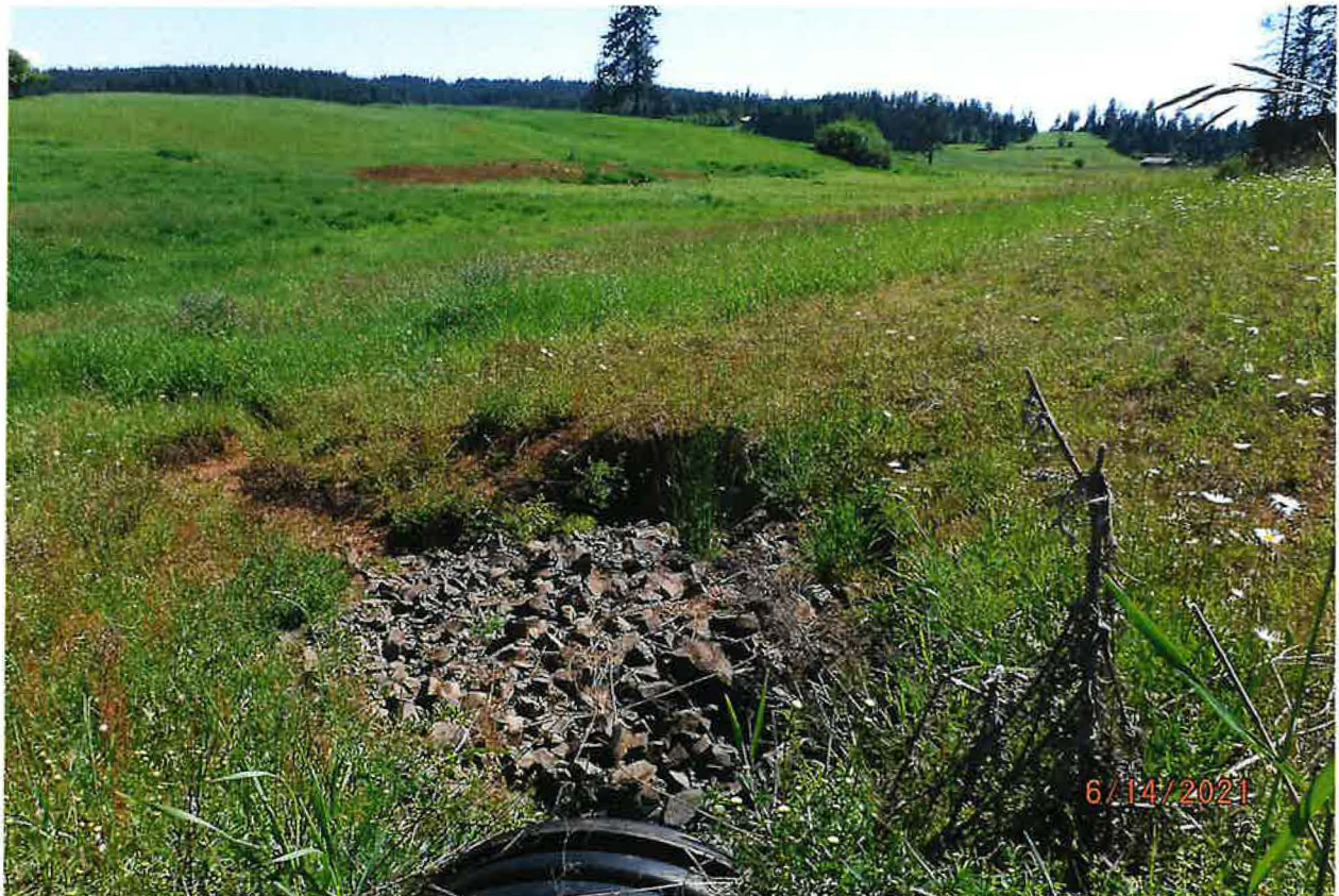
OVERFLOW DISCHARGE PIPE – ROUTES OVERFLOW DOWNSTREAM INTO SMALL DRAINAGE
