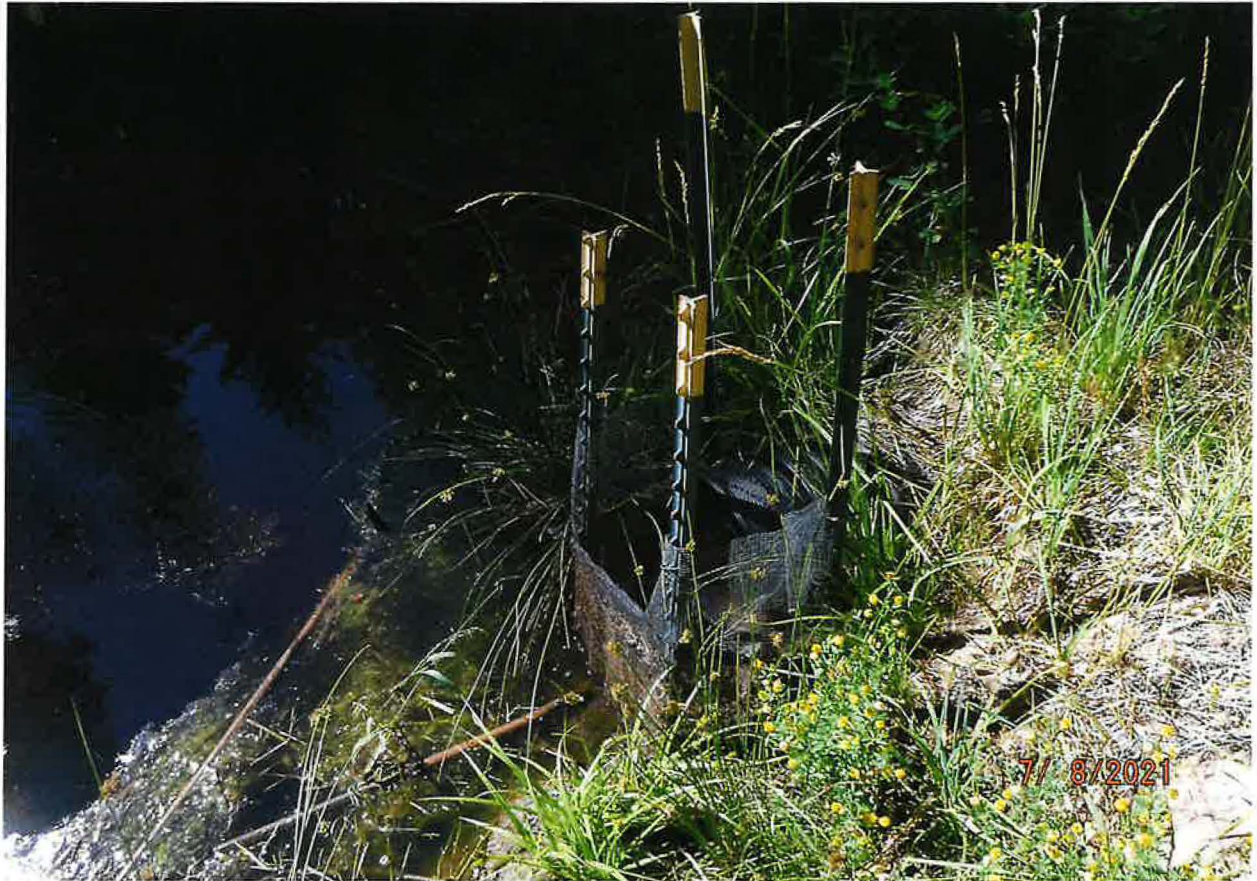
SCREENED OVERFLOW DISCHARGE PIPE – 12 INCH BLACK CORUGATED PIPE
