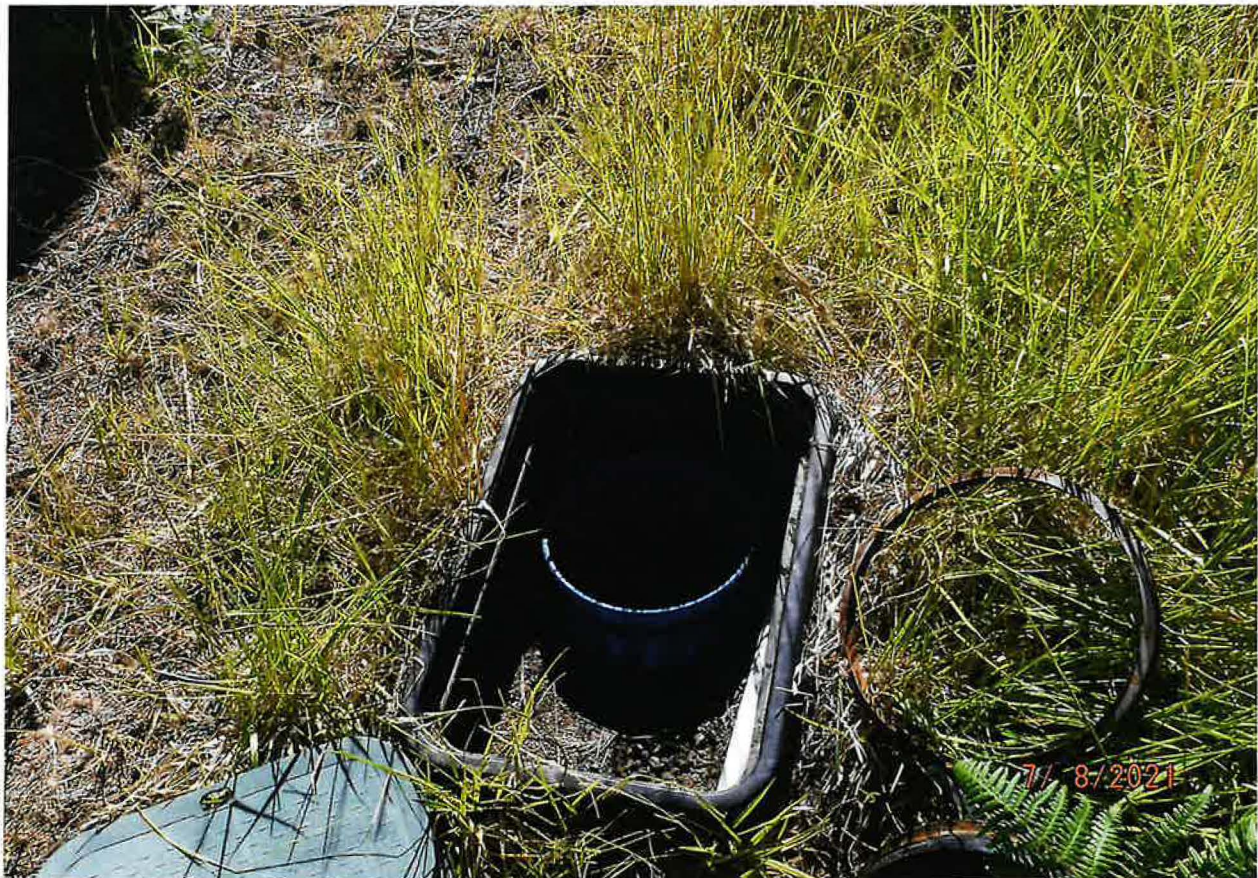
HIGHER ELEVATION SPRING POD - PERFORATED PIPE SPRING BOX TO BUCKET
