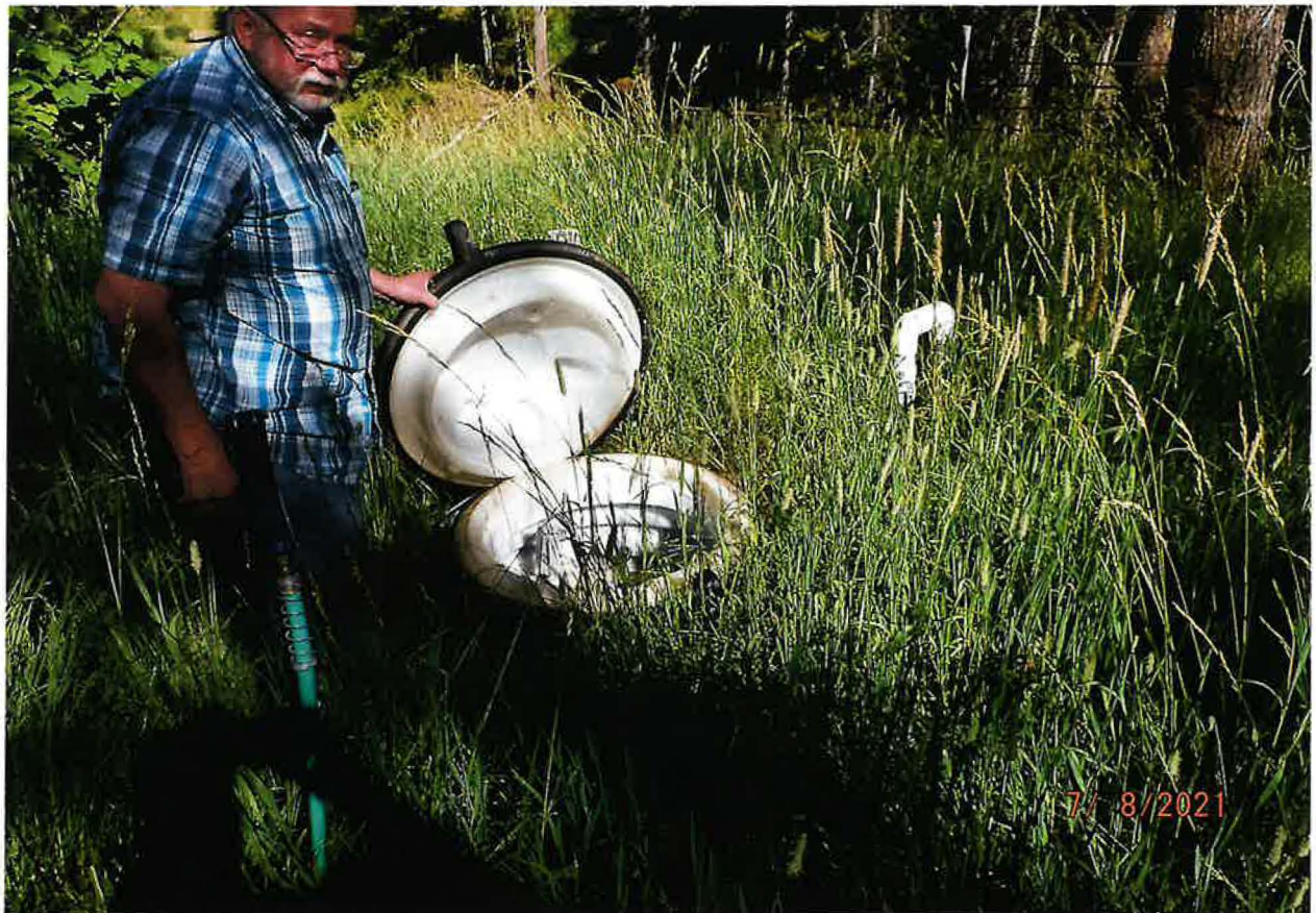
2EA SPRING POD HAVE PVC PIPE THAT FLOW INTO VAULTED 1,100 GALLON CISTERN
