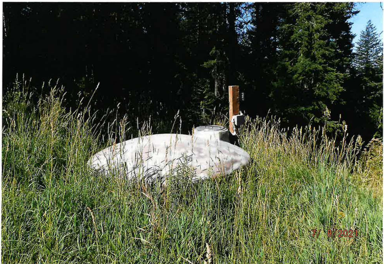
1,600 GAL STORAGE TANK – RECEIVES WATER FROM CISTERN, AND APPLIES GRAVITY FLOW TO POU
