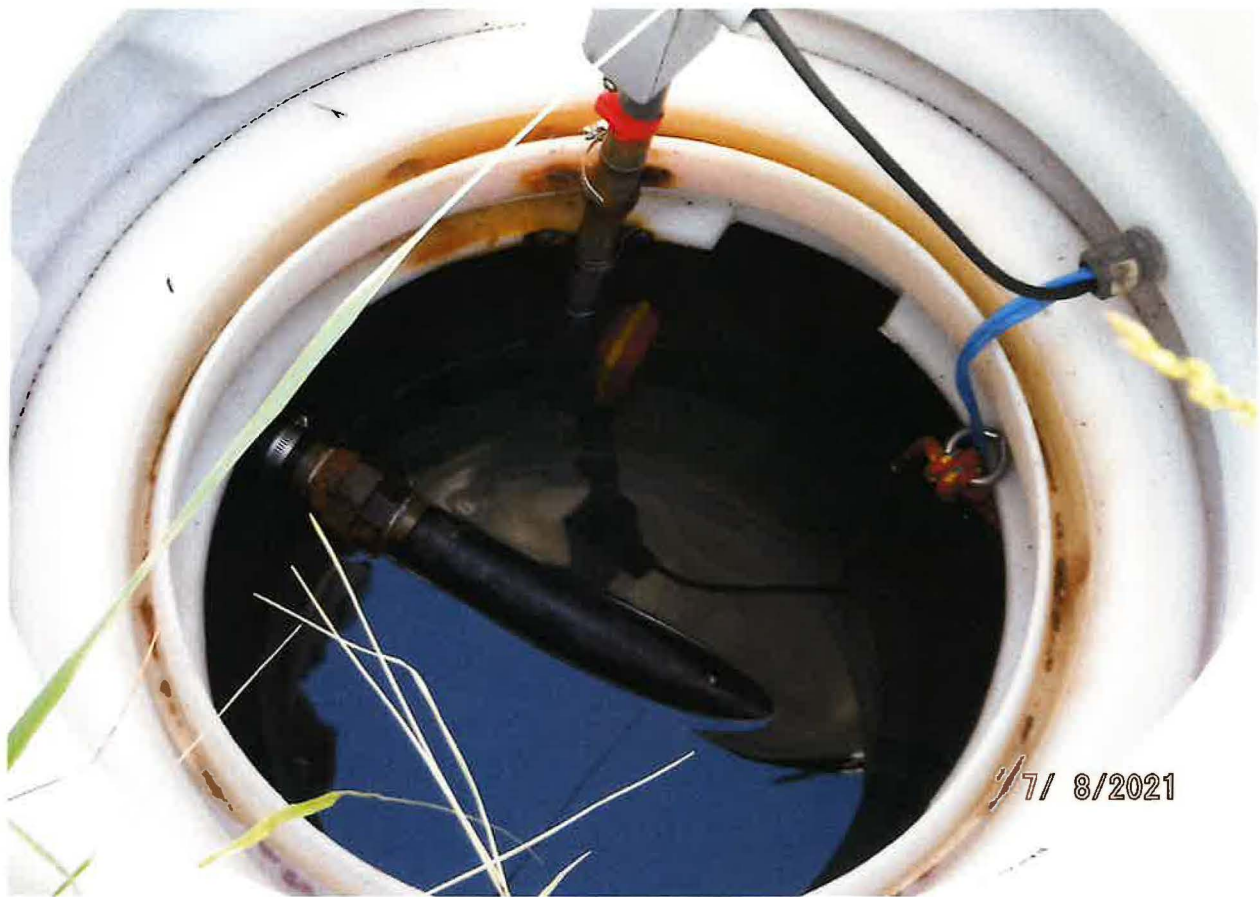
1,100 GAL CISTERN – WATER PUMPED FROM CISTERN UPGRADE TO SECONDARY STORAGE TANK
