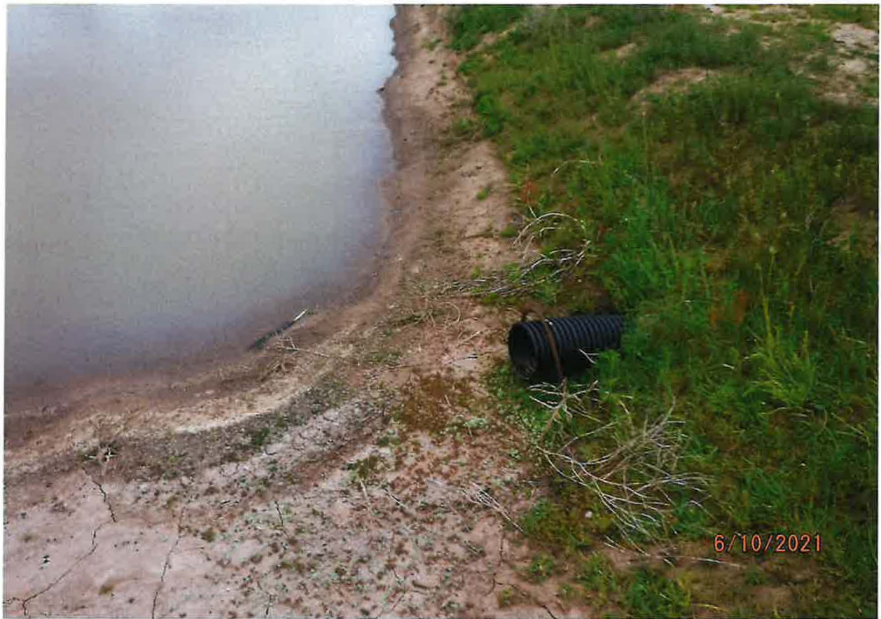
PRIMARY OVERFLOW DEVICE (NW CORNER OF POND)
