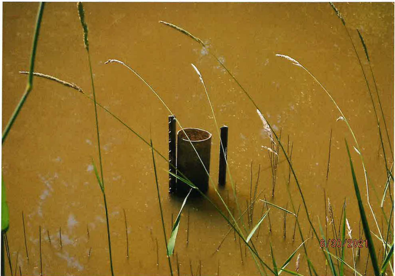
OVERFLOW DISCHARGE PIPE LOCTED IN POND
