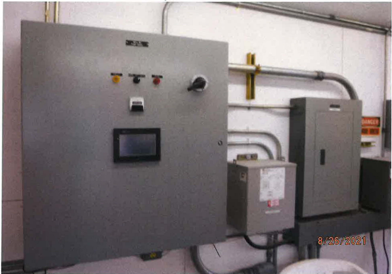
WATER SYSTEM CONTROL PANEL(S)
