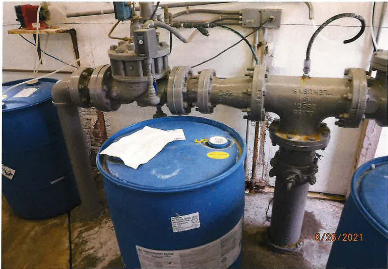
INFLOW MAIN FROM WELL #2, AND SMALLER OVERFLOW DISCHARGE PIPE
