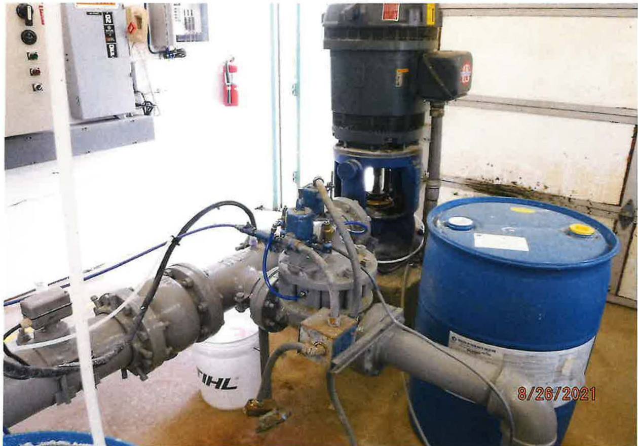
INFLOW MAIN FROM WELL #1 AND SMALLER OVERFLOW DISCHARGE PIPE
