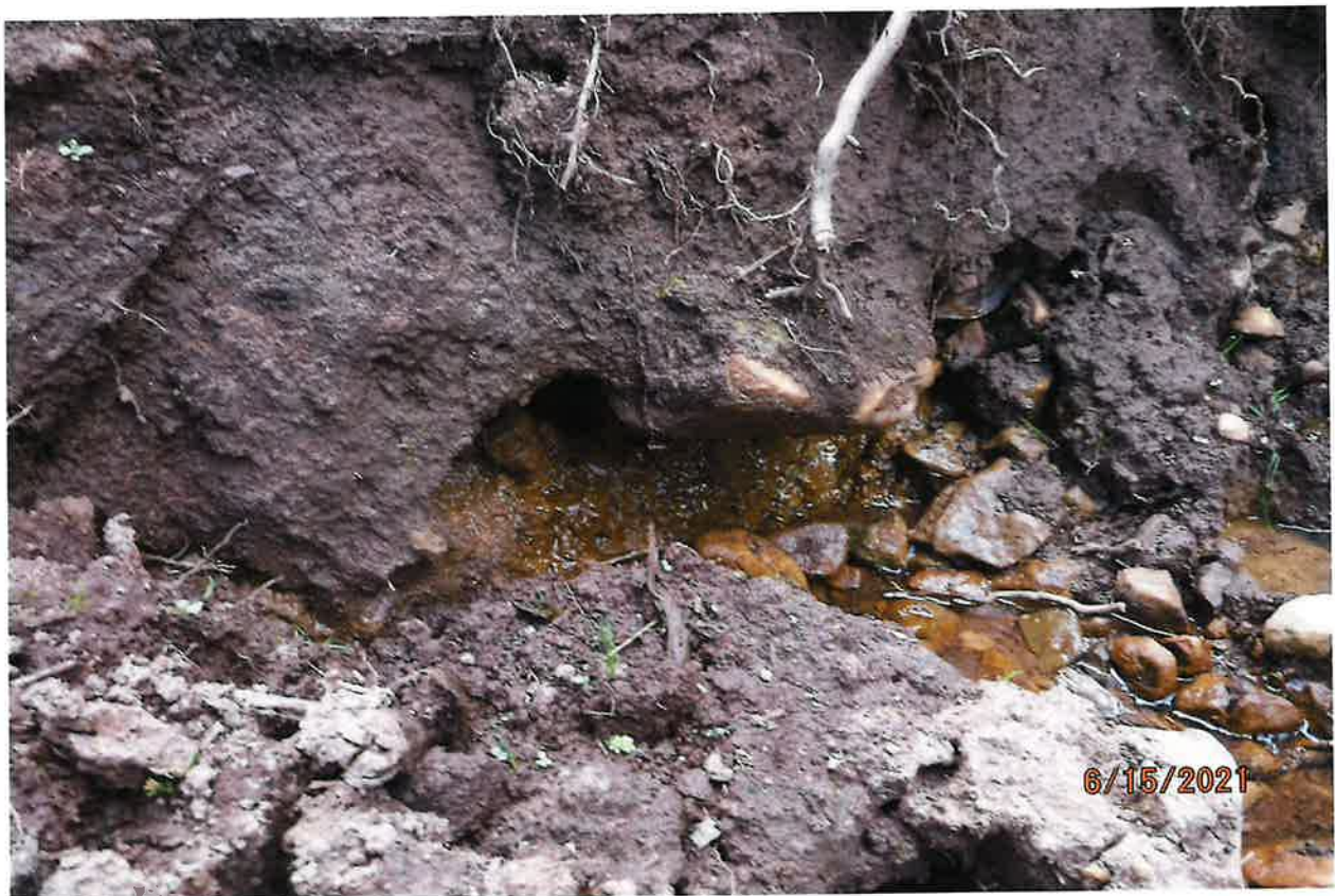
POD – SPRING FLOW FROM BANK
