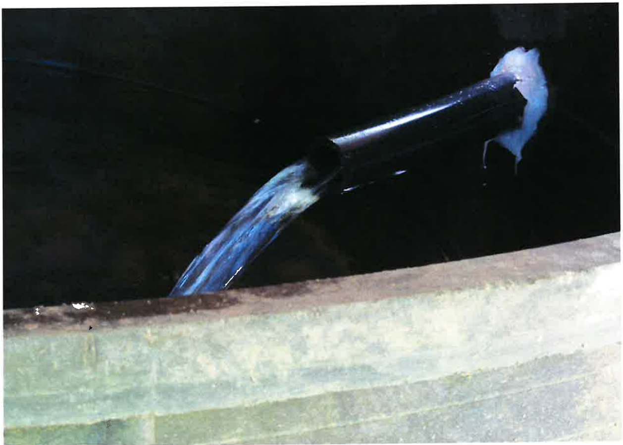
AT POD – 1 INCH BURIED SPRING BOX TO RUBBER & CONCRETE CISTERN
