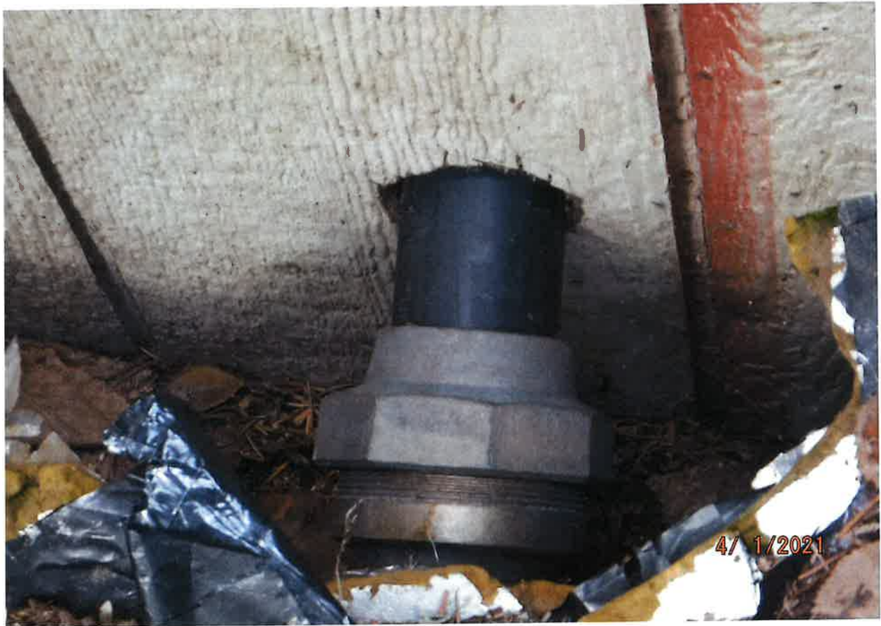
2 INCH POLY PIPE INFLOW TO HYDRO POWER STATION
