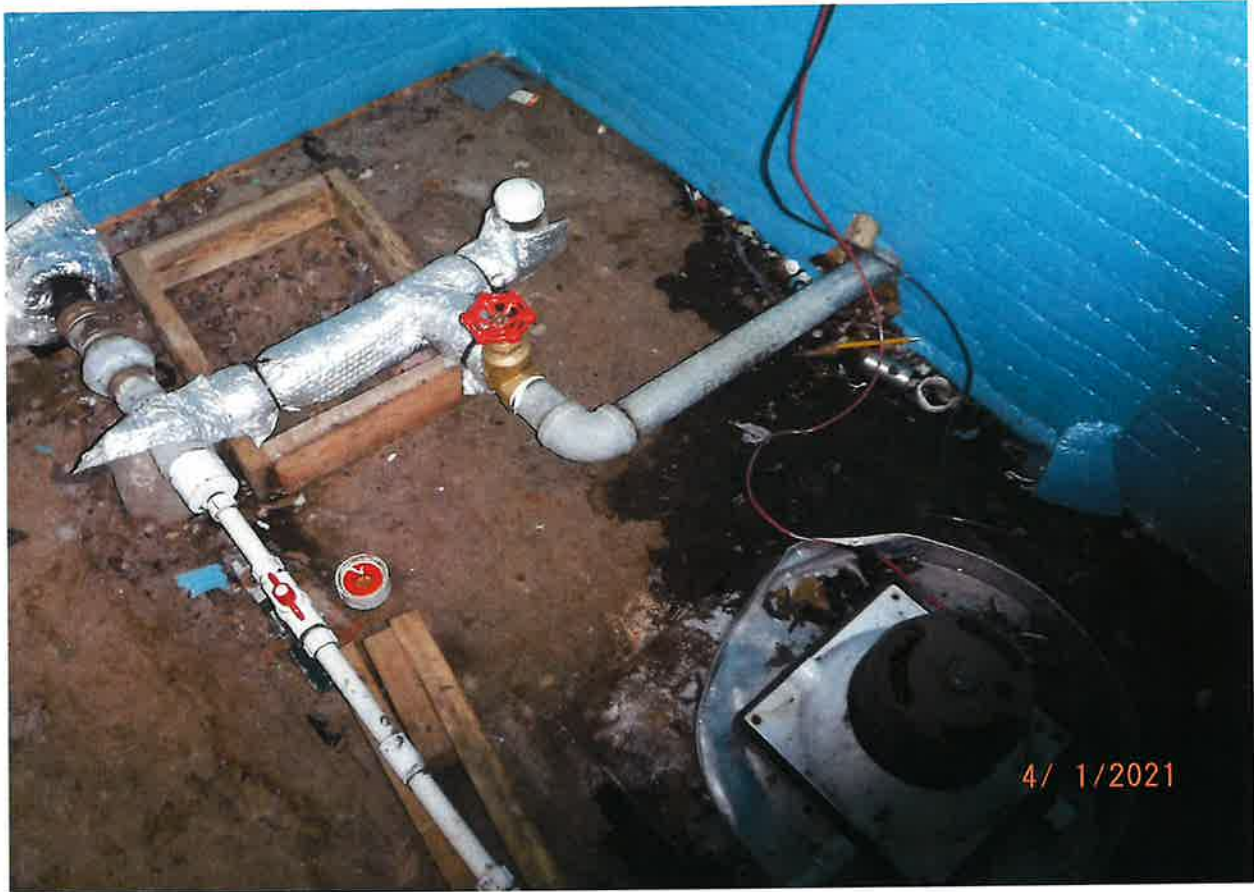
POU - HYDRO POWER SYSTEM
