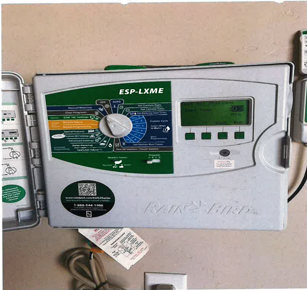
Fig. 3 – The sprinkler irrigation from the well is operated by this Rain Bird controller and is set to automatically irrigate the place of use on a timer.
