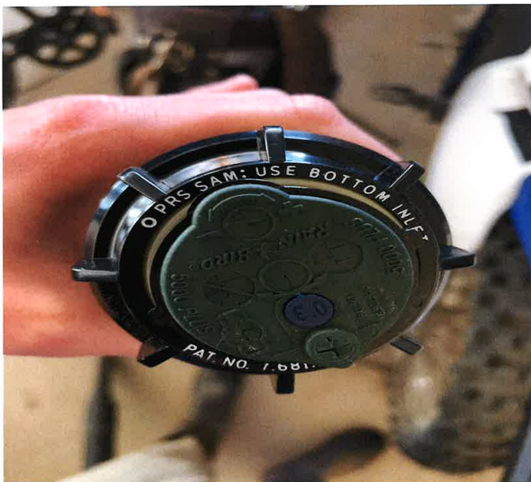
Fig. 6 – The sprinkler heads are Rain Bird 5000 Plus and are installed throughout the place of use.
