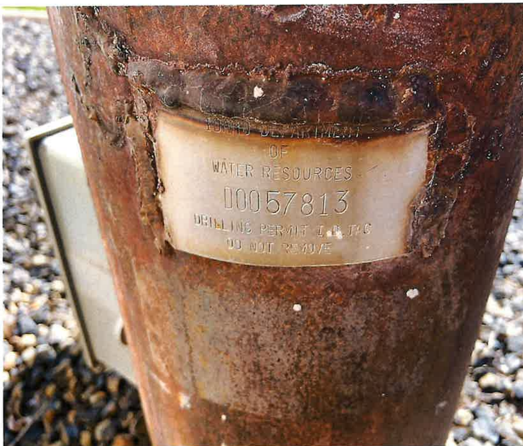
Fig. 2 – Well tag ID D0057813 was drilled by Treasure Valley Drilling and completed in 2010.
