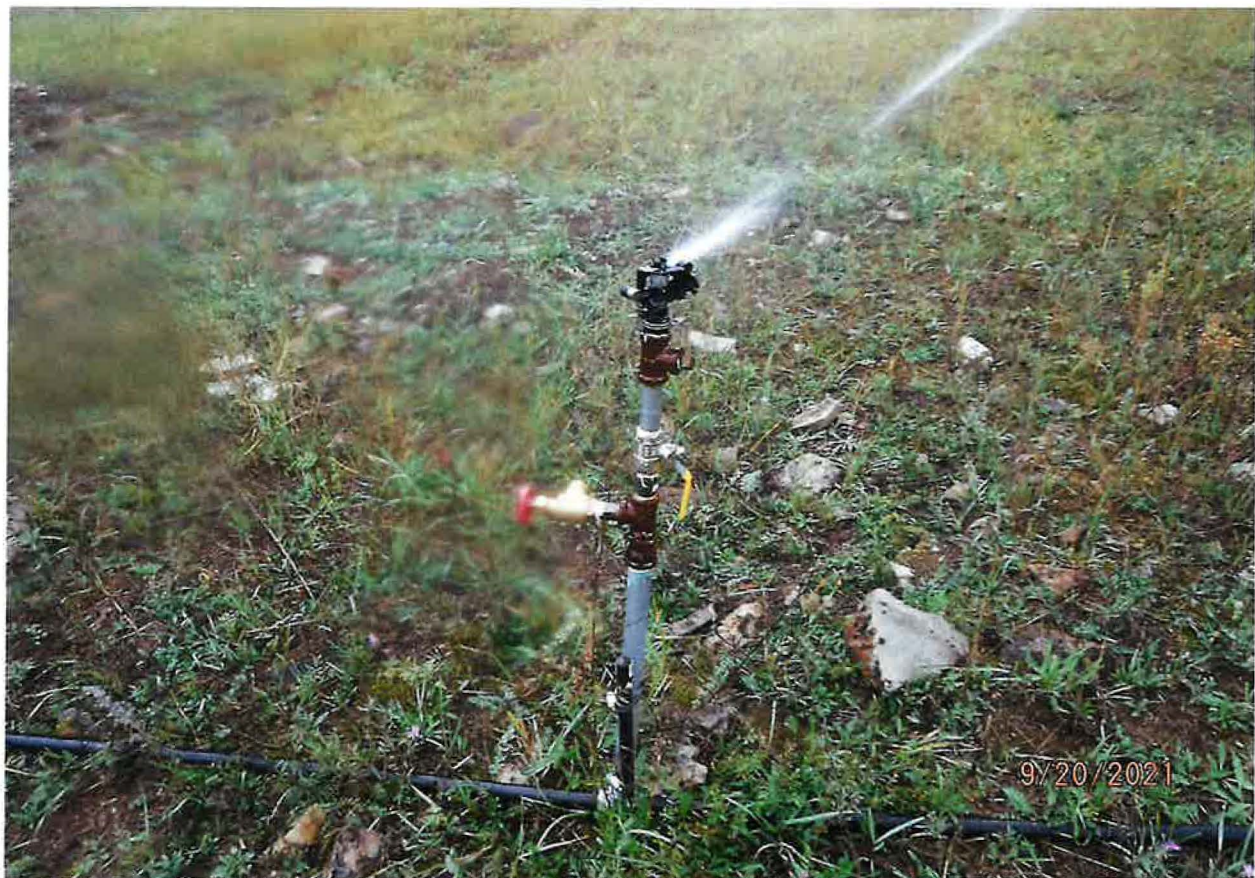
4EA ½ SPRINKLER RISER PIPES WITH HOSE BIB AND SPRINKLER ATTACHMENTS ALONG RIVER
