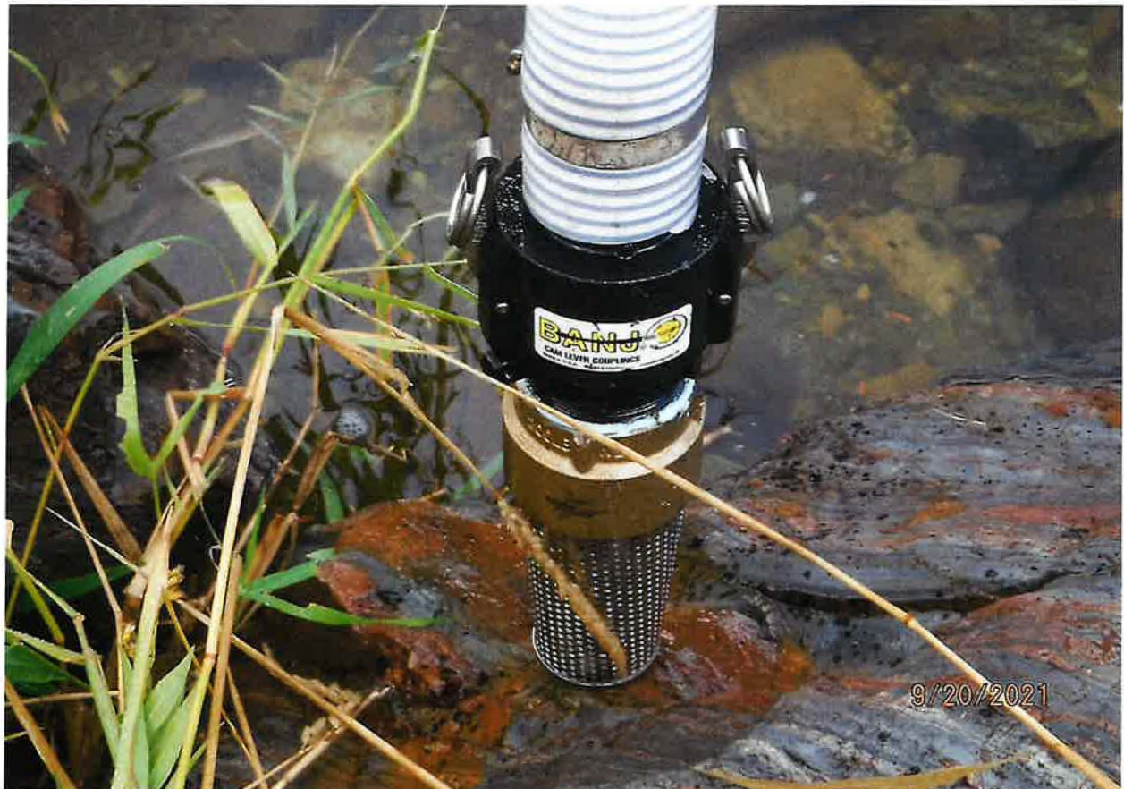
POD – SCREENED INTAKE PIPE TO PUMP FROM RIVER
