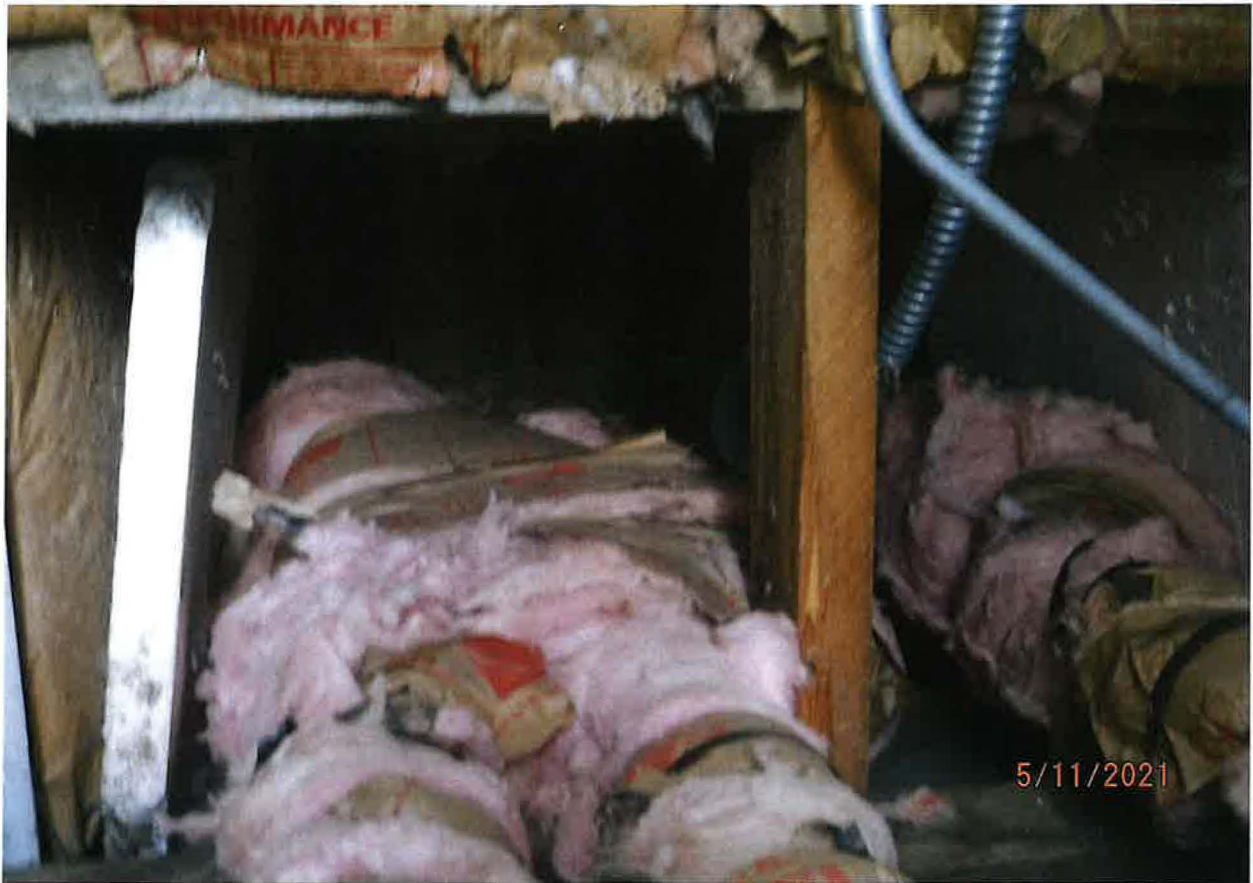
PIPING FROM WELL 95-80-N-90
