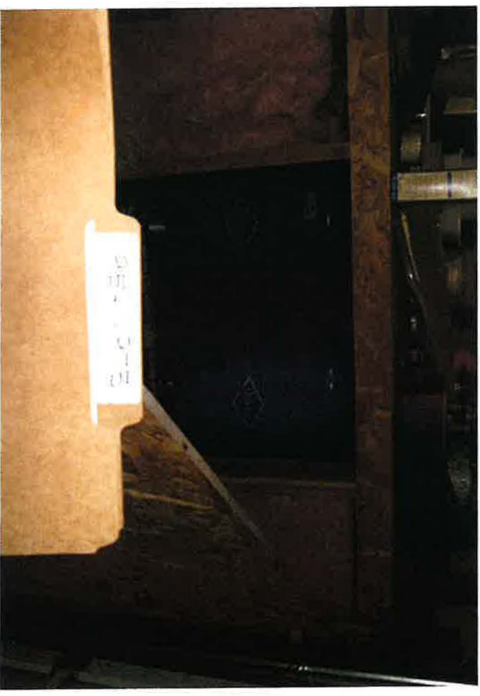
95-11975 Pressure Tanks in Outbuilding
