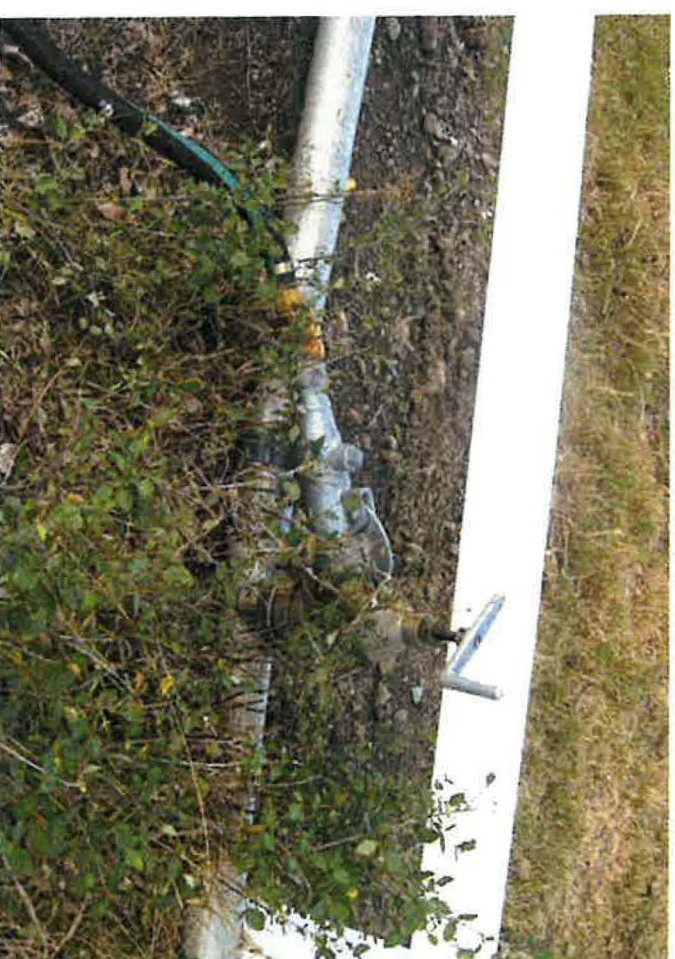
95-11975 3" Main Line, valve, & Hose to unit
