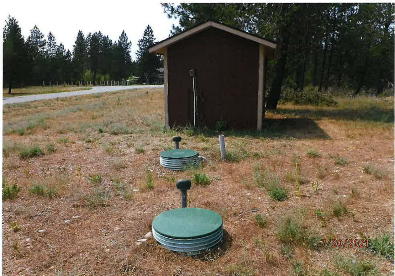
PUMP HOUSE WITH 2EA 2,500 GAL STORAGE TANKS
