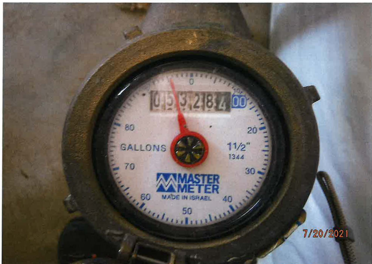
MASTER METER FLOWMETER INSTALLED ON SYSTEM
