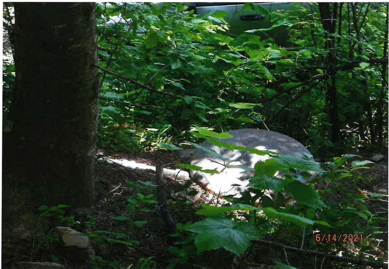
PARTIALLY BURIED STORAGE TANK COLLECTS SPRING WATER PRIOR TO PUMPING TO POU
