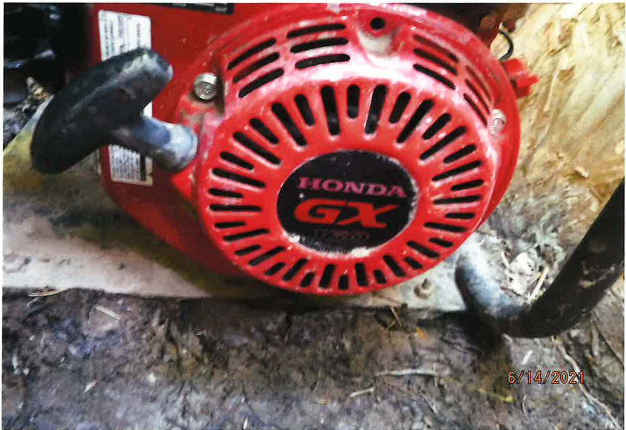
HONDA GX160 WATER TRANSFER PUMP – PUMPS WATER FROM POD STORAGE TANK UPHILL TO POU VIA ¾ INCH POLY PIPE
