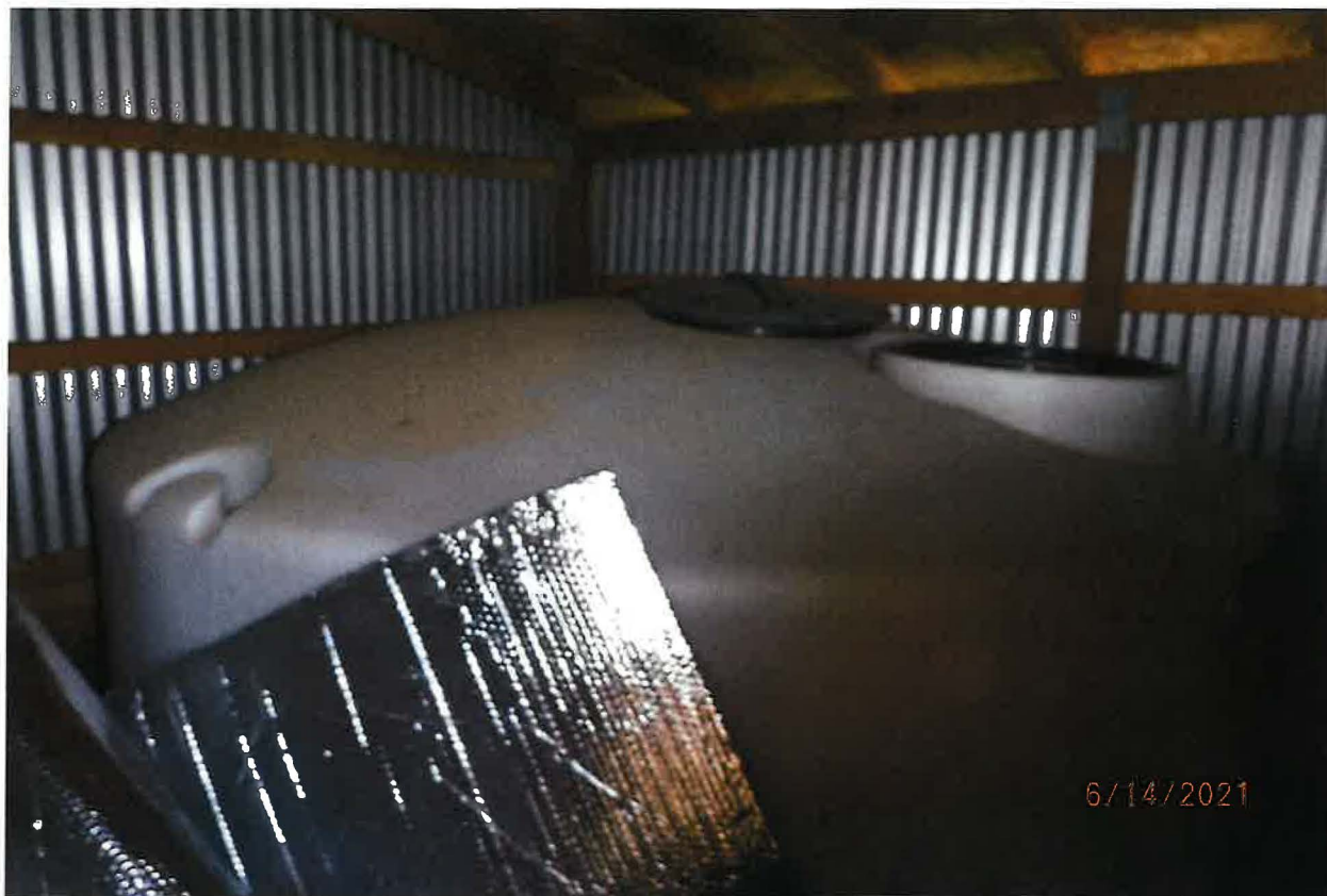
1,500 GALLON STORAGE TANK IN SMALL SHED CO-LOCATED WITH HOME
