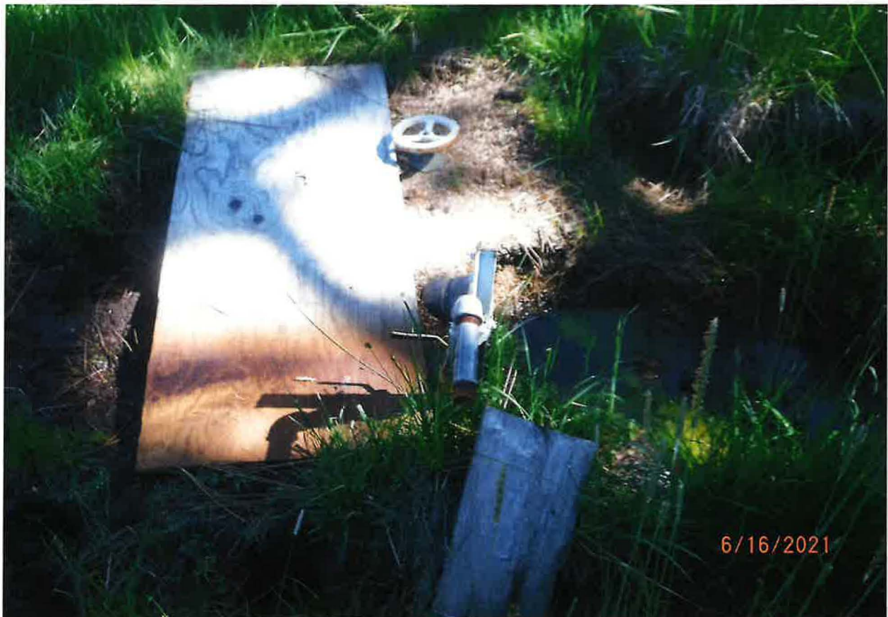
FROM STORAGE USE(S) RISER PIPE AND VALVE
