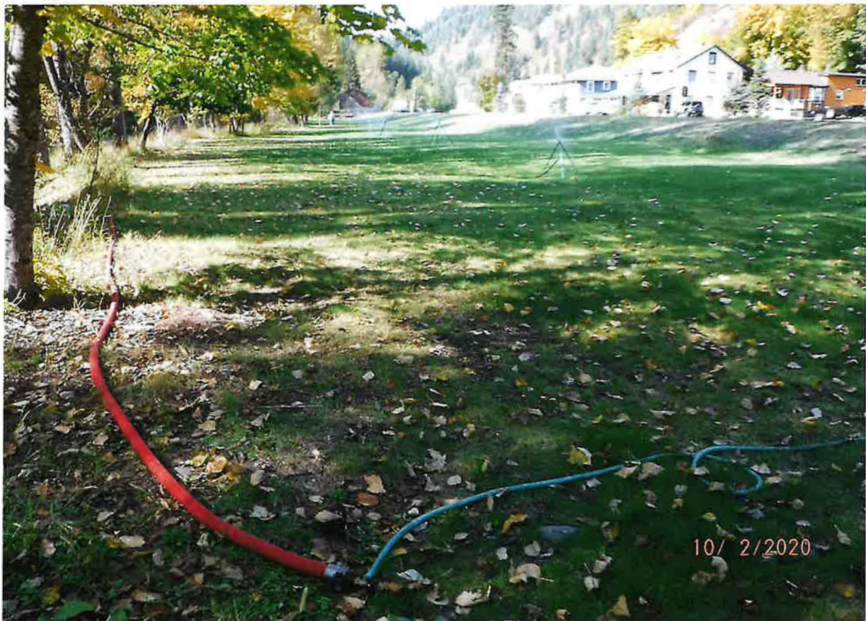
IRRIGATION RISER CONNECTIONS TO HOSE AND TRIPOD SPRINKLER AT INTERVAL ON MAIN TRUNK LINE
