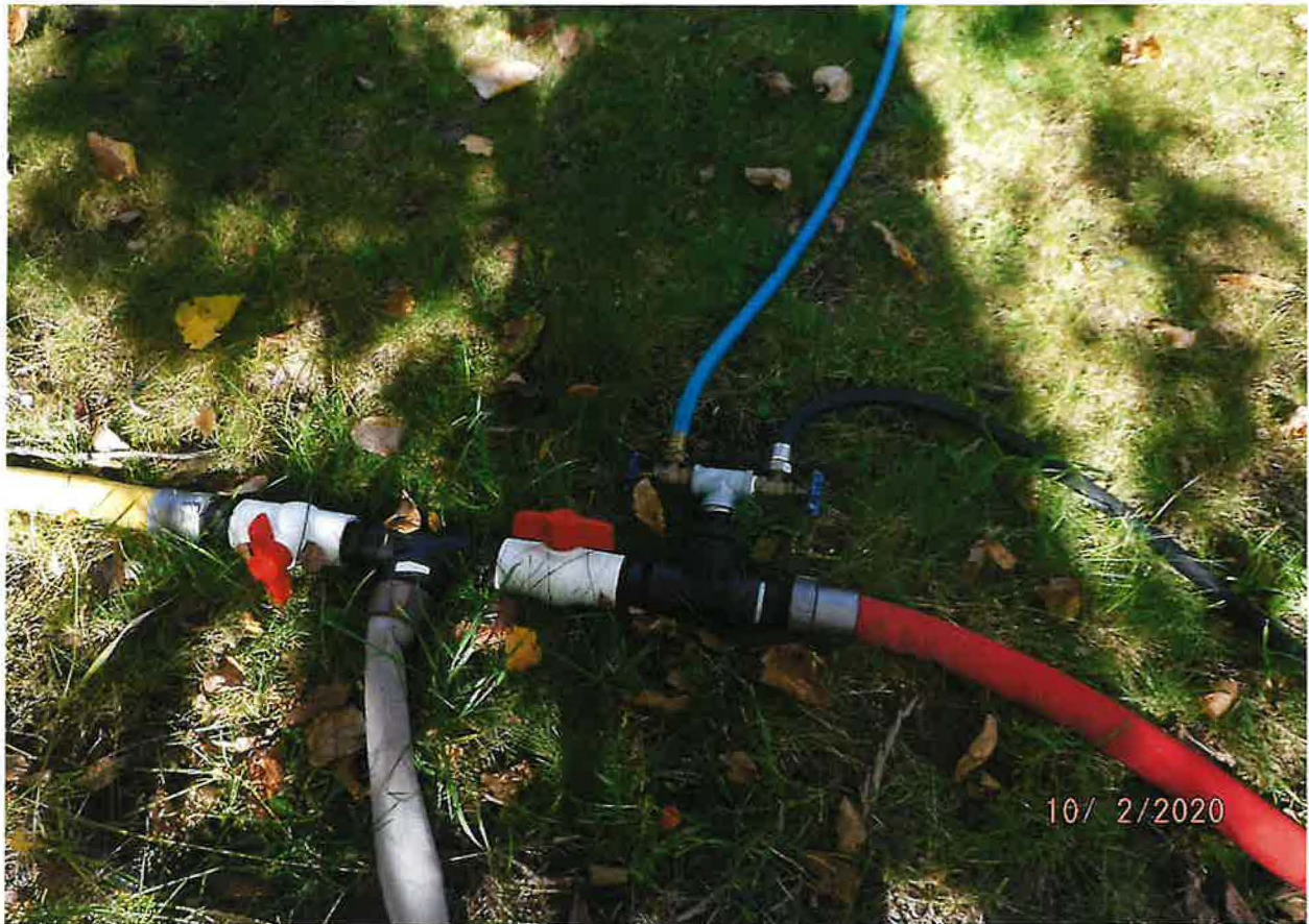
FIRE PROTECTION & IRRIGATION POU – WATER SYSTEM DELIVERY LINE MAIN TEE JUNCTION
