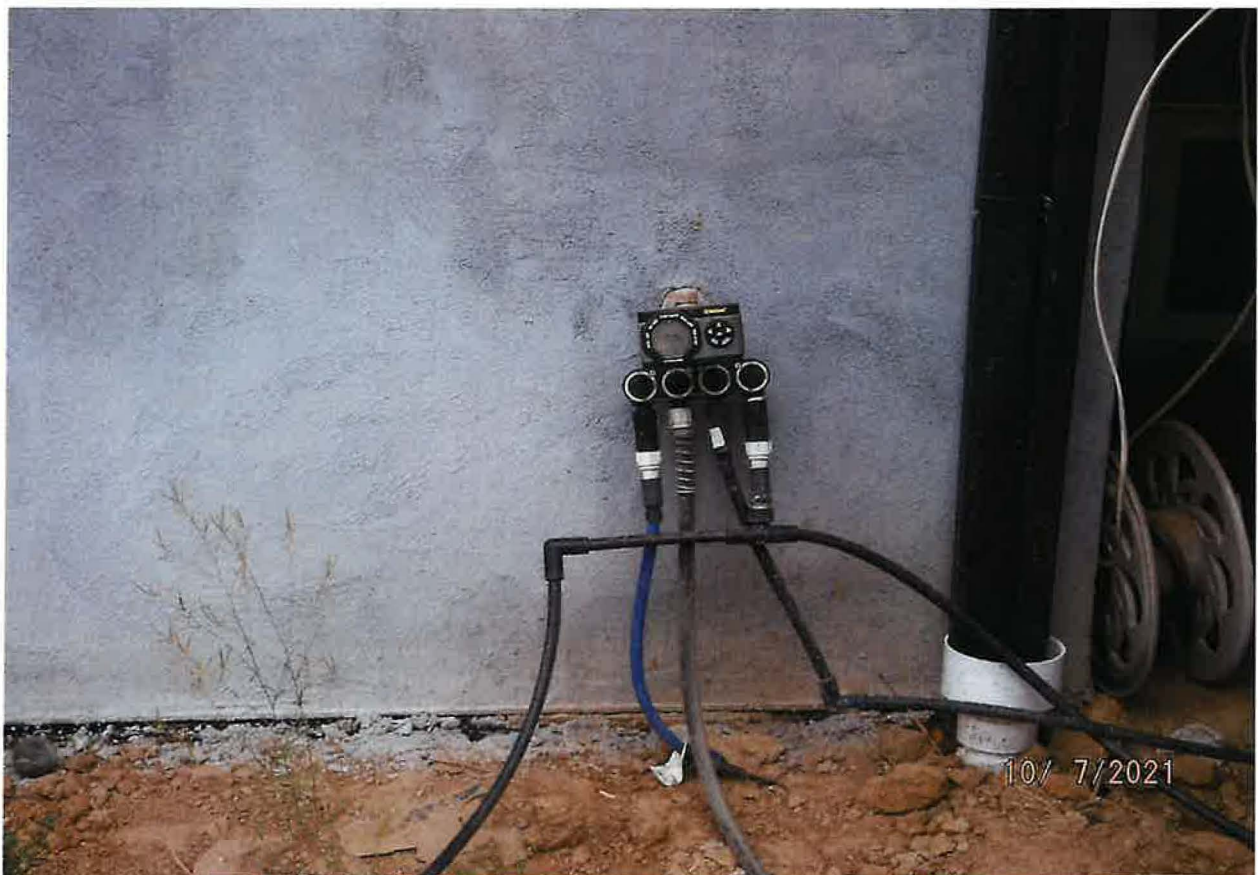
IRRIGATION SYSTEM CONNNECTIONS
