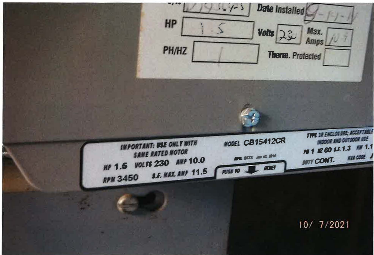
1.5 HP PUMP MOTOR INSTALLED ON PUMP IN WELL
