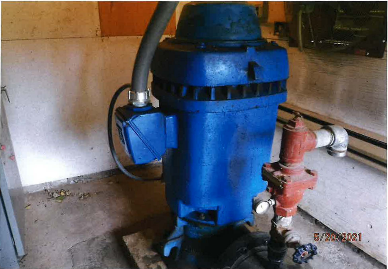
WELL # 1 - 125 HP PUMP INSTALLED
