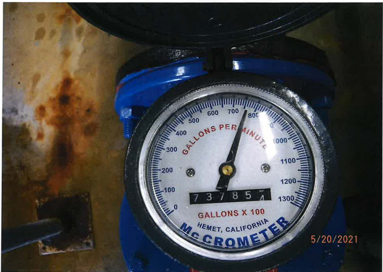
WELL #1 FLOW METER MEASURED 770 GPM
