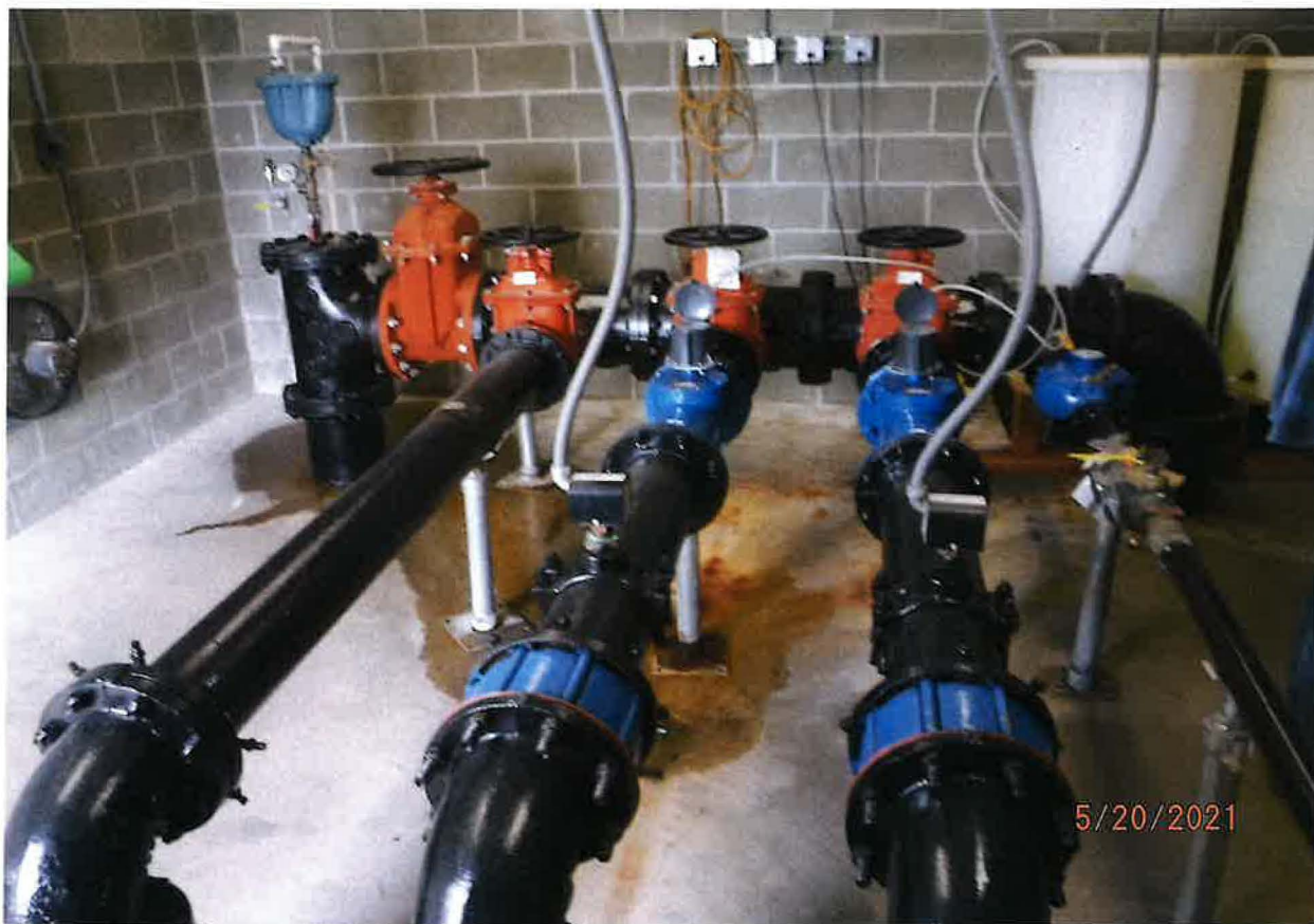
INTERIOR PUMP STATION – MIDDLE TWO WATER MAINS ARE #1 & #3 WELL(S)
