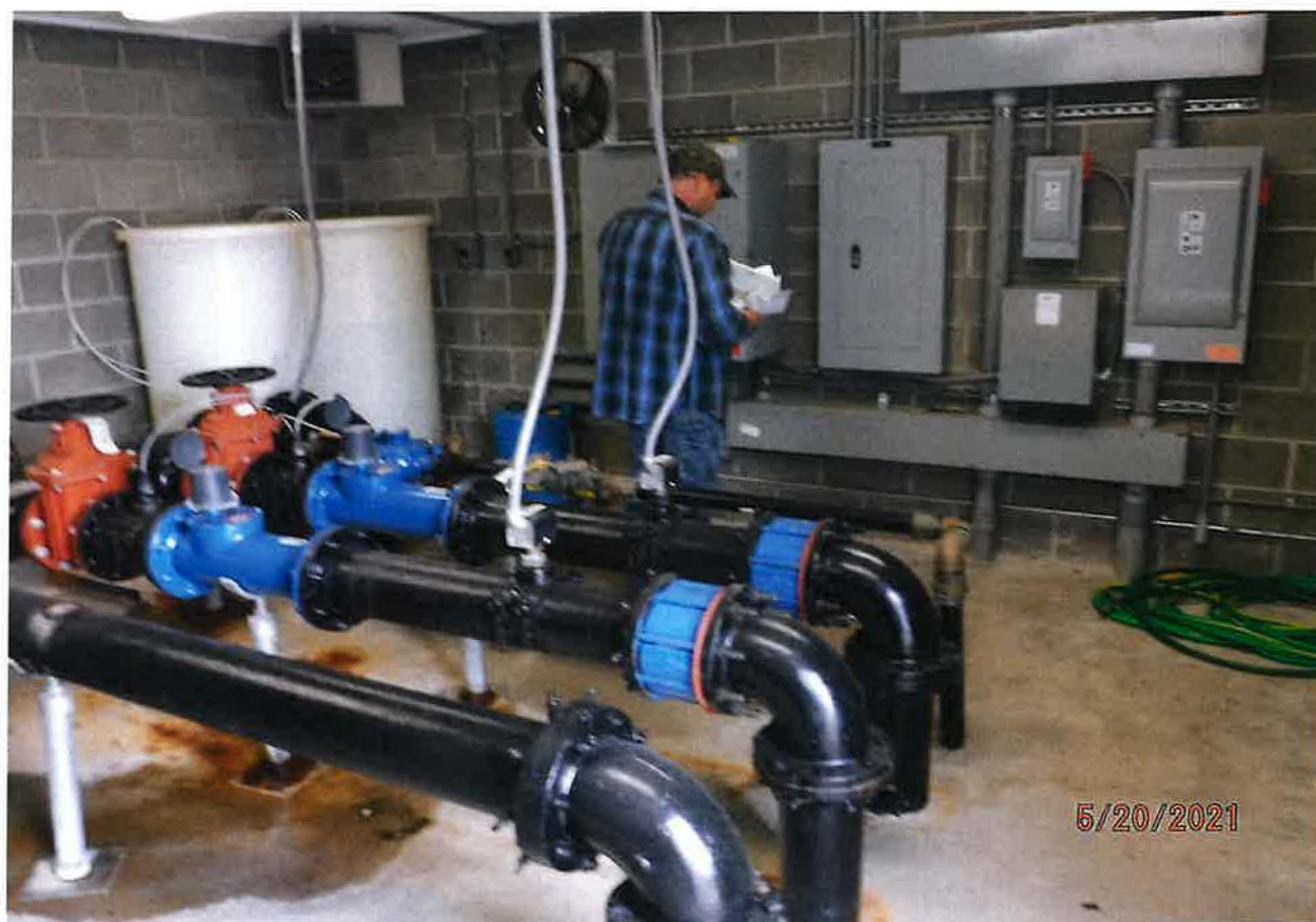
PUMP CONTROL PANELS IN BACKGROUND
