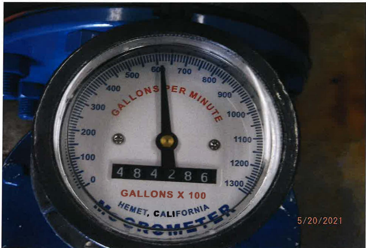
WELL #3 FLOW METER MEASURED 620 GPM
