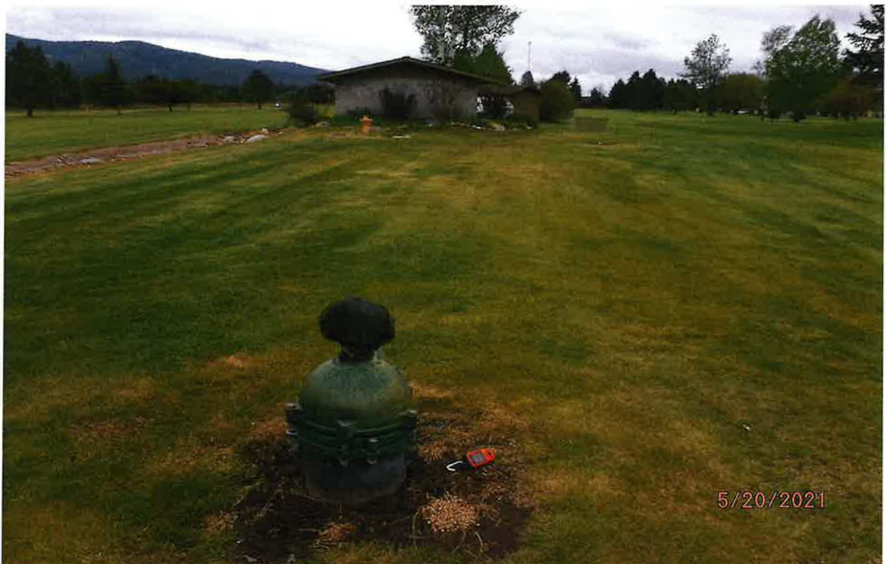
POD – GROUNDWATER WELL # 3; D0040131 (100 HP PUMP INSTALLED), PUMP STATION IN BACKGROUND
