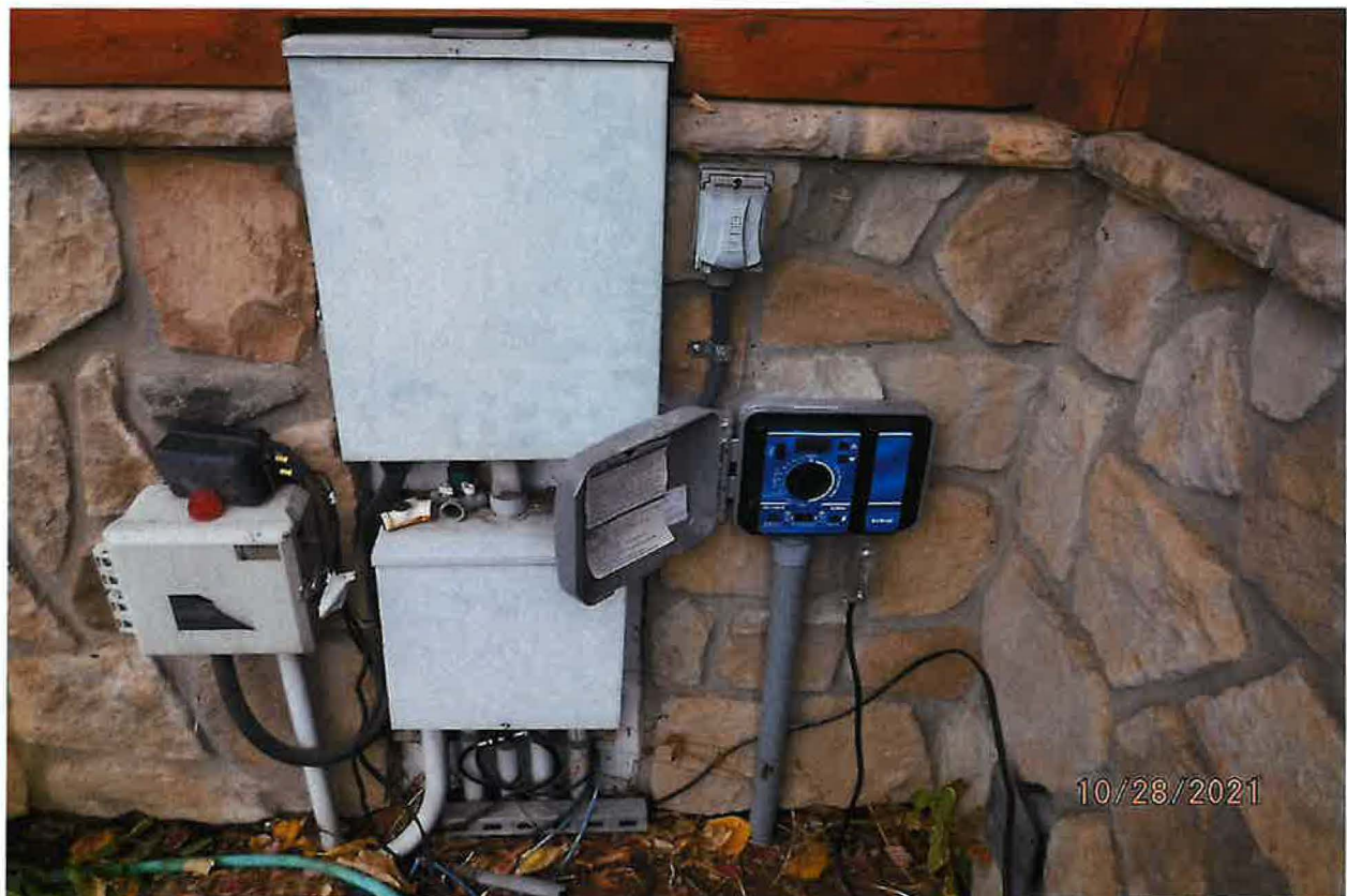
IRRIGATION SYSTEM CONTROL PANEL – SOUTHERN PORTION OF IRRIGATION POU
