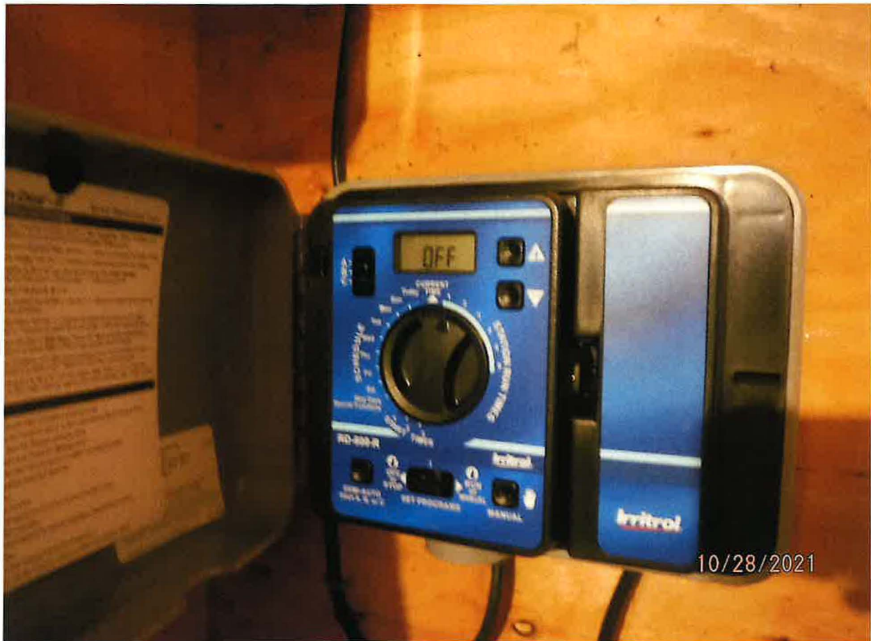
IRRIGATION SYSTEM CONTROL PANEL – NORTHERN PORTION OF IRRIGATION POU
