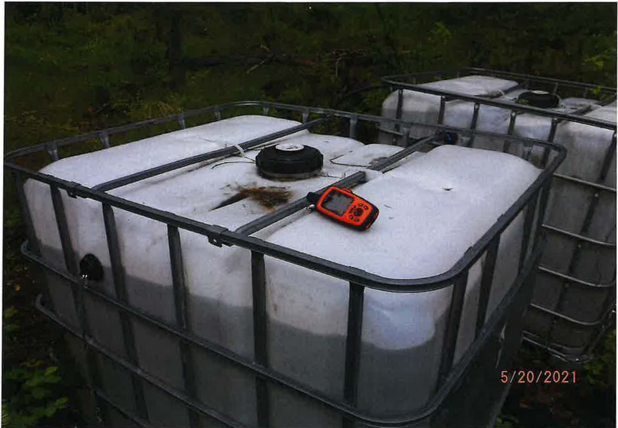
2 EA 275 GALLON STORAGE TANKS USED IN WATER SUPPLY SYSTEM
