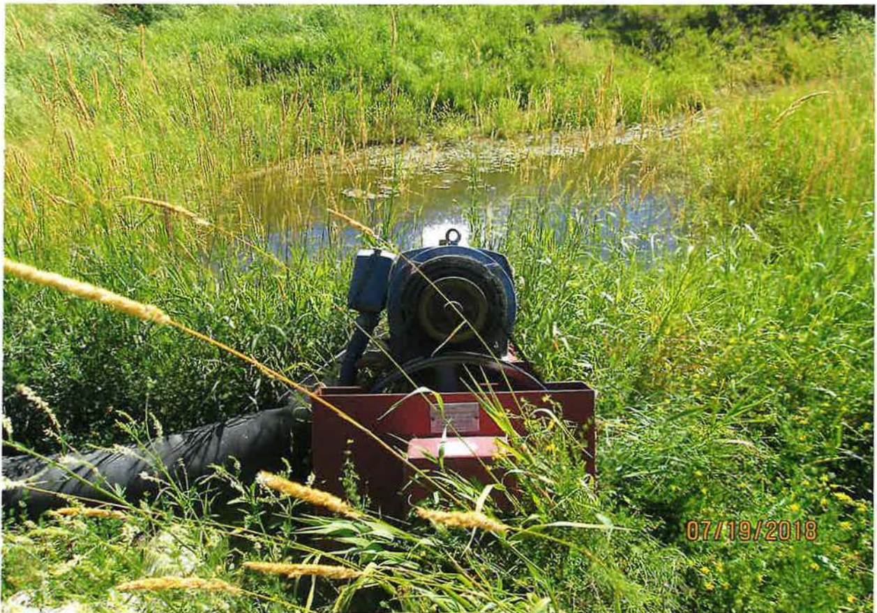
POD – PUMPING STATION 50 HP PUMP
