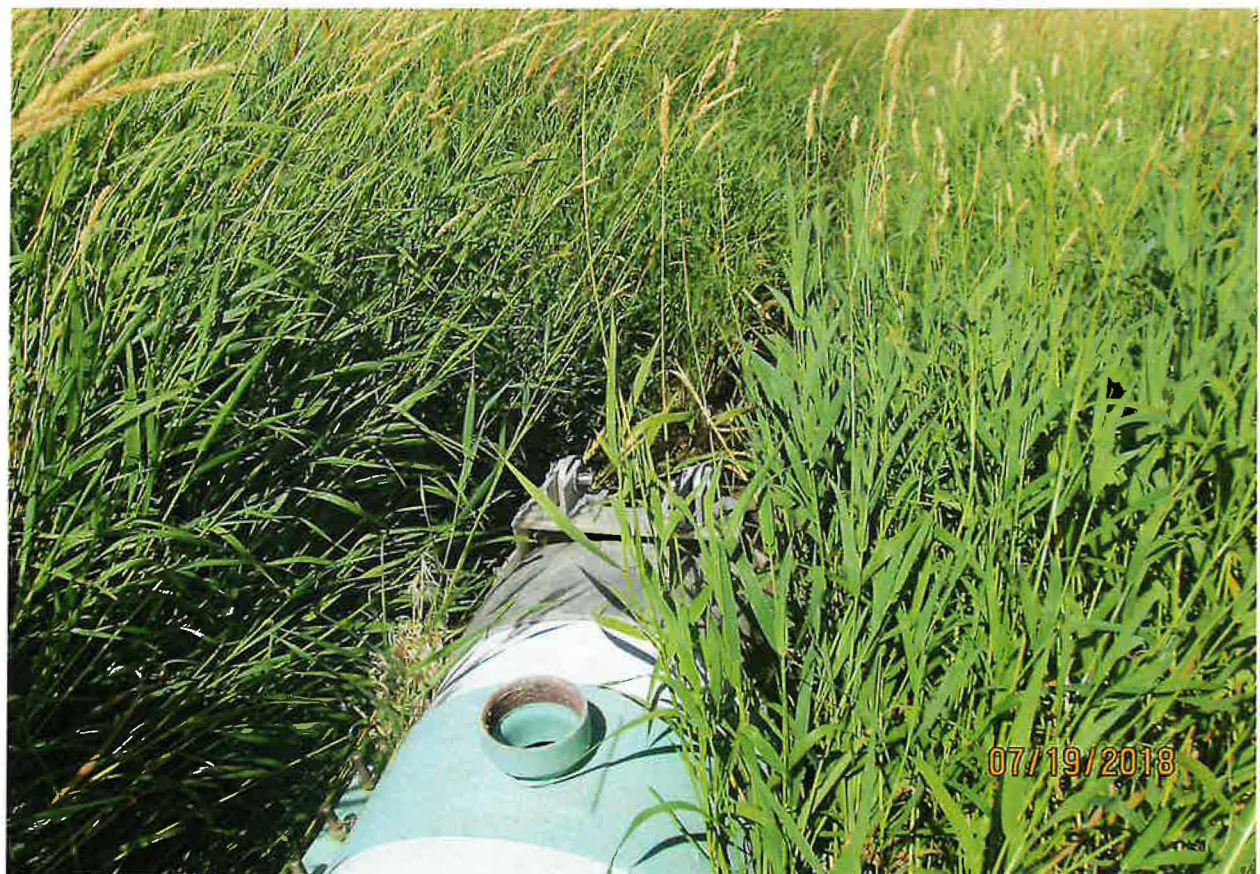
DISCHARGE PIPE TO WETLAND POU
