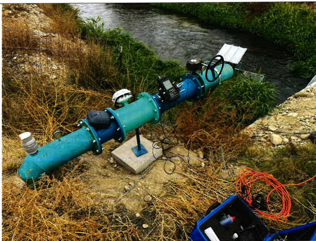
8" McCrometer DuraMag flow meter installed on system.
