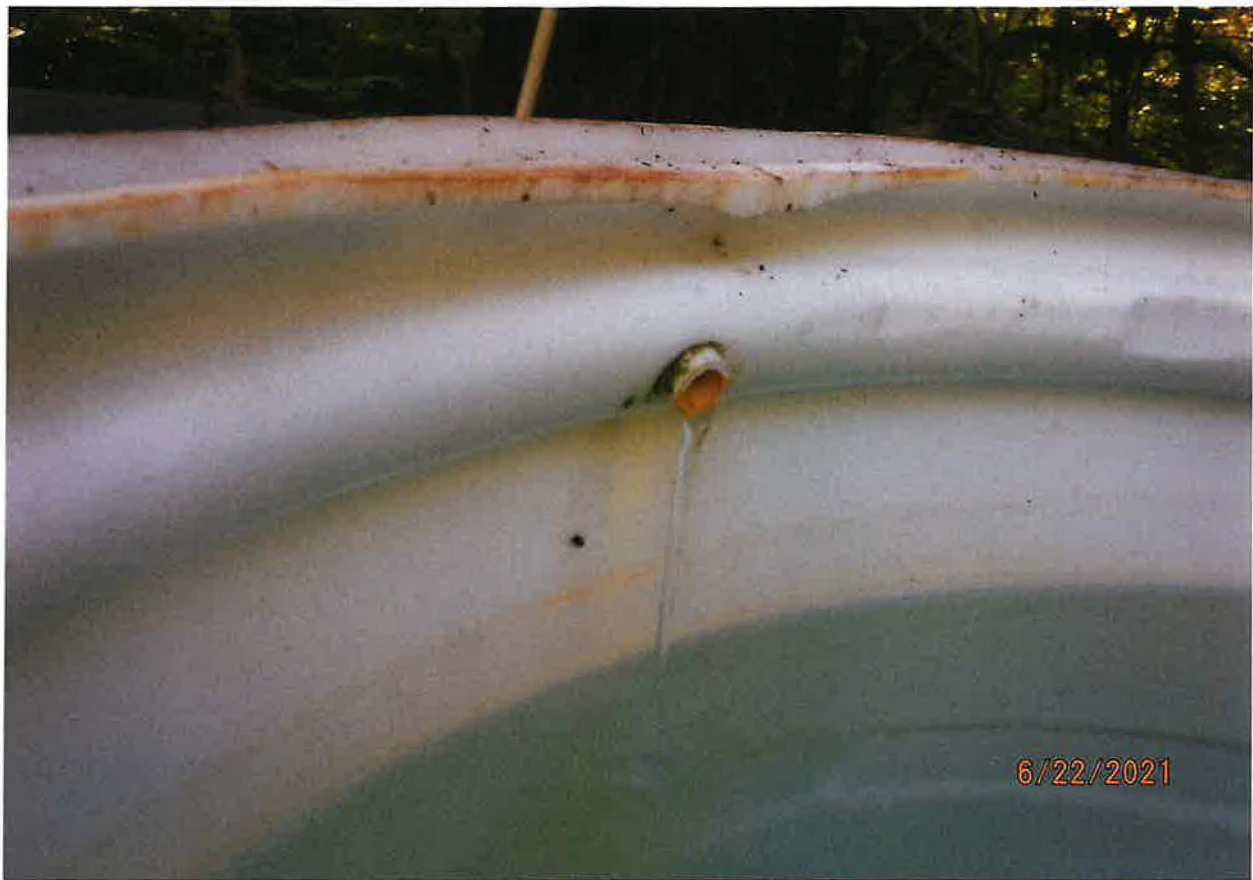
DIVERSION FROM SPRING SOURCE AT INTAKE TO STORAGE TANK – LOW FLOW SPRING
