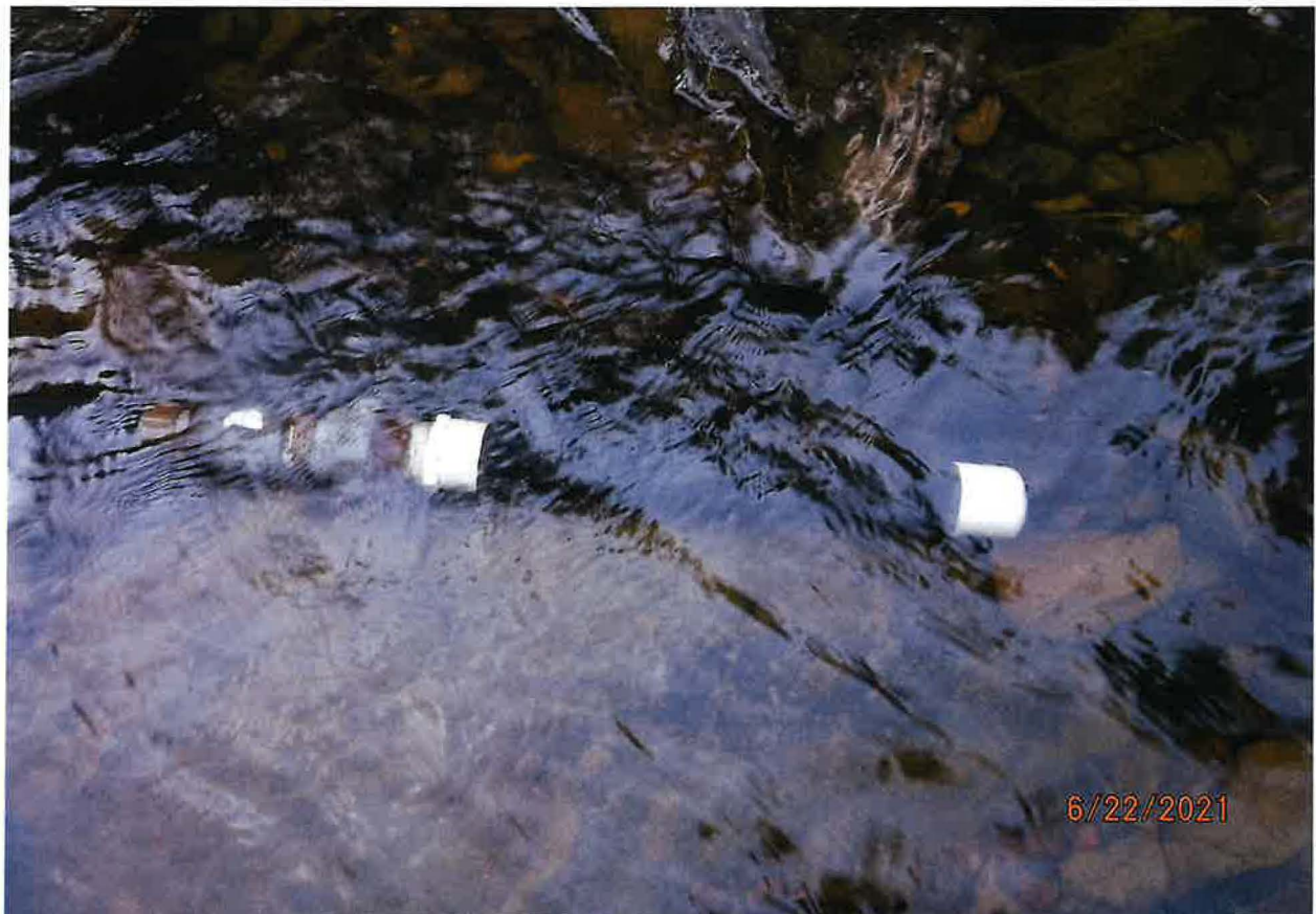
POD – CREEK DIVERSION WITH SCREENED INTAKE PIPE TO PUMP
