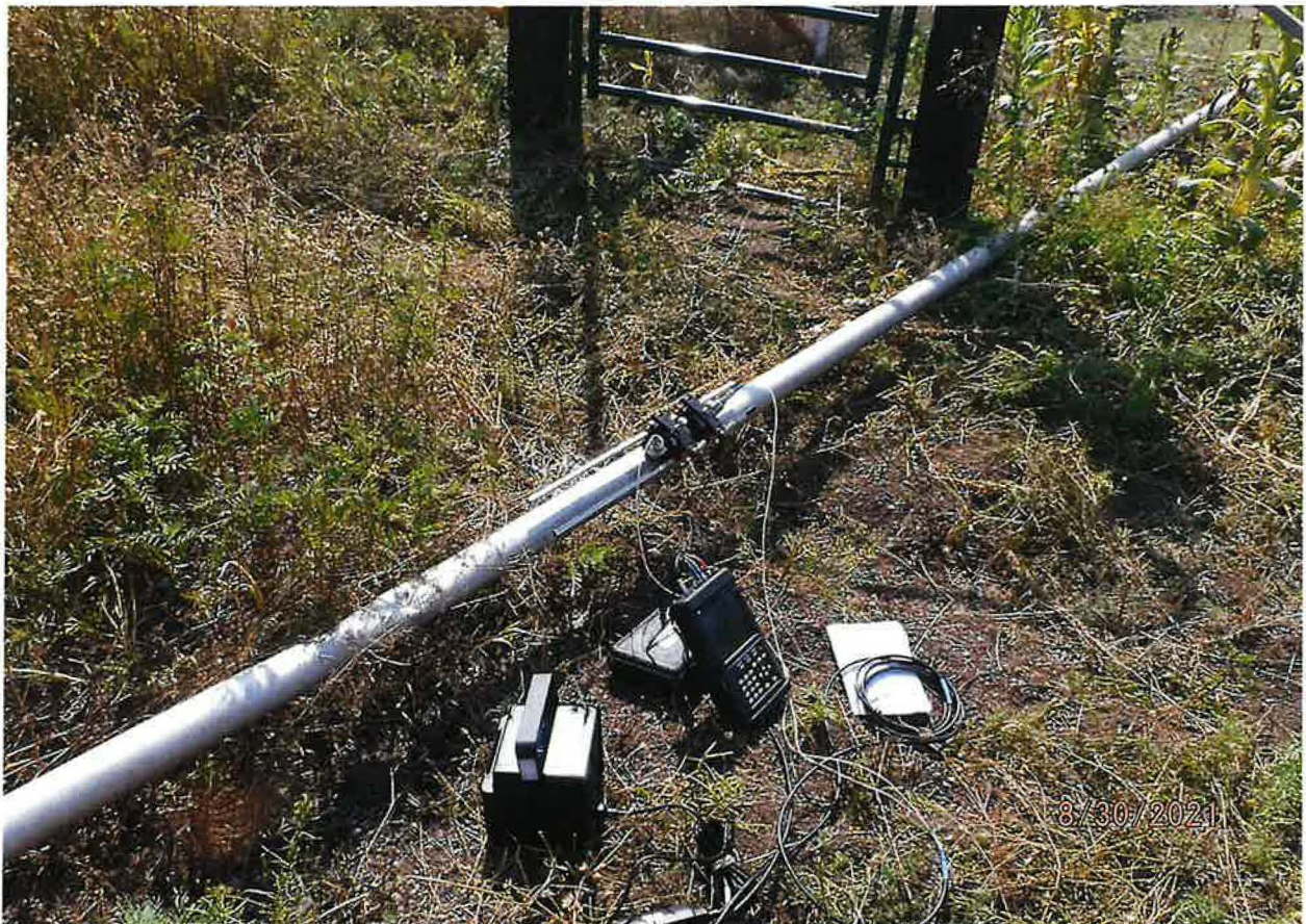
PANEMETRIC PT878 ULTRASONIC FLOWMETER INSTALLED NEAR POD FOR FLOW MEASUREMENTS
