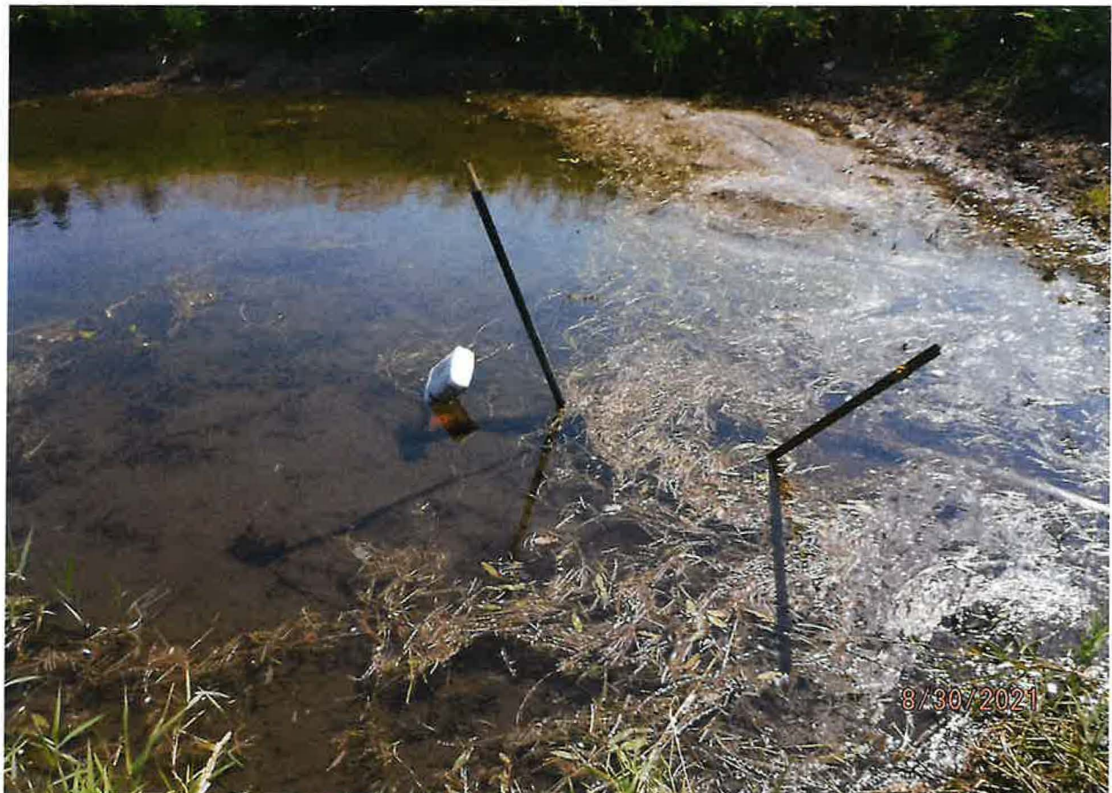
POD – SCREENED INTAKE PIPE IN LAKE
