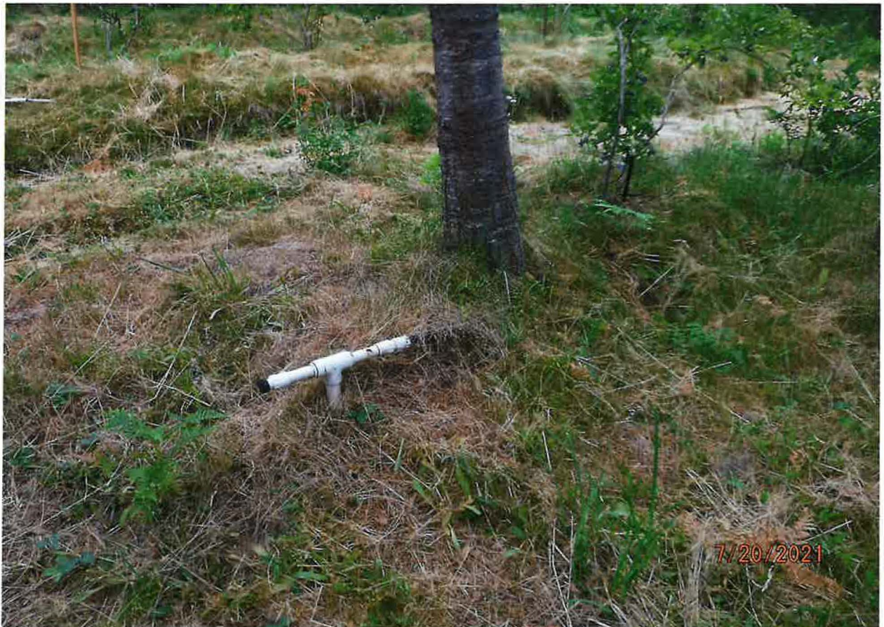
IRRIGATION POU – RISER PIPE TO SMALL EMITTER SPRINKLERS
