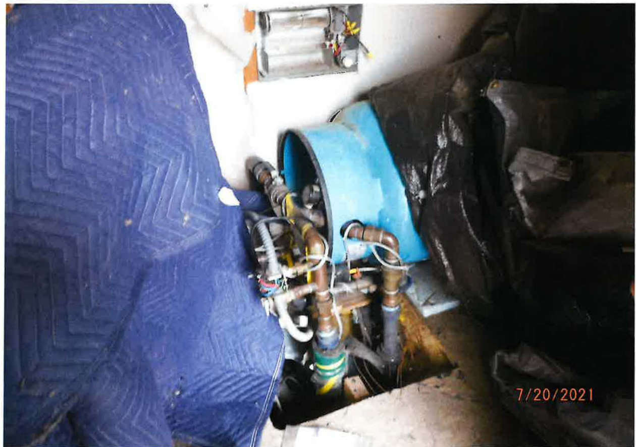
WELL PUMP WITH SMALL PRESSURE POT
