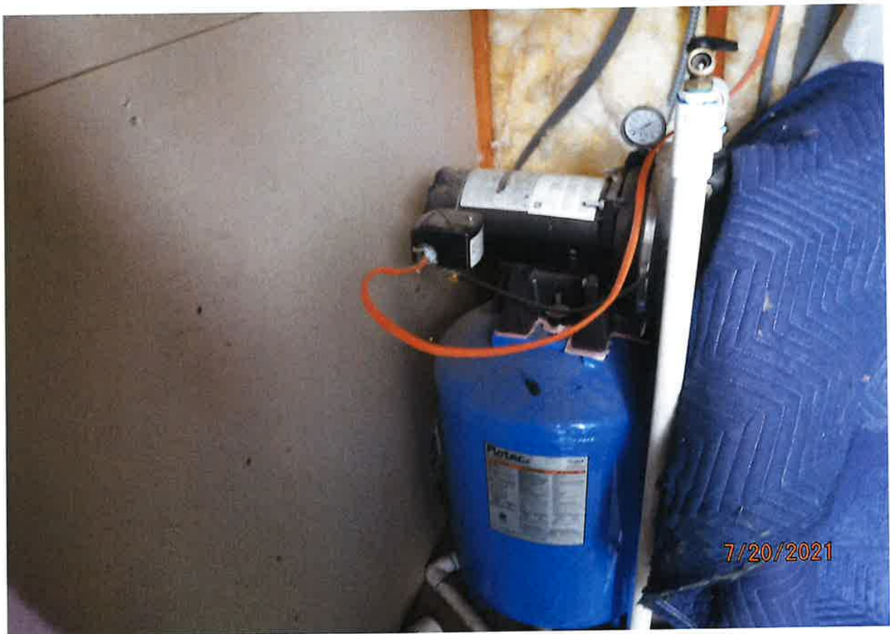
JET PUMP USED IN IRRIGATION SYSTEM FROM CREEK
