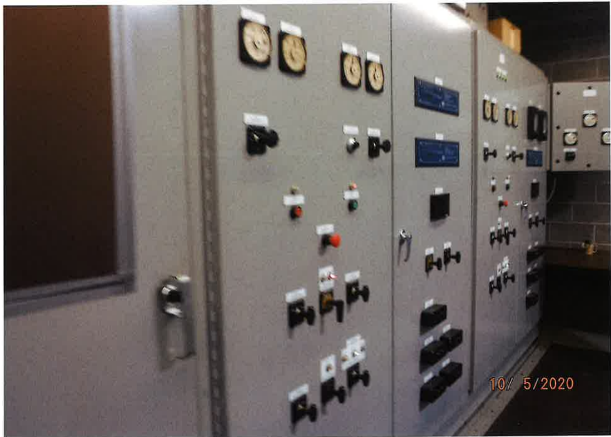
POWERHOUSE ELECTRIC CONTROL PANEL
