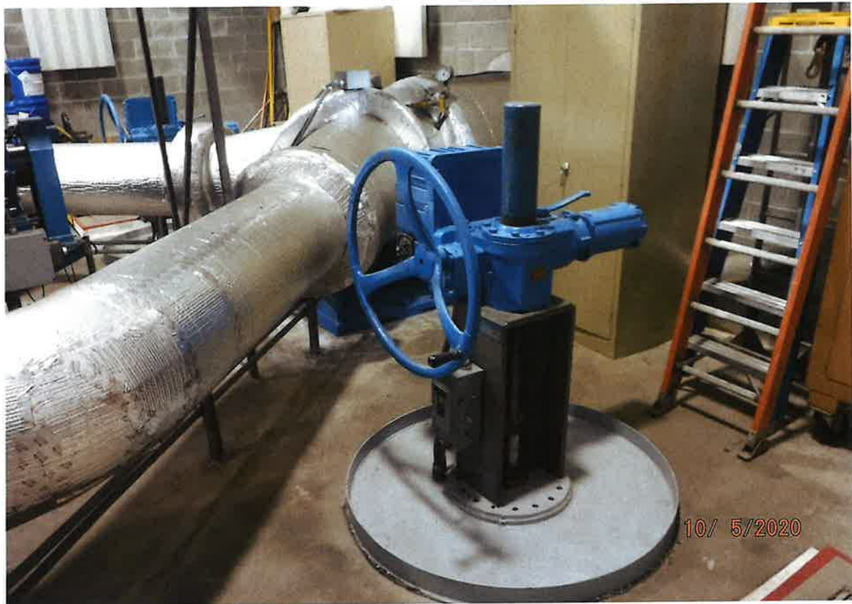
SECONDARY PIPE INTERIOR OF POWERHOUSE
