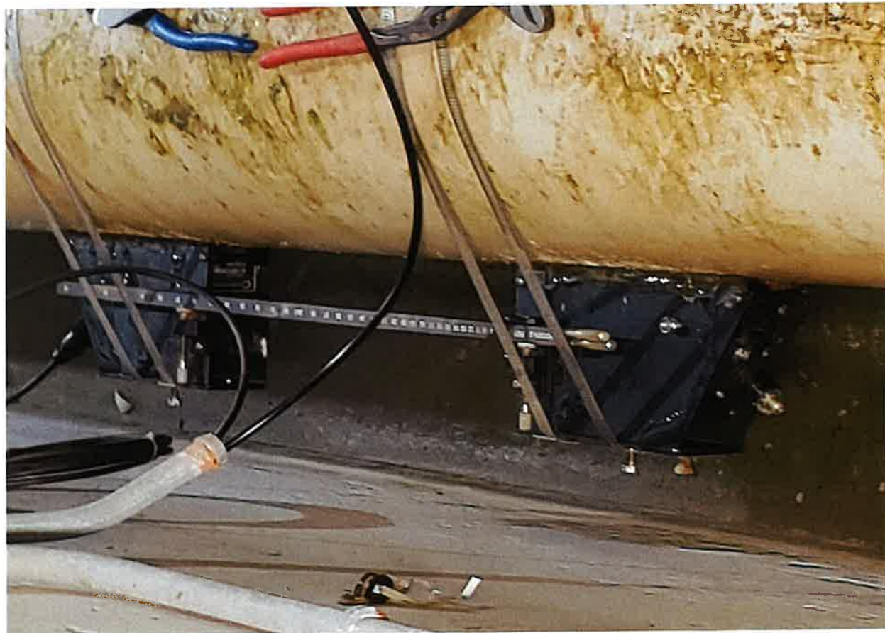
SECONDARY PIPE ULTRASONIC MEASURING DEVICE – INSIDE DAM PIPE ROOM
