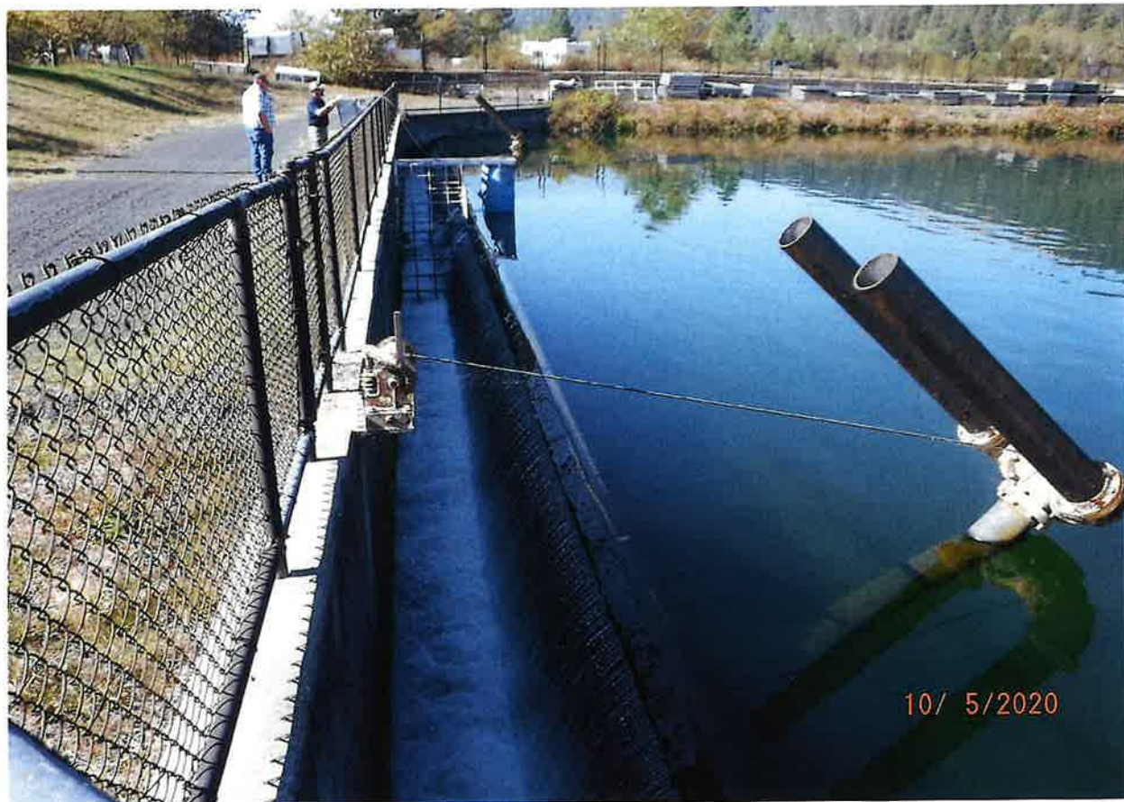
FISH PROPOGATION POU – METERED WEIR FROM SETTLING POND 2 OF 2 BEFORE DISCHARGE TO RIVER
