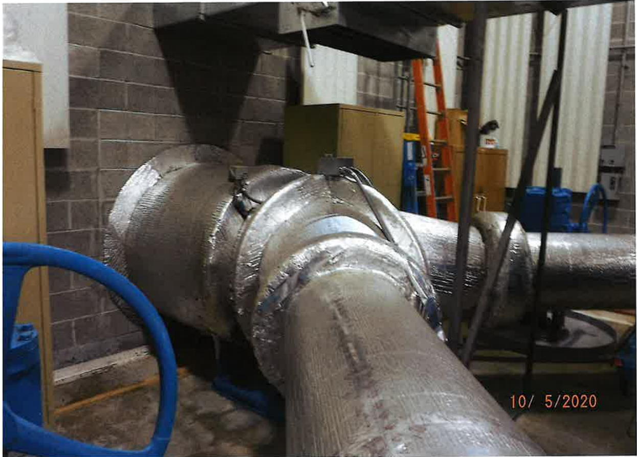
PRIMARY PIPE INTERIOR OF POWERHOUSE
