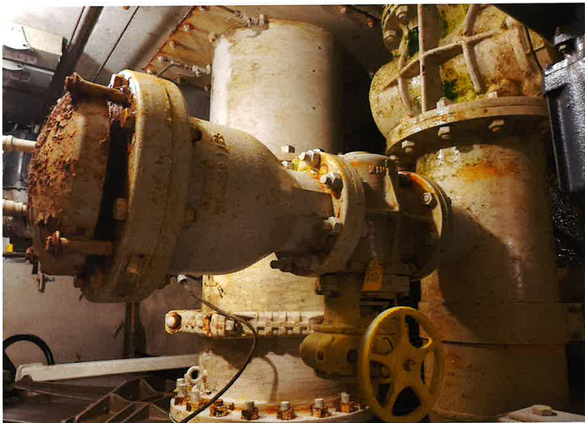
PRIMARY AND SECONDARY (FOREGROUND) PIPES – LOCATED INSIDE DAM PIPE ROOM
