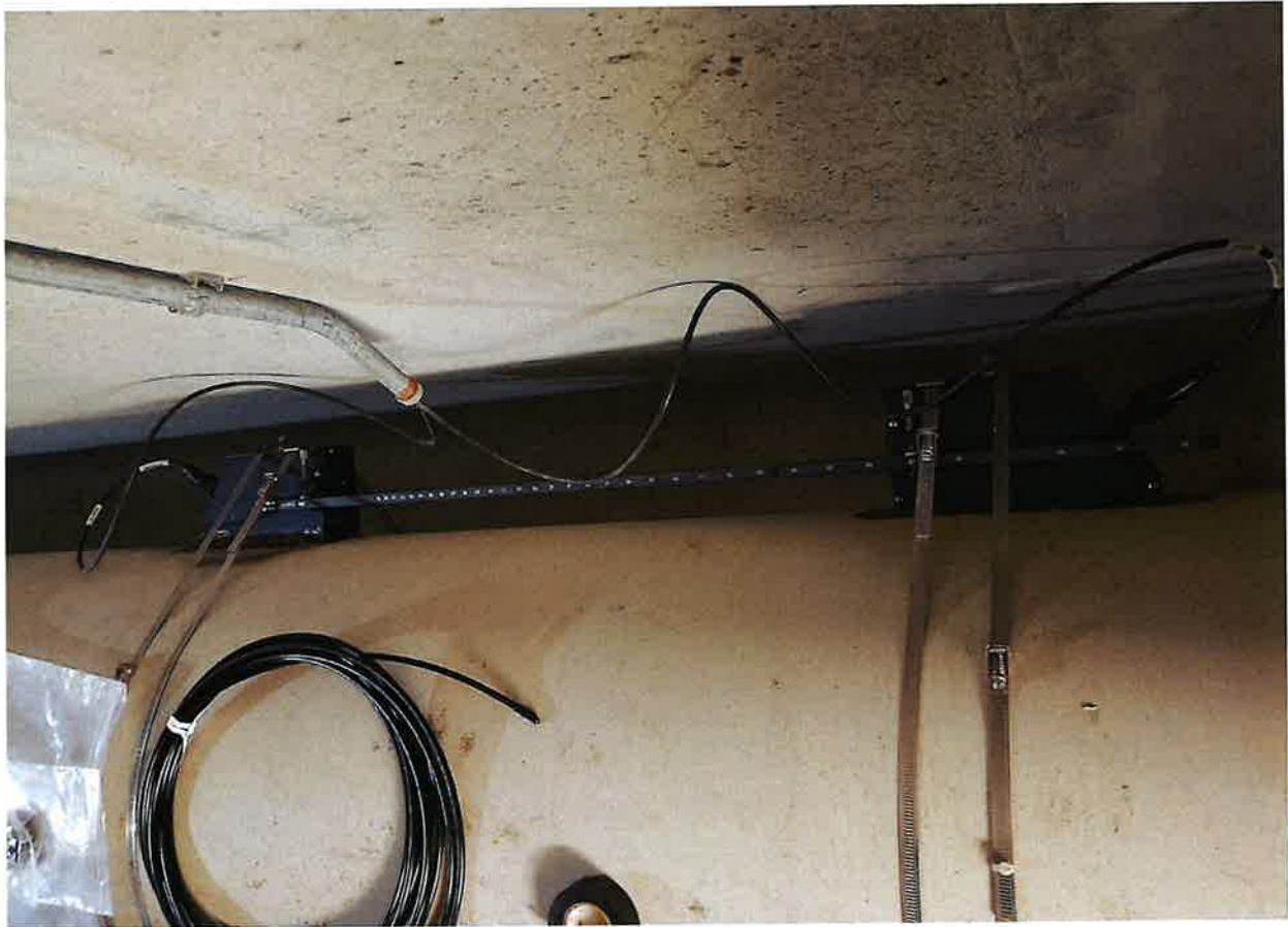
PRIMARY PIPE ULTRASONIC MEASURING DEVICE – INSIDE DAM PIPE ROOM
