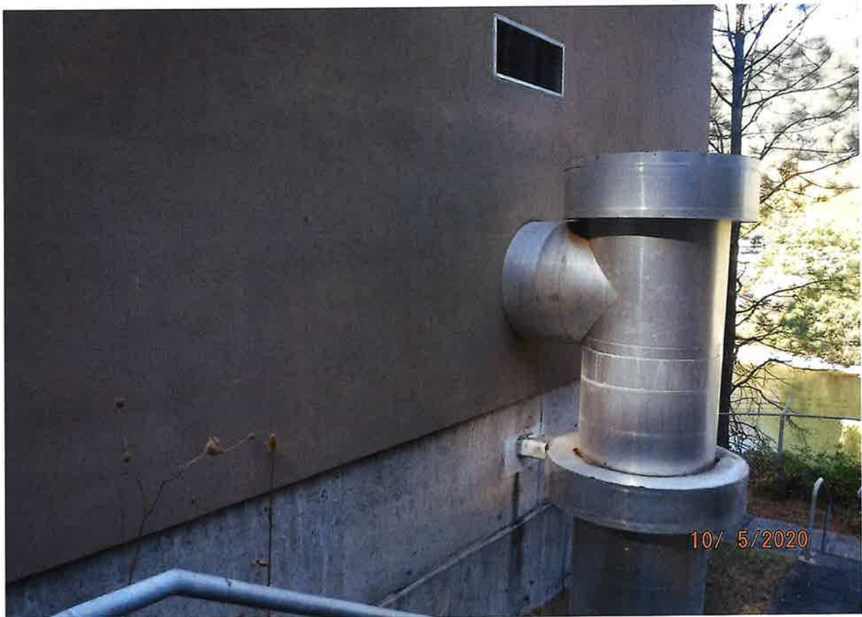
PRIMARY PIPE INTO POWERHOUSE
