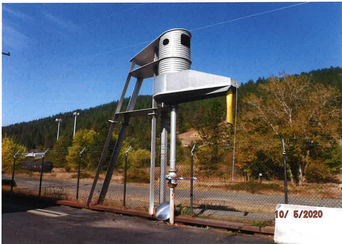
FISH PROPAGATION POU - TRUCK FILLING STATION
