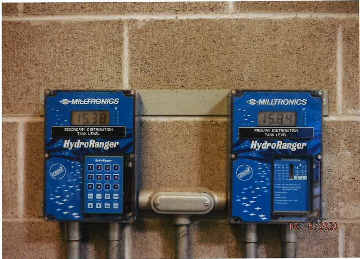
PRIMARY/SECONDARY TANK LEVEL PANELS
