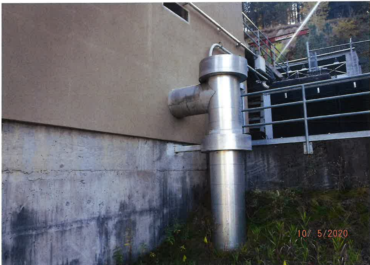
SECONDARY PIPE INTO POWERHOUSE
