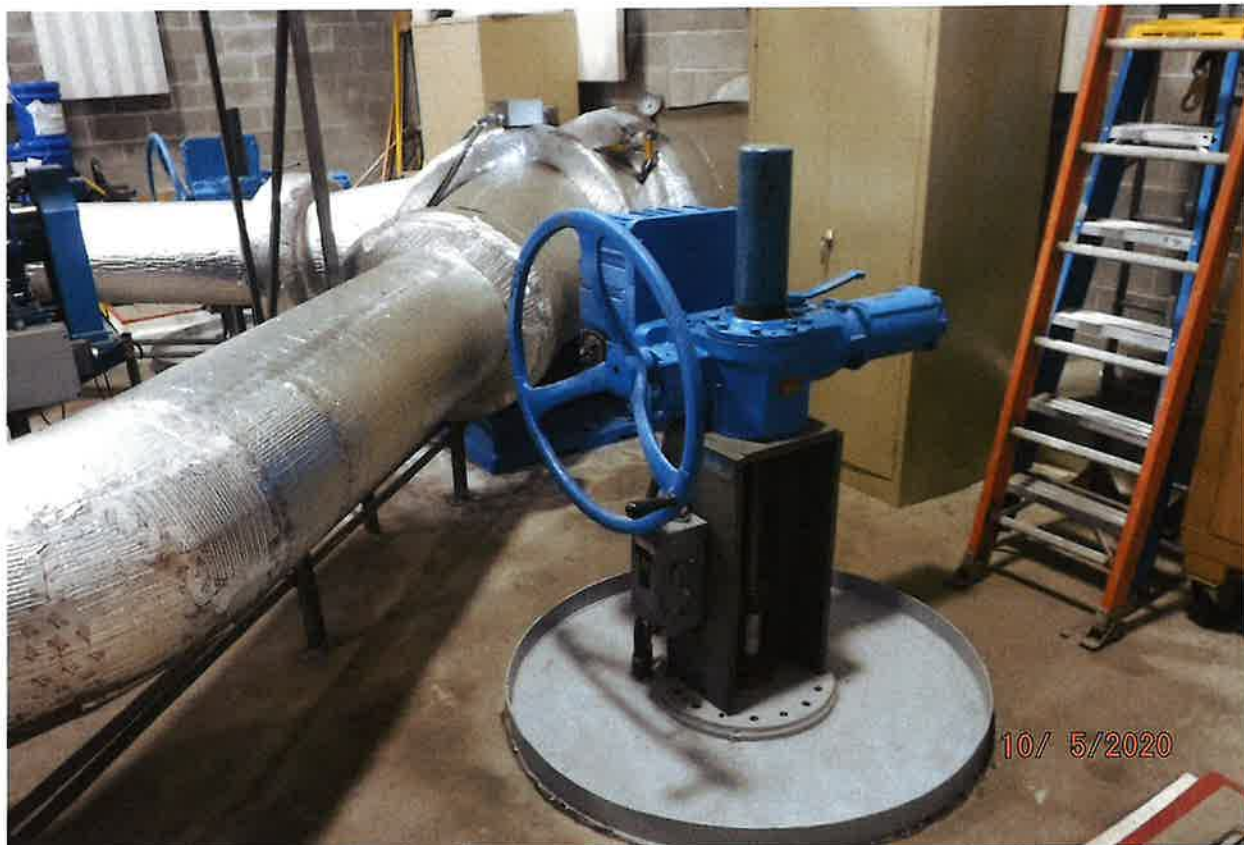
PRIMARY PAN SLEEVE VALVE FOR MANUAL OPERATION
