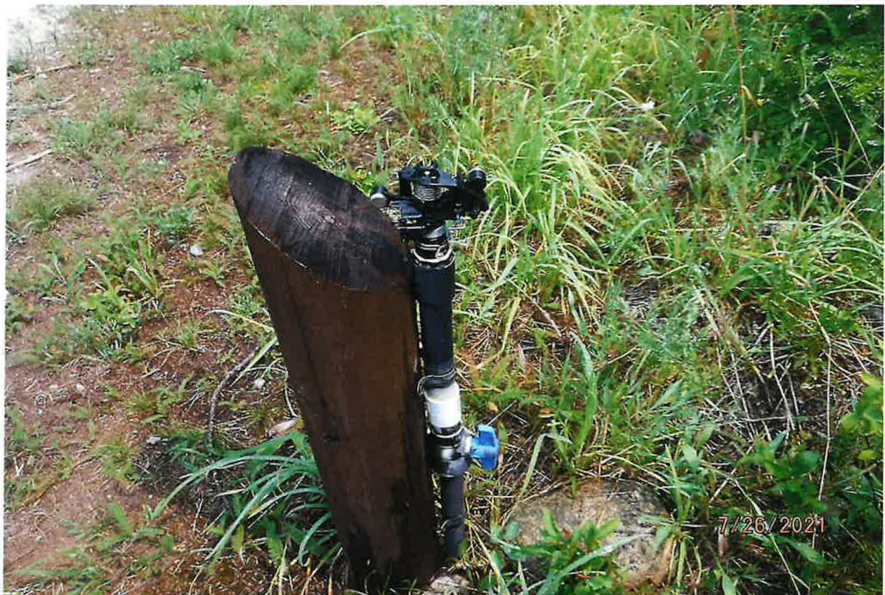
IRRIGATION POU – RISER PIPE TO SPRINKLER SET AT INTERVAL TO WATER LAWN & TREED LOT
