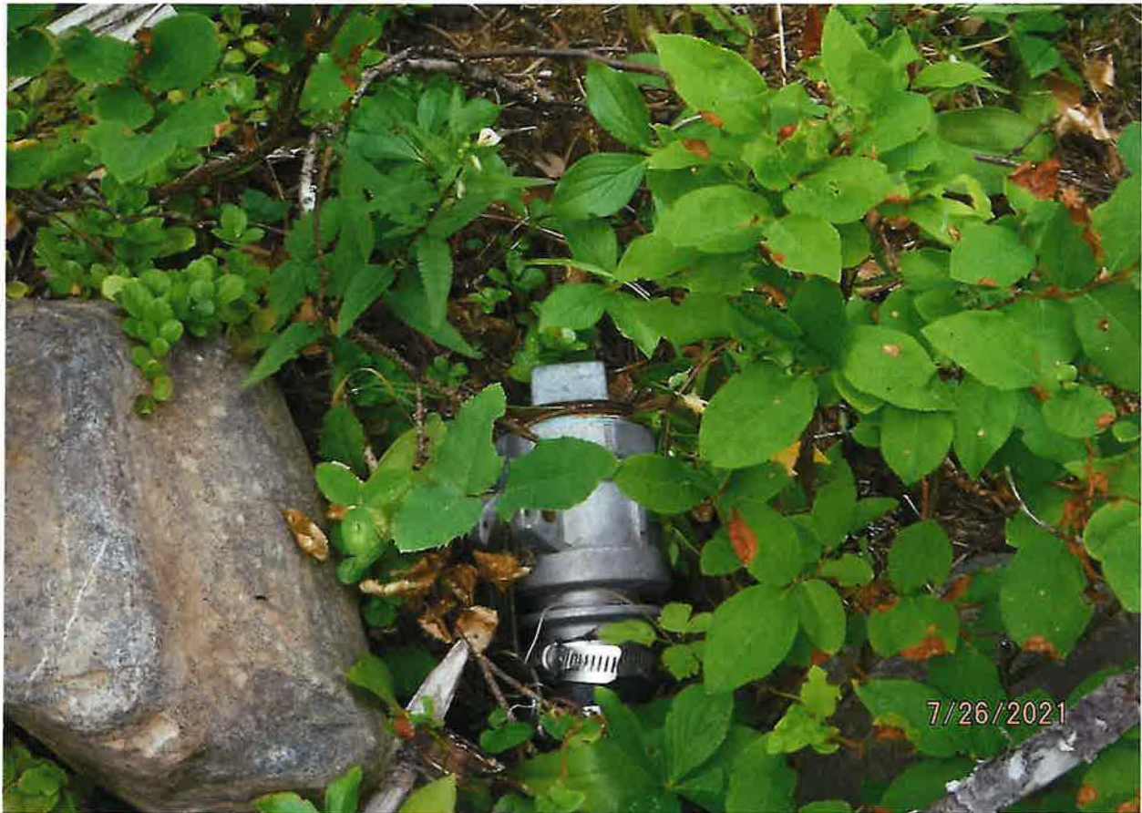
IRRIGATION SYSTEM BLOWOUT PORT
