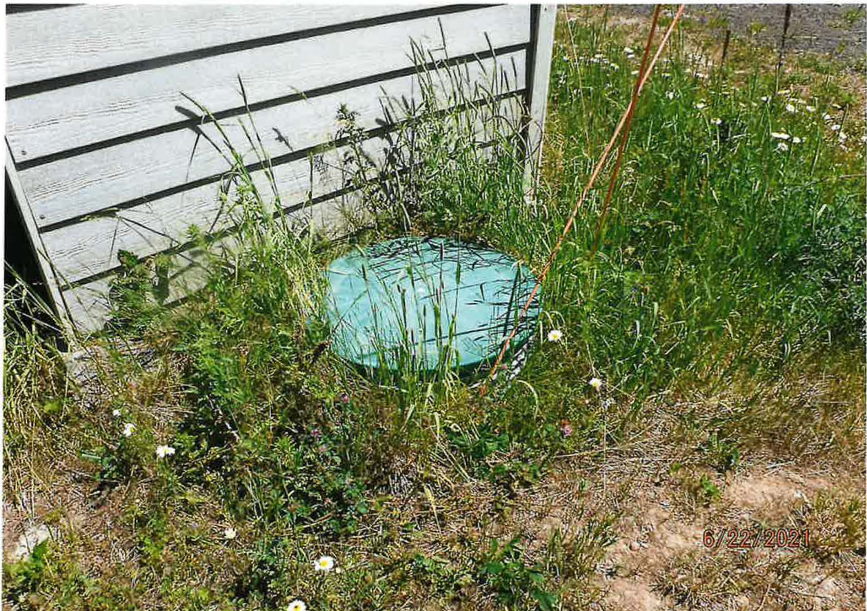
3,000 GALLON STORAGE TANK RECEIVES WATER DIRECT FROM WELL
