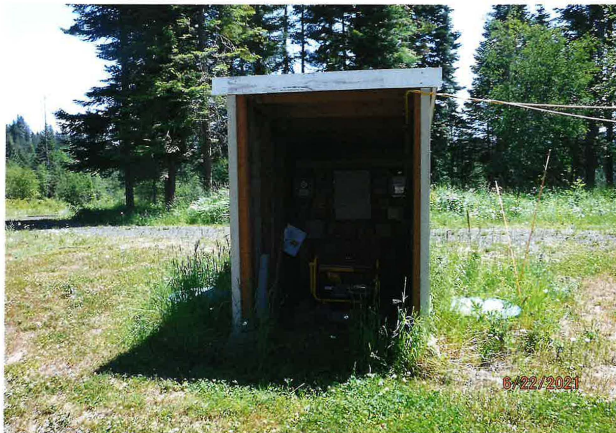
PUMP CONTROL PANEL
