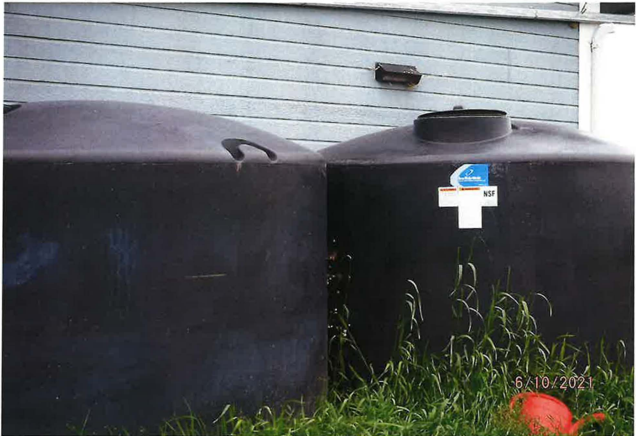
IRRIGATION FROM STORAGE 24HR IMPOUNDMENT TANKS
