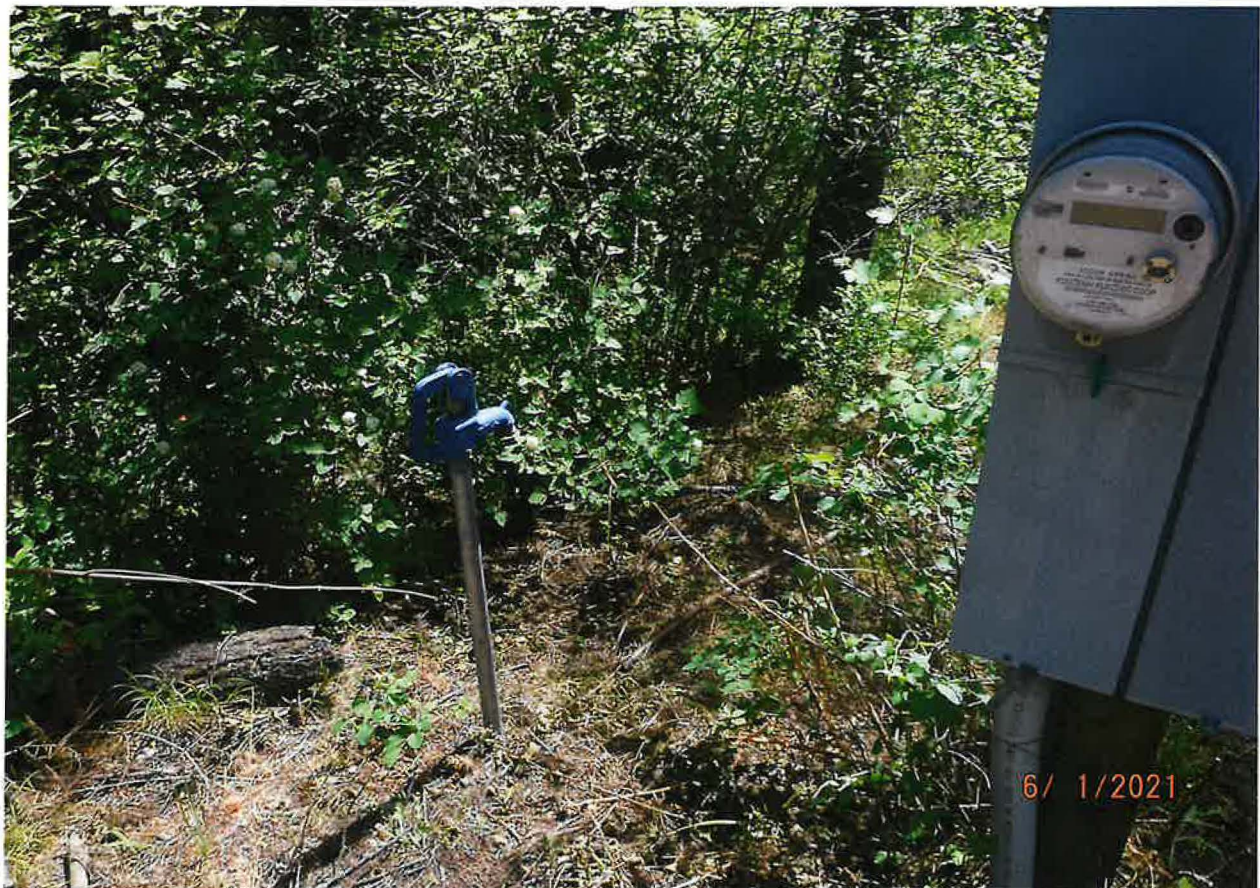
DOMESTIC POU – FROST FREE HYDRANT AND POWER BOX, STUB IN FOR LOT 14; LAKEWOOD ON HAYDEN SUBDIVISION – PARCEL No. 048200000140
