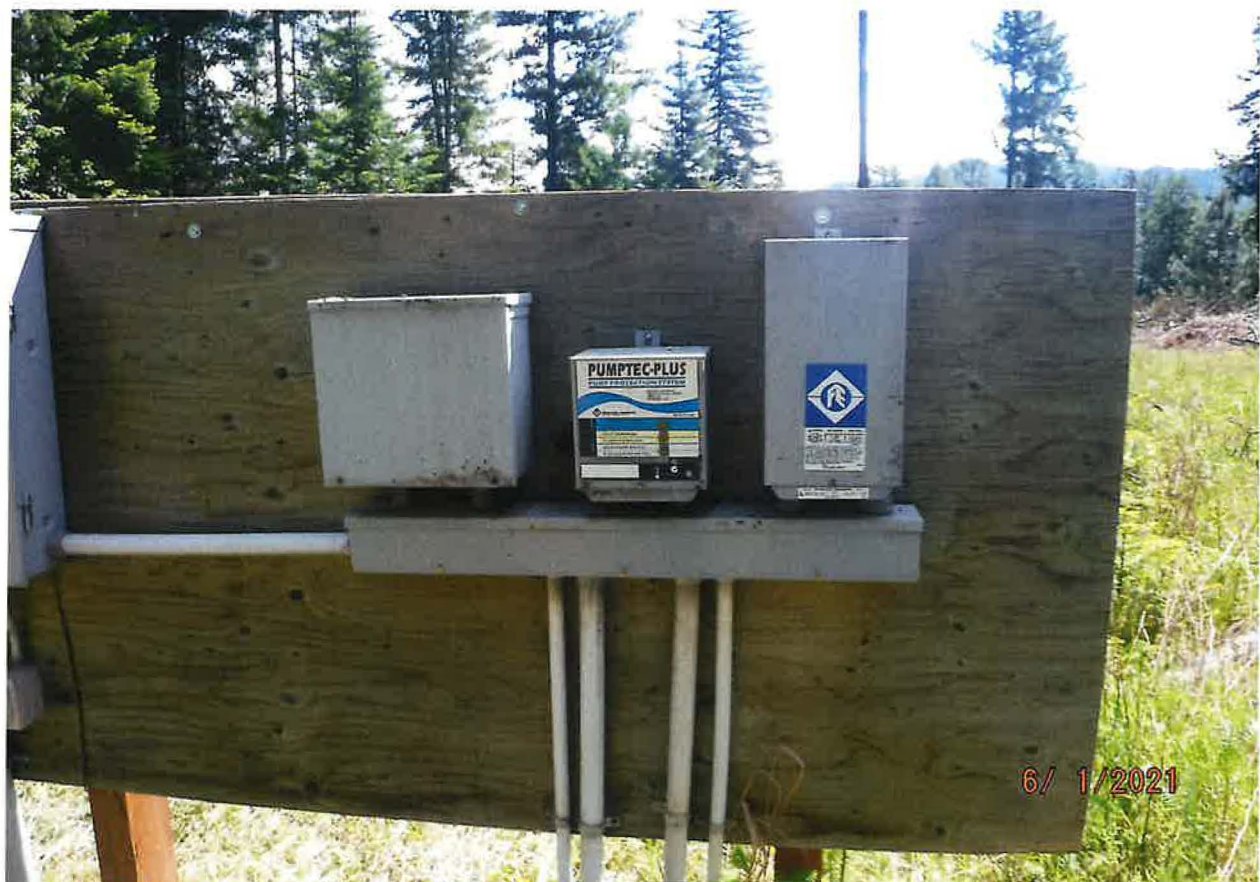
WELL PUMP CONTROL PANEL AND TRANSFER PUMP CONTROL PANEL
