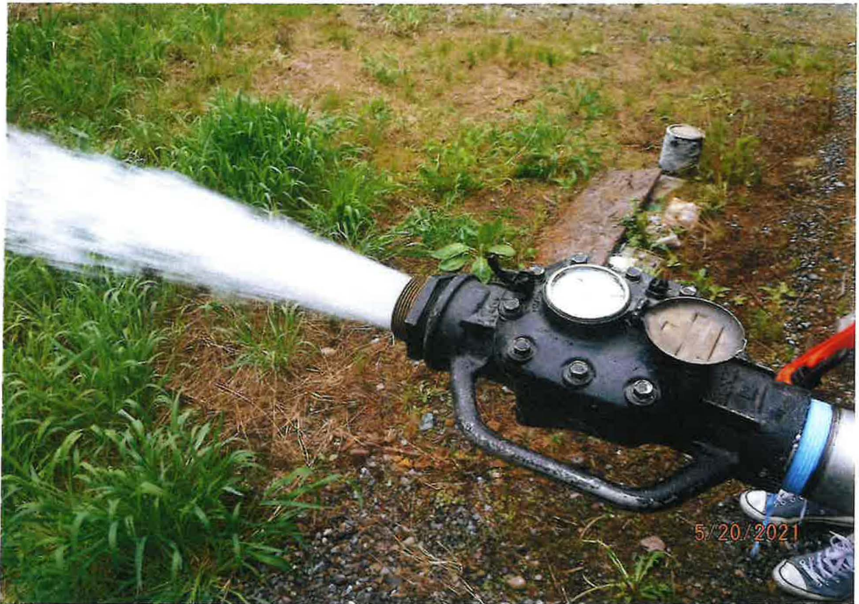
FLOW MEASUREMENT TAKEN AT SYSTEM BLOW-OUT VALVE
