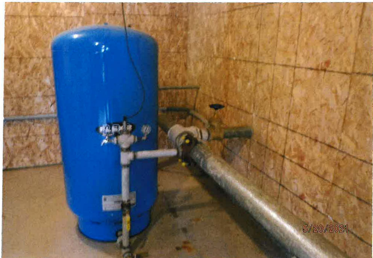
DIVERTING WORKS – 65 GALLON PRESSURE TANK WITH MAIN LINE
