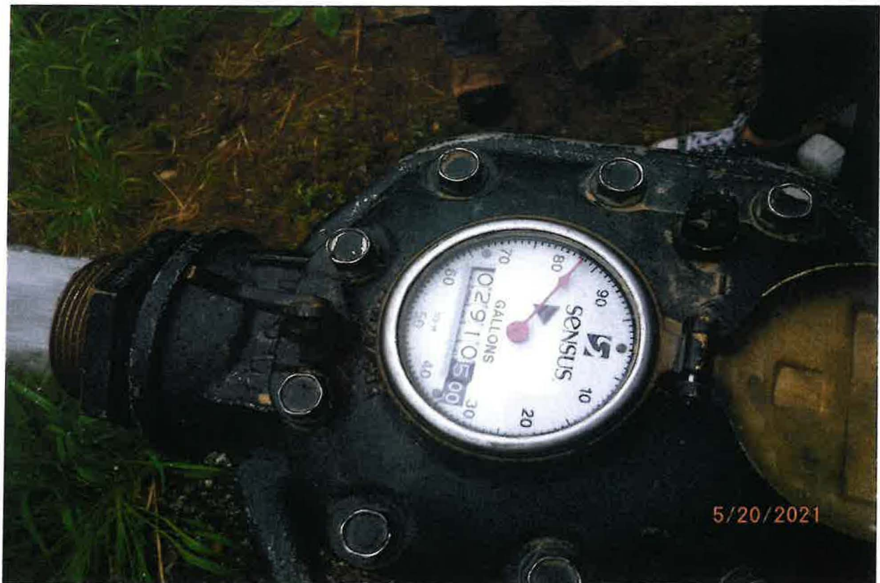
FLOWMETER USED FOR FLOWMEASUREMENT—SYSTEM FLOW STABILIZED AT 90 GPM (NOT REPRESENTED IN THIS PHOTOGRAPH)
