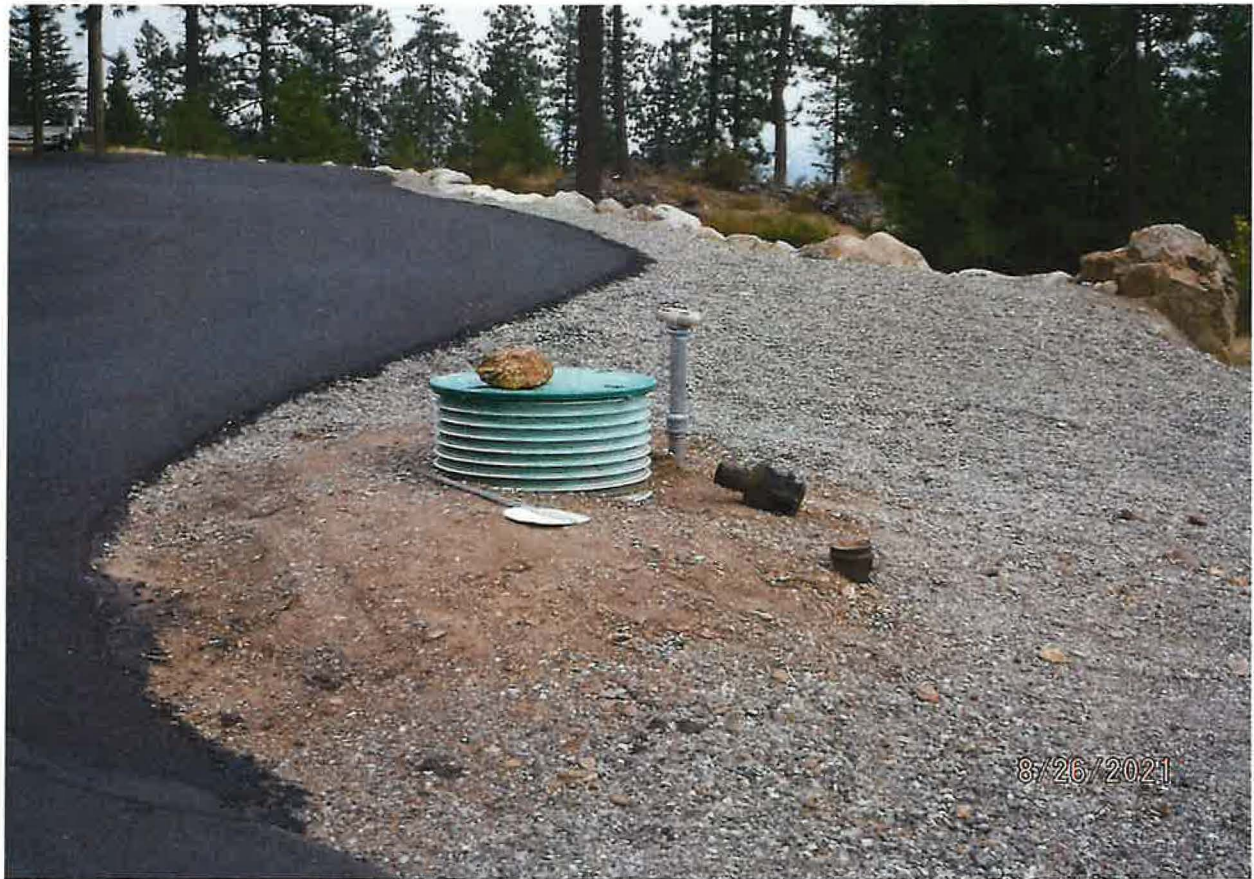
WATER SYSTEM INCORPORATES A 1,500 GAL STORAGE TANK FOR EACH LOT – 9 TOTAL
