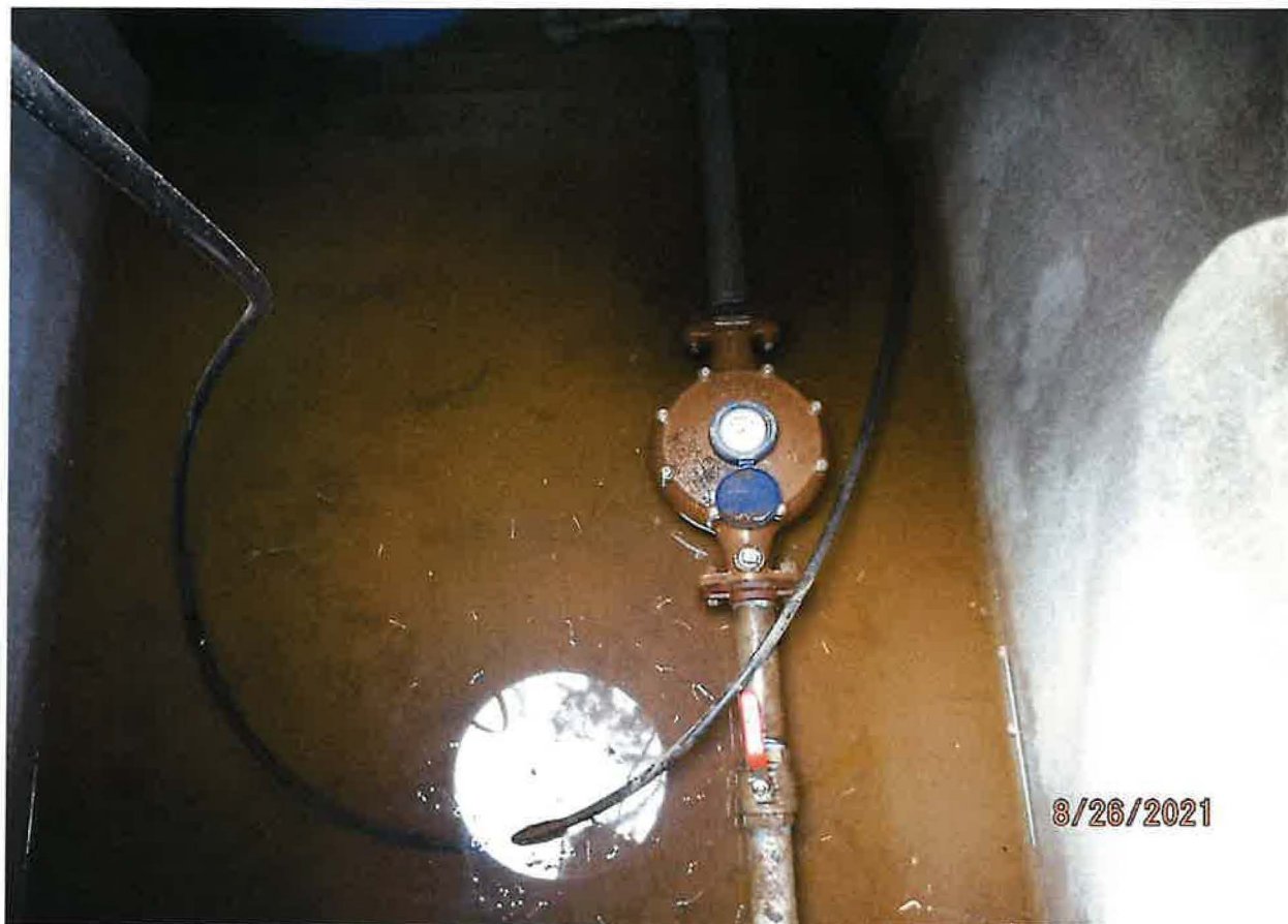
WELL D0084679 DIVERTING WORKS, INCLUDES PRESSURE TANK AND FLOWMETER
