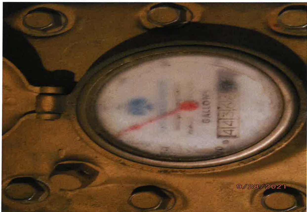
ROCKWELL INTERNATIONAL FLOW METER INSTALLED ON WELL MAIN WATER LINE
