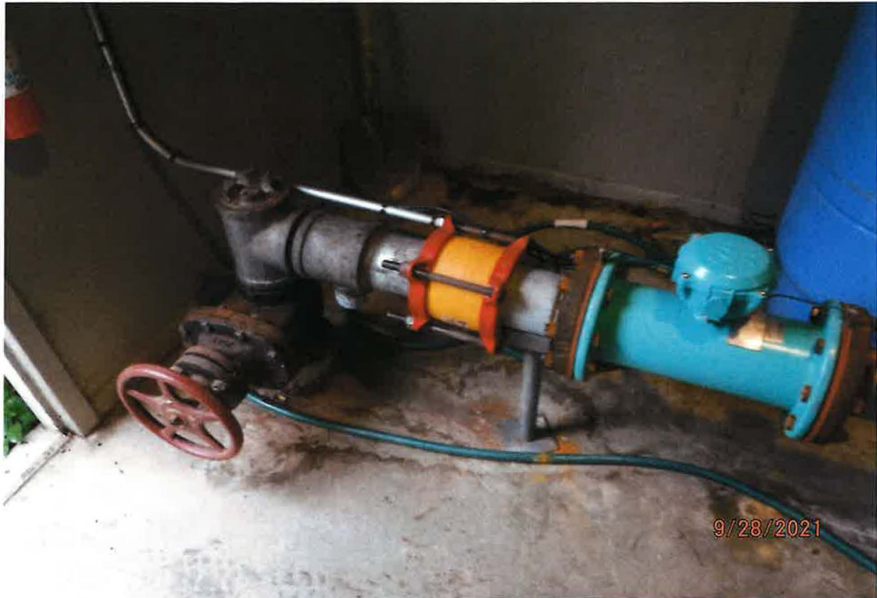
FROM STORAGE TANK WATER SYSTEM PIPES
