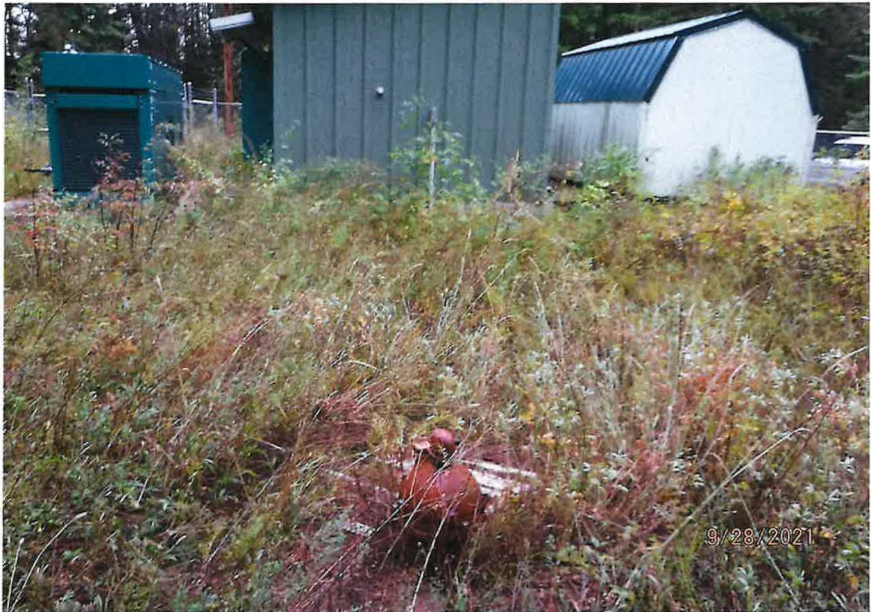
POD – WELL 95-81-N-74 WITH 30 HP PUMP INSTALLED
